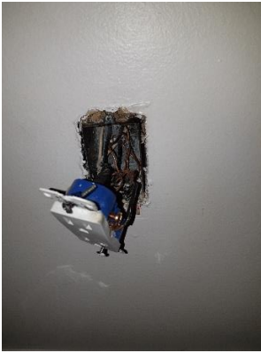
Receptacle and outlet box at scene of incident
