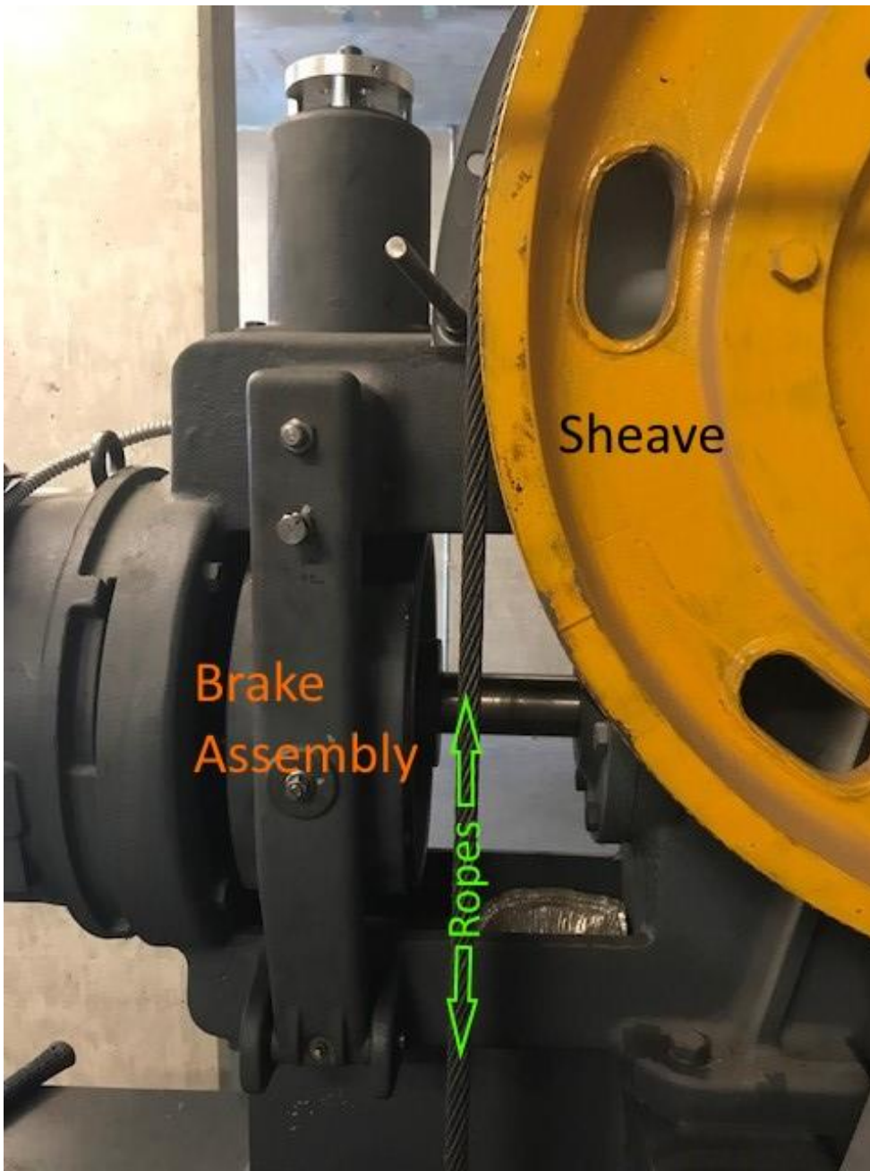
Components involved in the incident.
