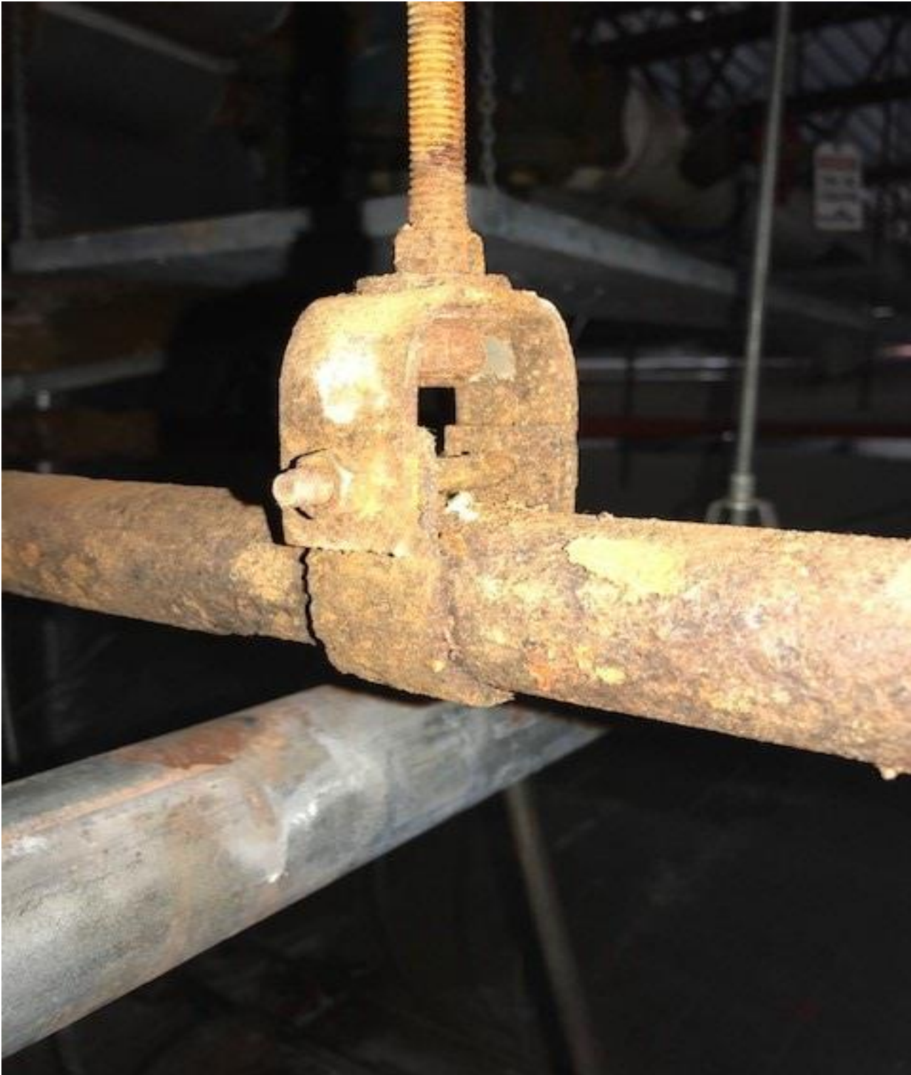
Picture 2 Corroded pipe, pipe hanger and metal thinning
