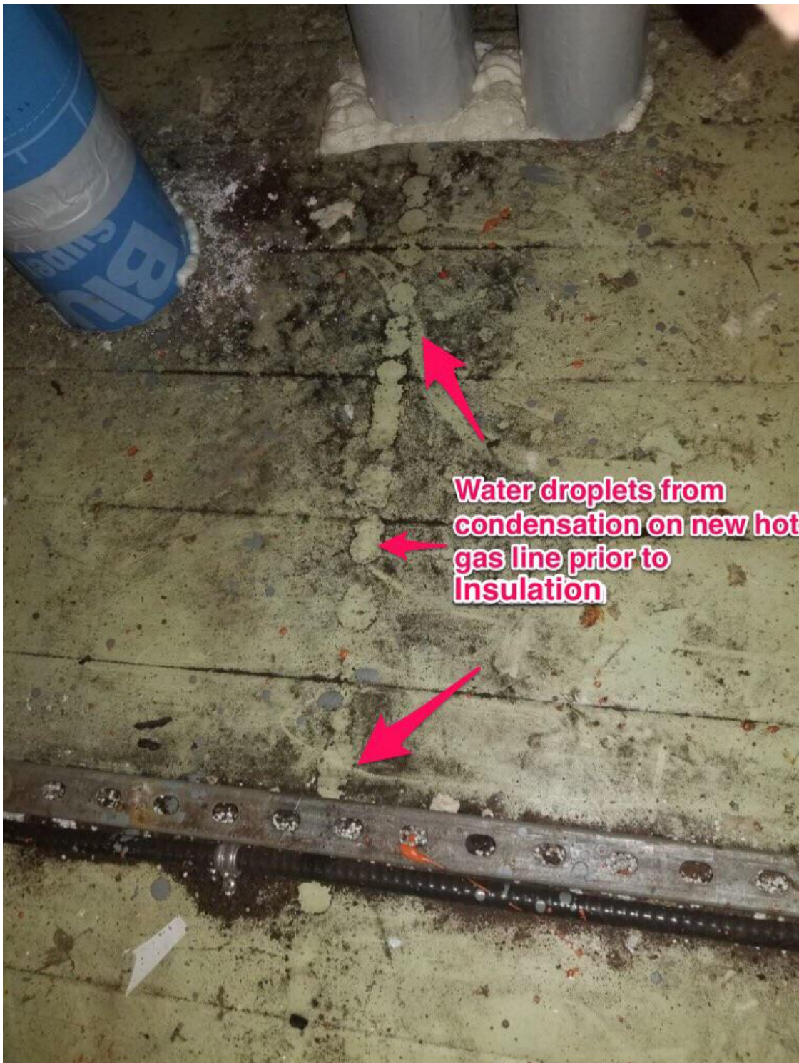
Picture 5 Mezzanine floor under newly installed hot gas pipe prior to new vapor type insulation being applied.
