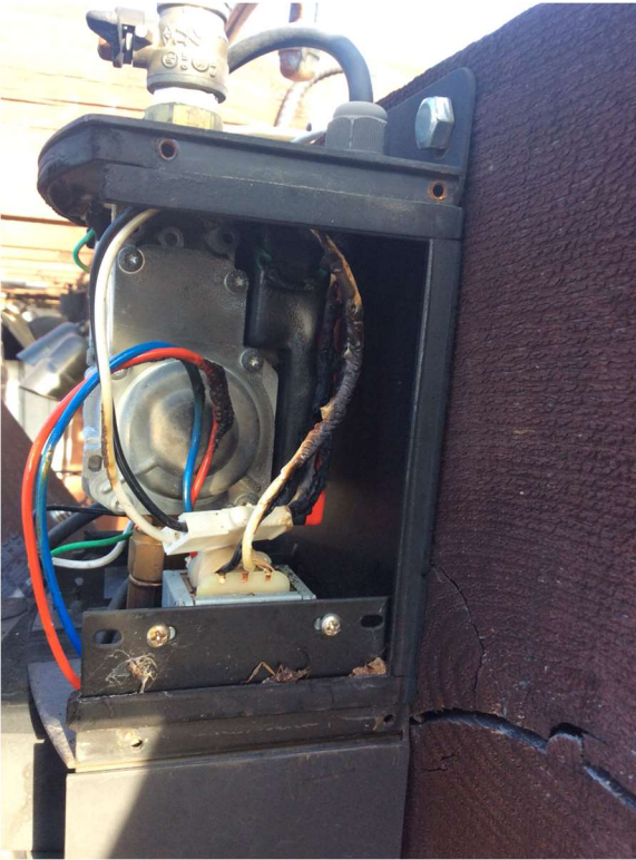
Burnt wiring by gas valve
