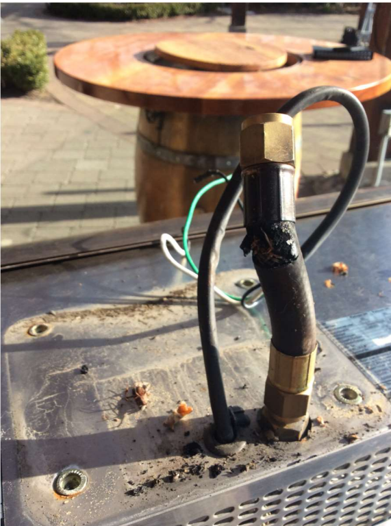
Gas hose connected to burner
