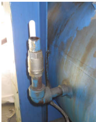
Figure 1: The 1" valve on the P34 HPR that was the source of the release
