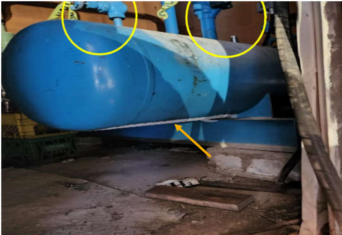
Figure 12: P24 receiver frost line after purging
