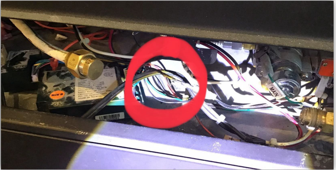
Image – Damaged conductors below fireplace.
