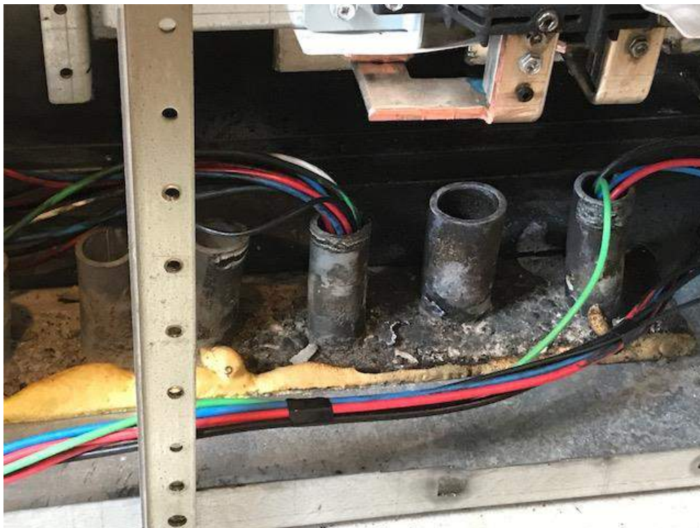
Initial burn damage within enclosure
