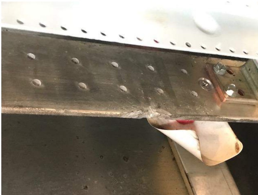
Extent of Buss damage- at load end of enclosure
