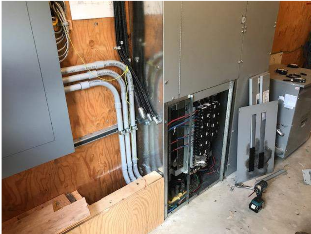
MDC after incident
