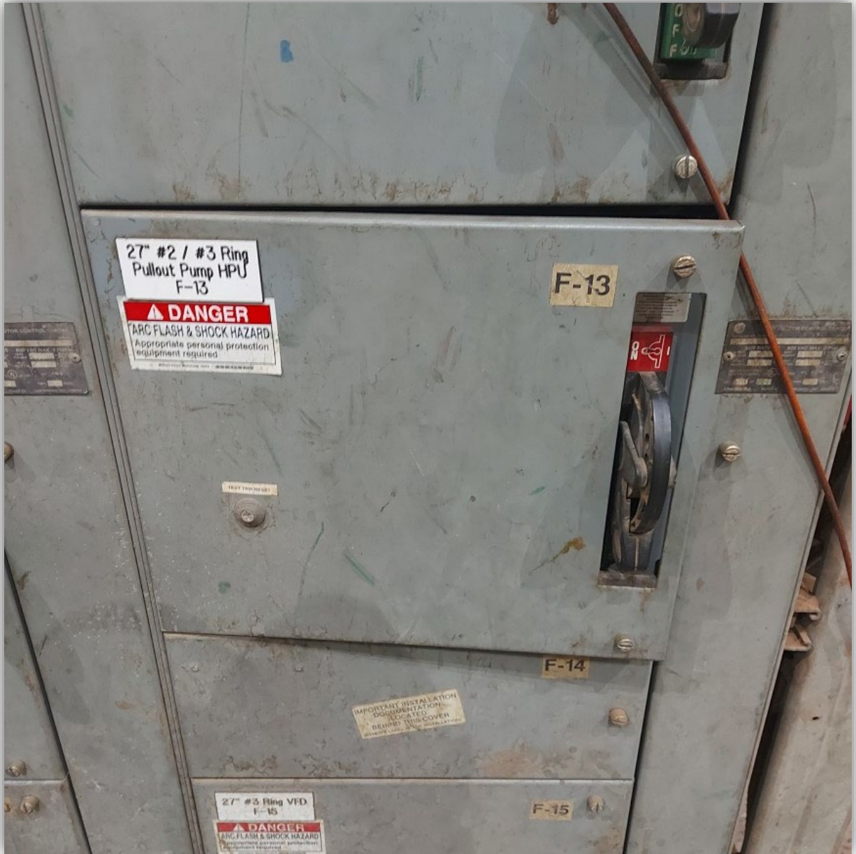
Image 1 - Front of Motor Control Centre (MCC) Bucket.
