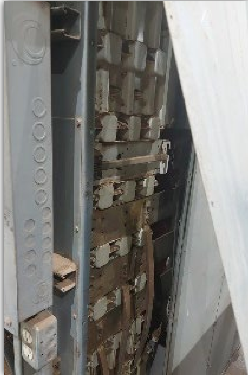
Image 4 - Rear of Motor Control Centre (MCC) with cover removed to inspect for any damage from the arc-flash incident (Image supplied by Mill Manager).
