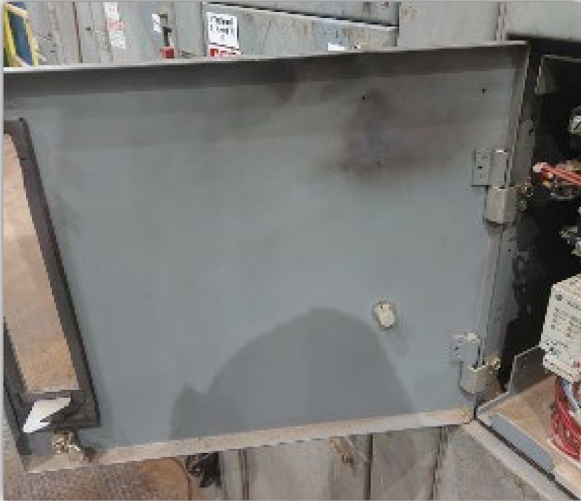
Image 3 - Door of Motor Control Centre (MCC) Bucket showing some charring and soot from the arc-flash incident.
