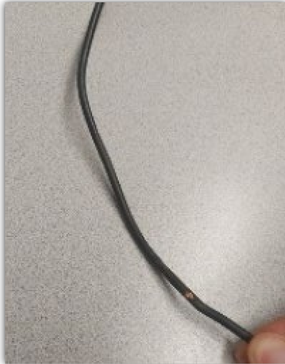
Image 5 - TEW 600volt wire from phase "A" that arced. Worn to copper where it arced due to friction on mounting bracket components in the MCC.
