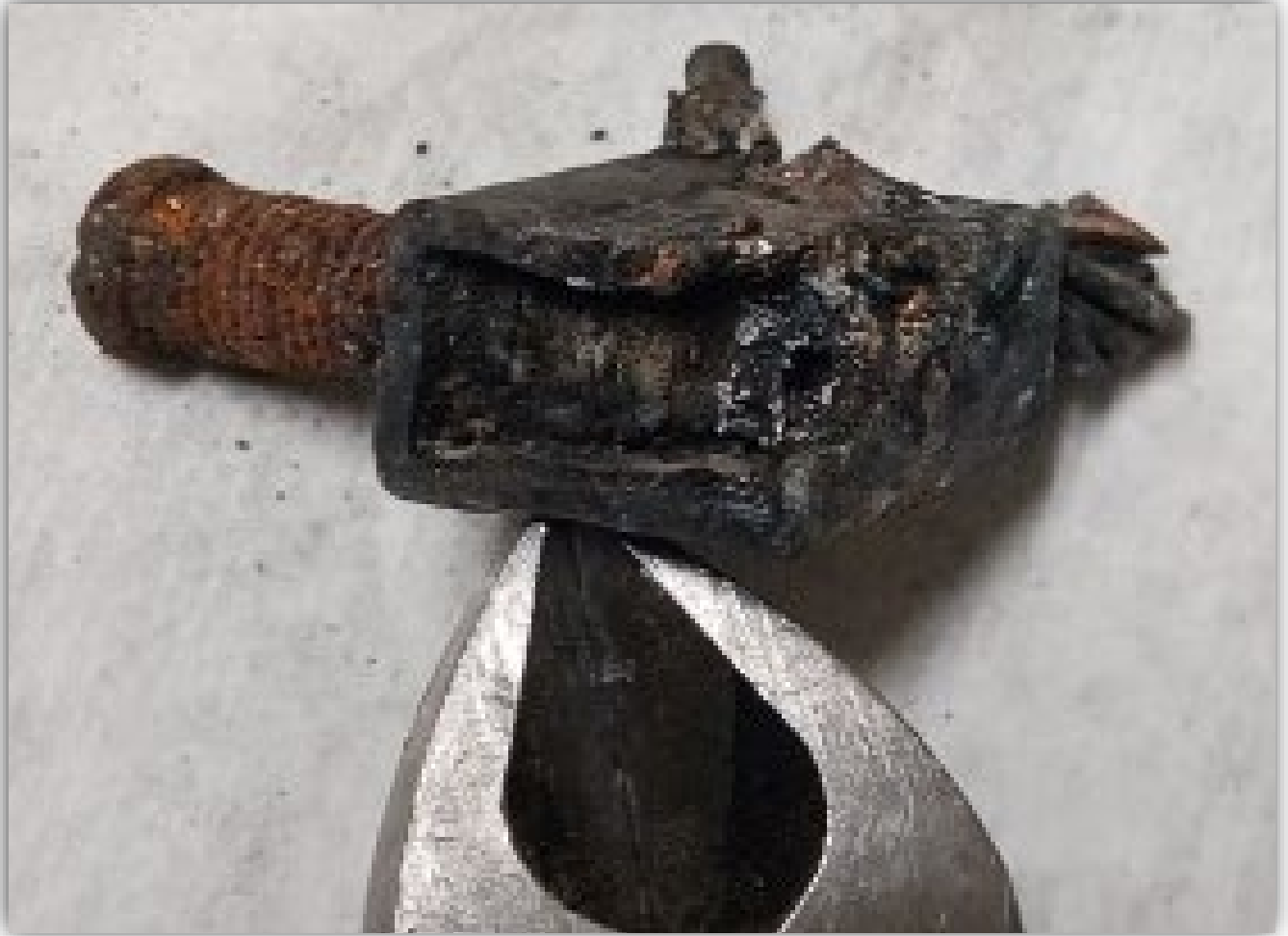
Image 3 – Termination lug involved in arcing incident.
