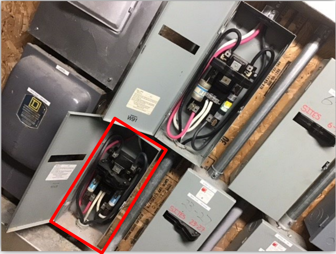
Image 5 – New fuses installed for supply to sites 17 through 22.
