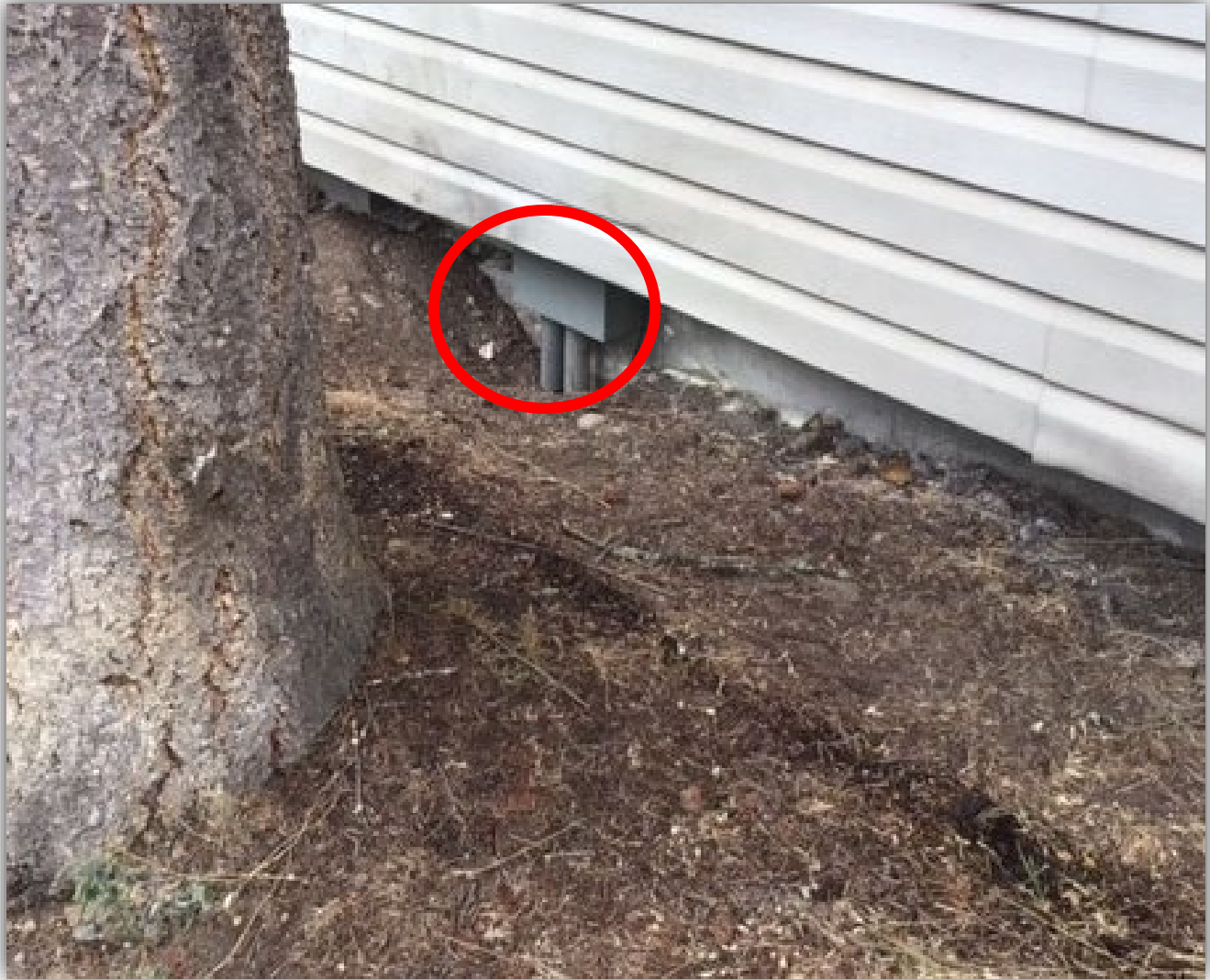
Image 2 – Southeast corner of power shed - grass fire occurred below exterior junction box.
