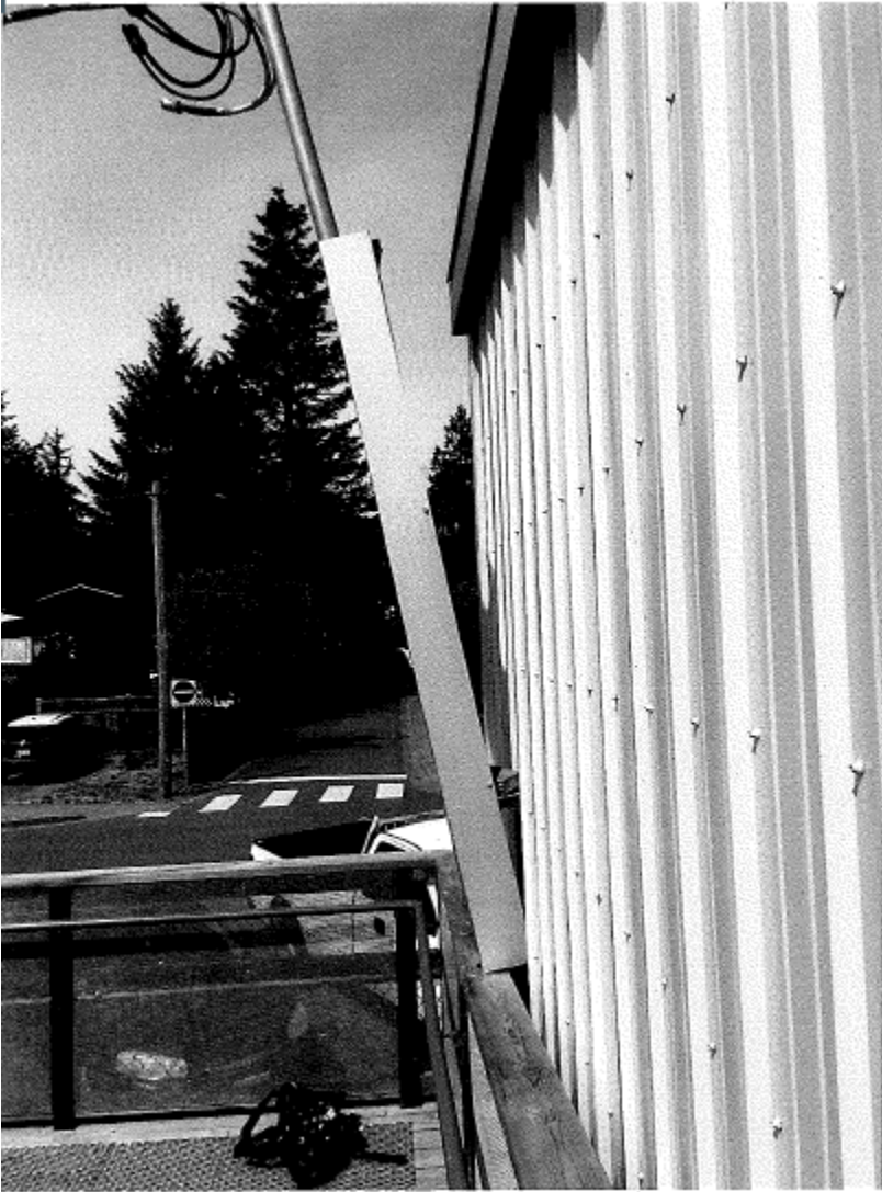
Photo 2: Close up of mast after repairs had occurred and been completed. (provided by FSR).
