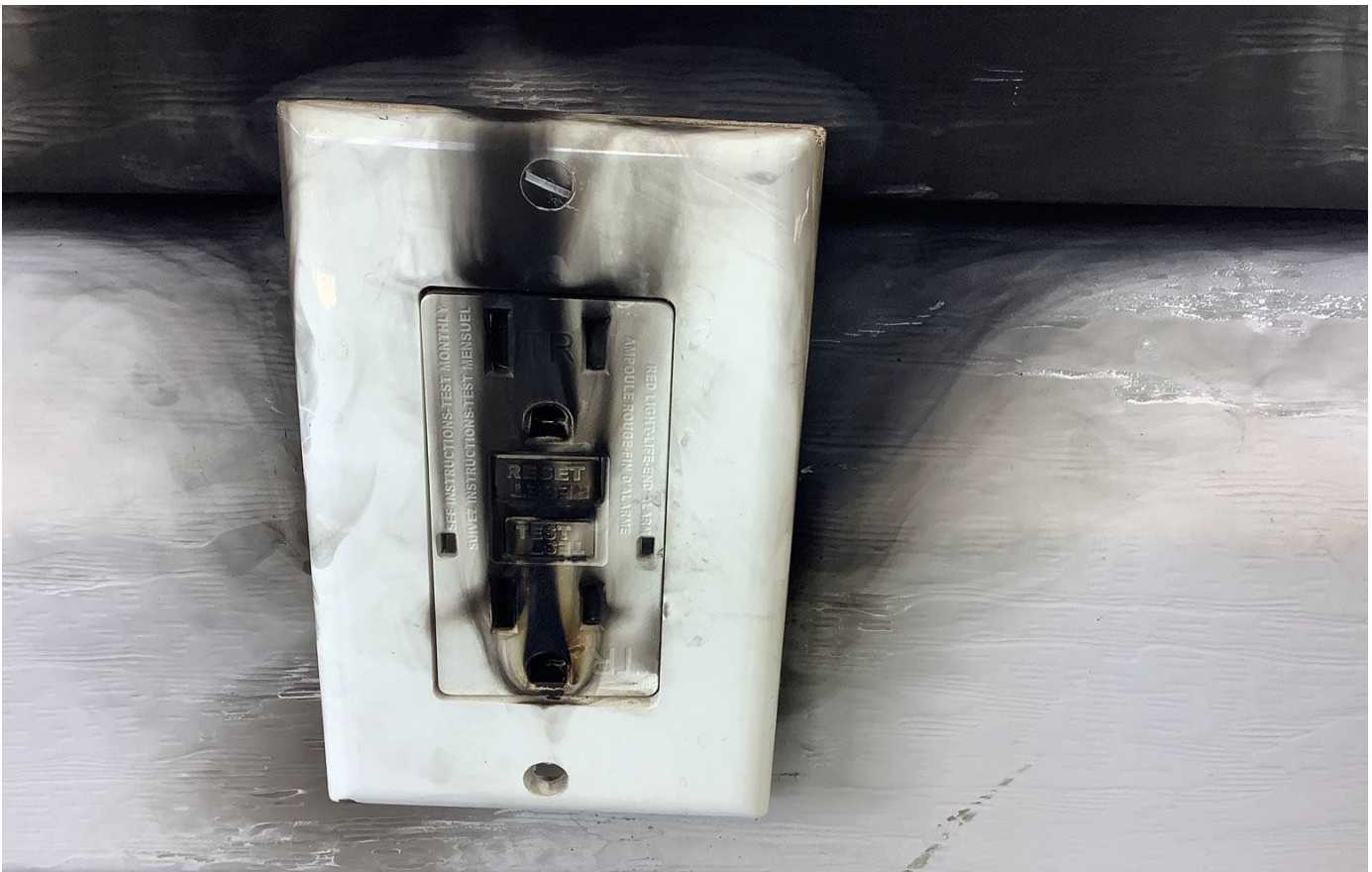
Image 1 – Exterior deck receptacle with dry location cover.
