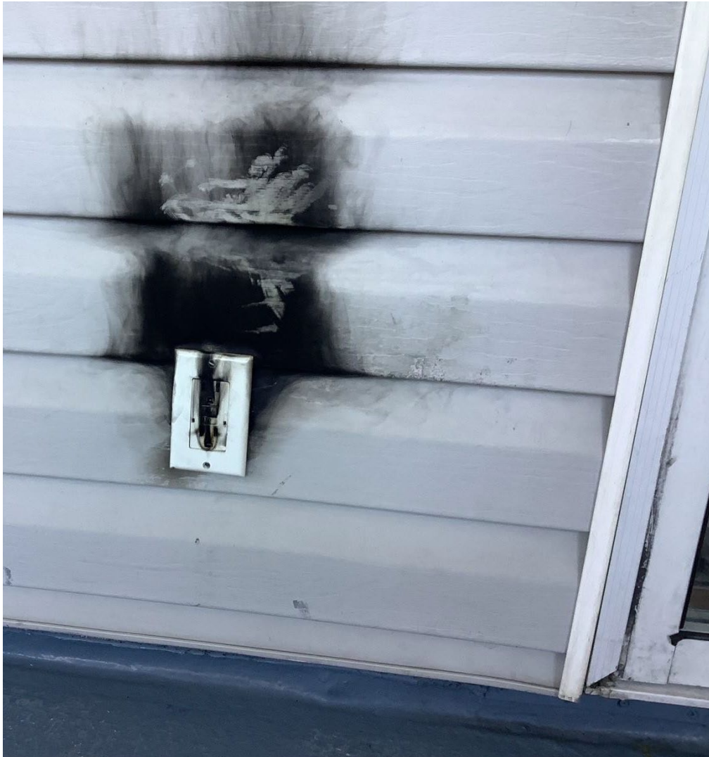
Image 2 – Damage to exterior siding and receptacle
