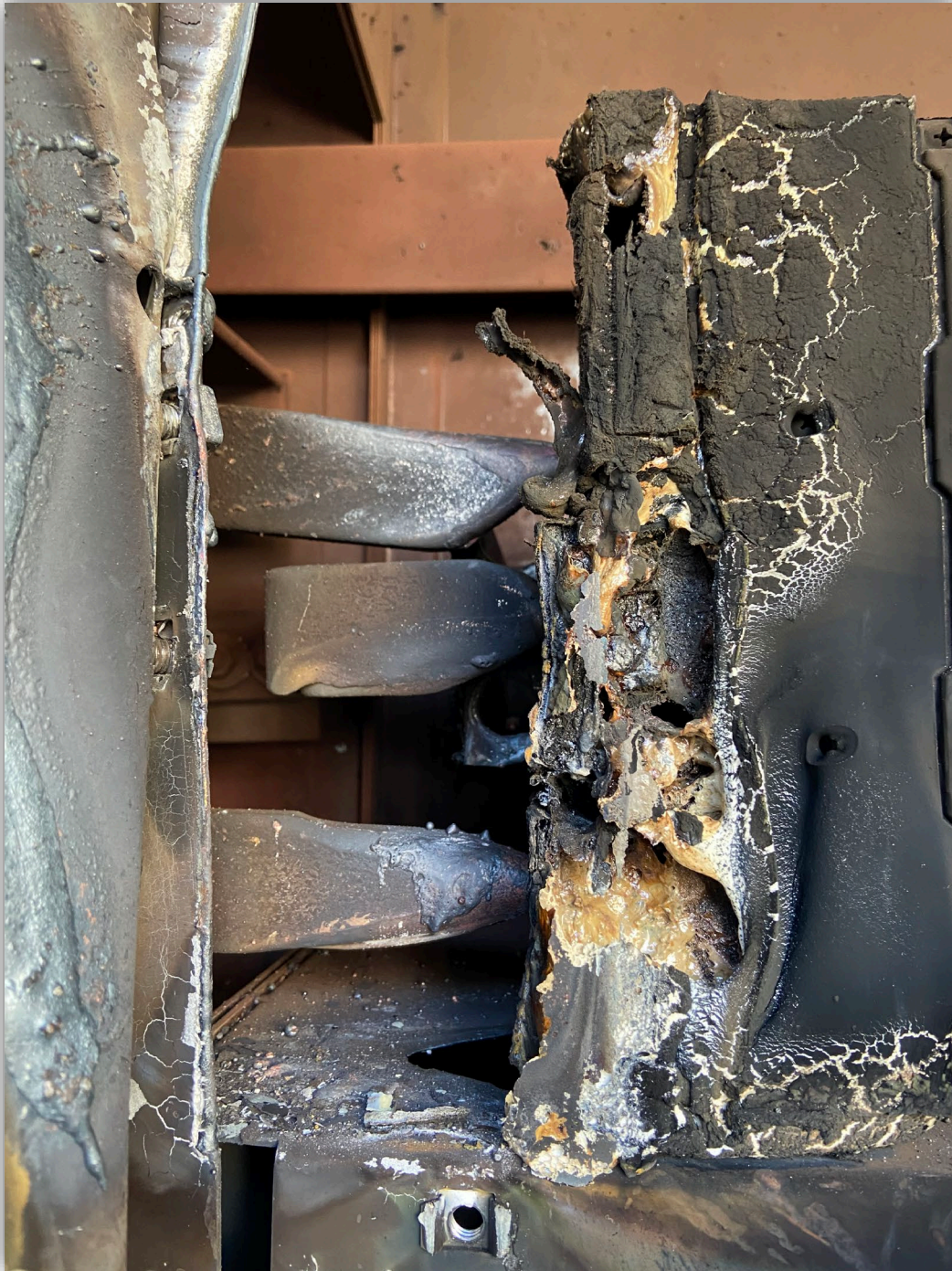
Image 1 - Melting of bus bars due to arcing fault.
