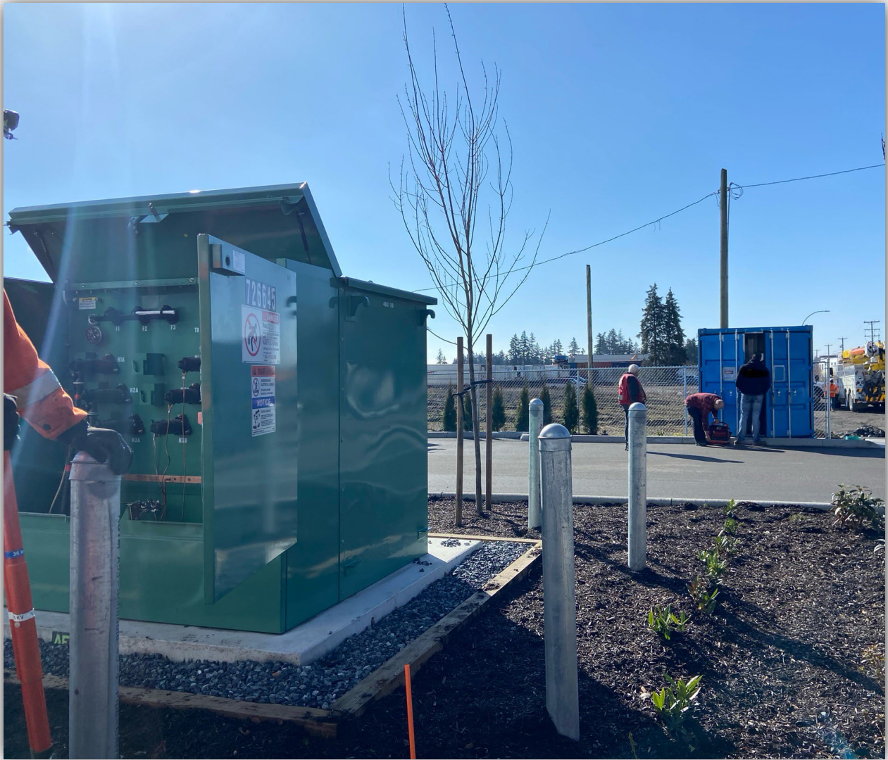
Image 4 – Overall site layout of temporary service equipment and utility transformer.
