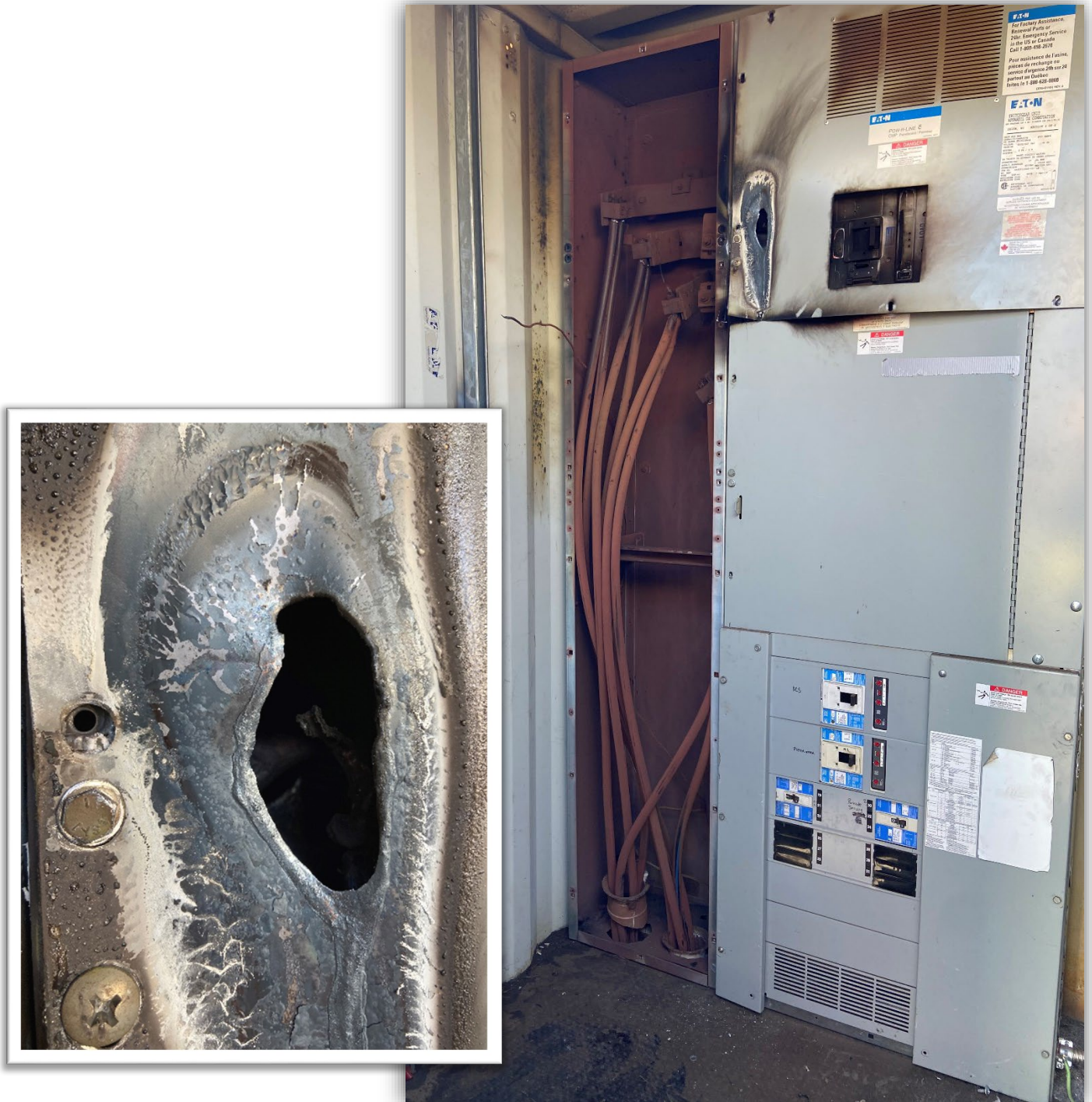
Image 3 – Overall damage to main distribution equipment. And close up of the hole melted through front of MDC due to arc flash.
