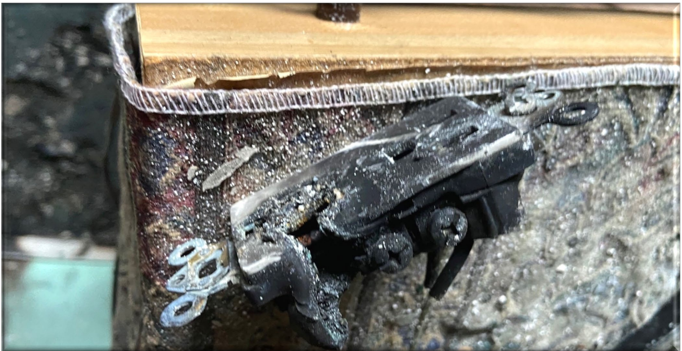
Photo 6 – Melted receptacle was the point of origin of the fire.
