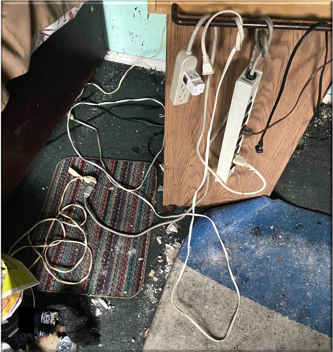
Photo 2 – Power bars and multi-outlet adapters that were connected to the overheated receptacle.
