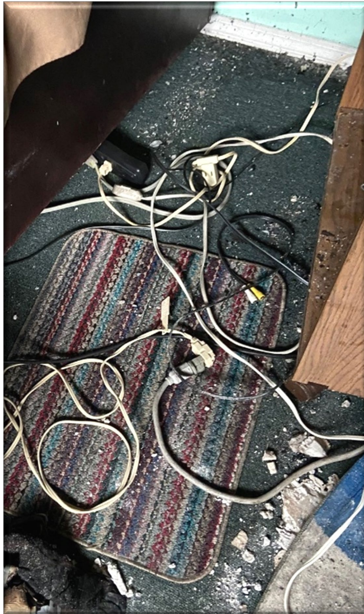
Photo 3 – Additional power bars connected downstream from power bars in Photo 2 .
