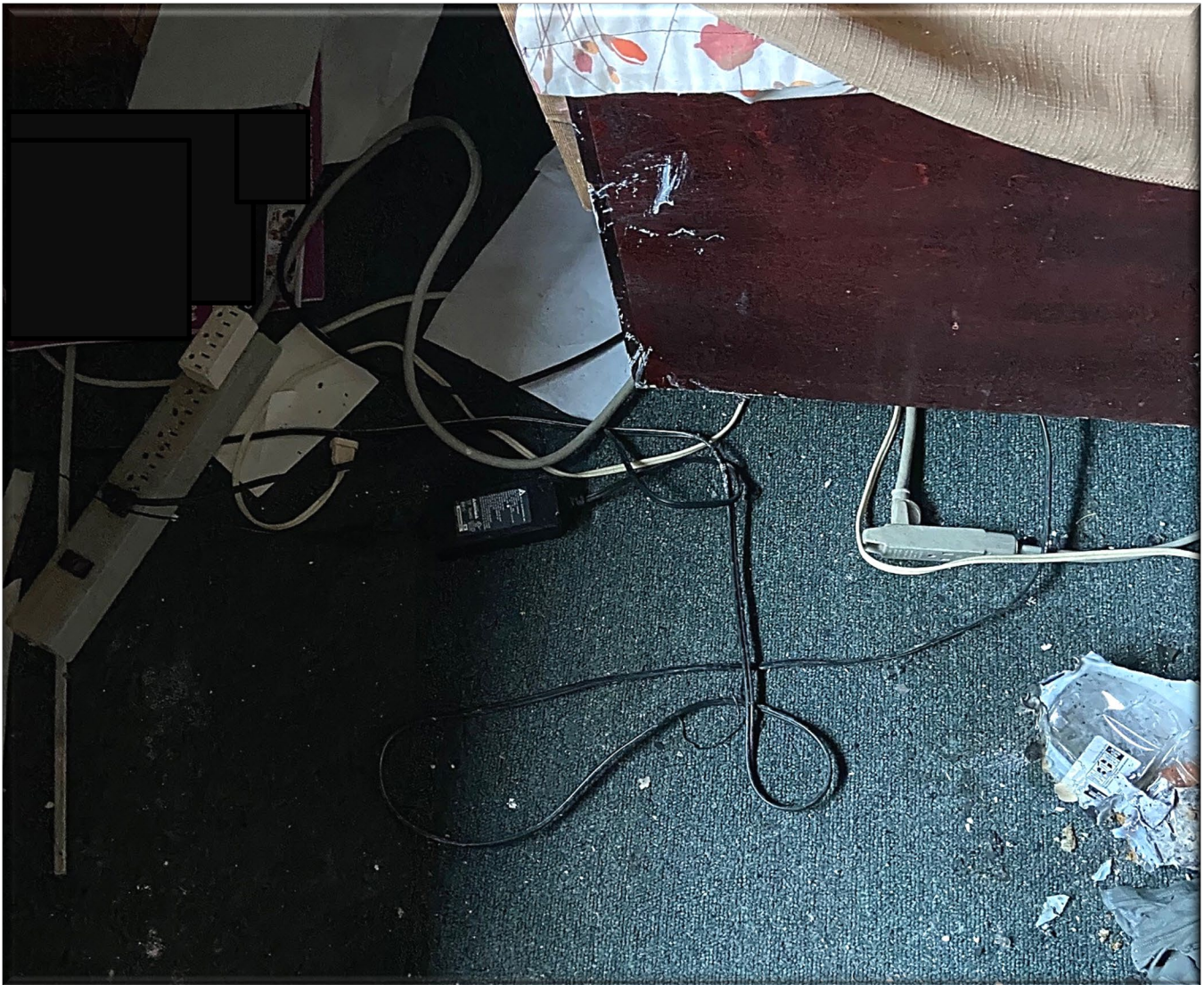
Photo 4 – Further power bars connected downstream from power bars in Photo 3 .
