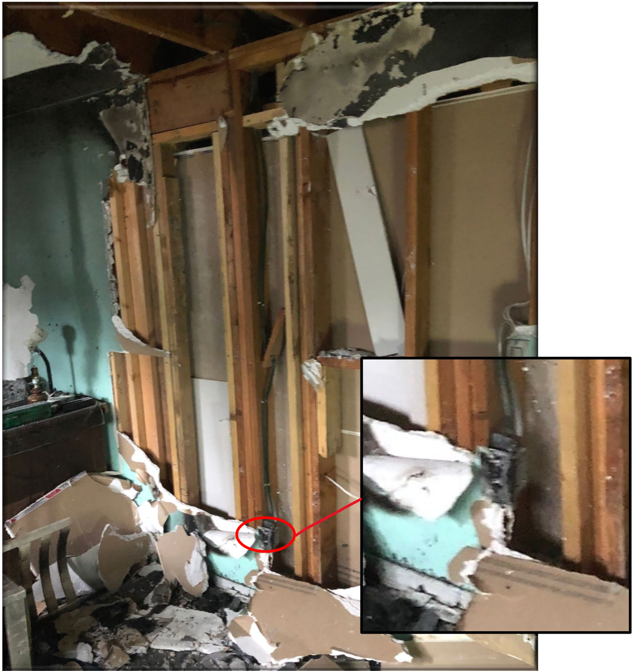
Photo 1 – Area of fire damage including point of origin of fire (red outline).
