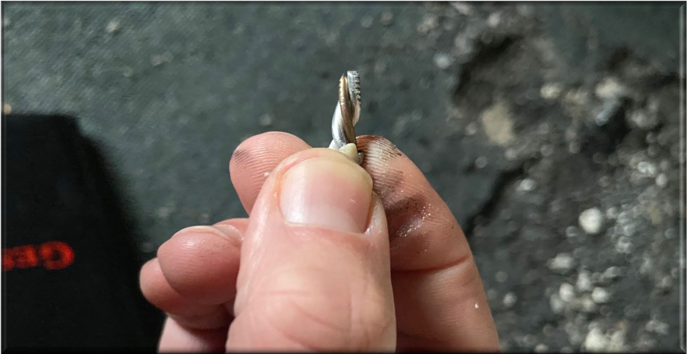
Photo 5 – Wiring connected to receptacle where fire originated shows no signs of overheating.
