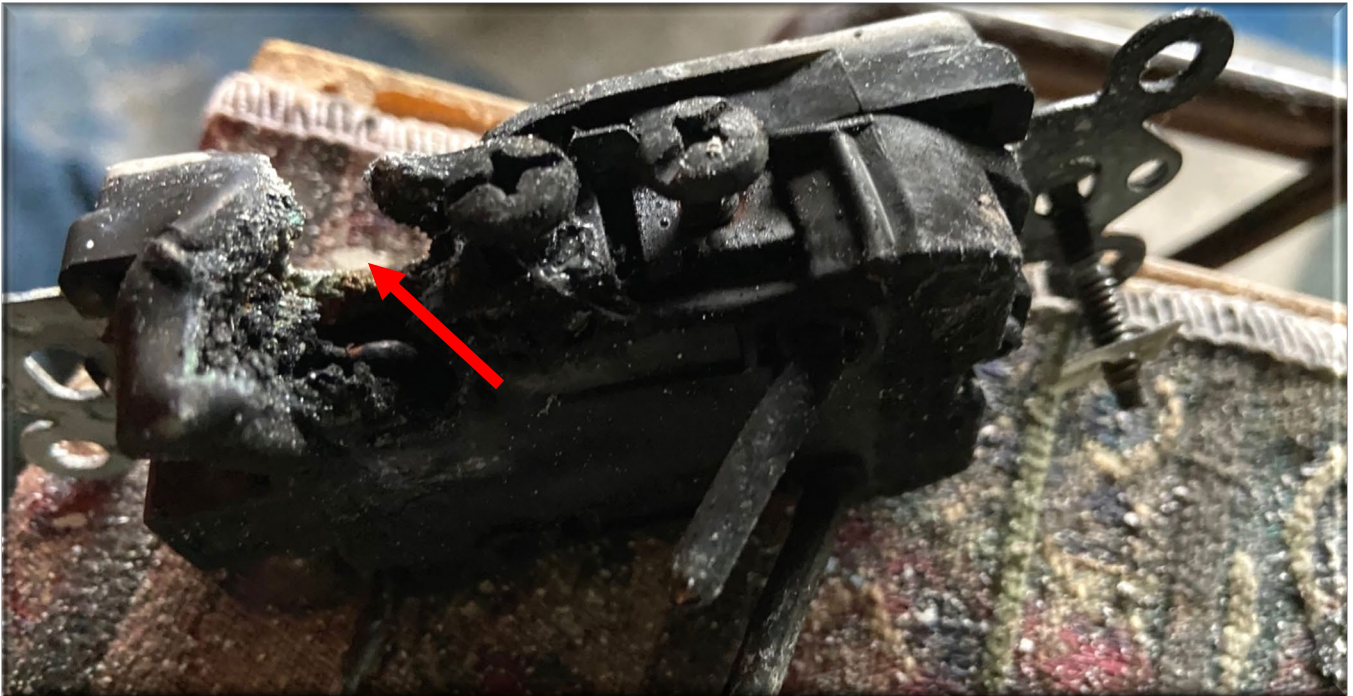
Photo 7 – Closeup of overheated receptacle showing that point of origin was the internal connection point for a cord end (red arrow).
