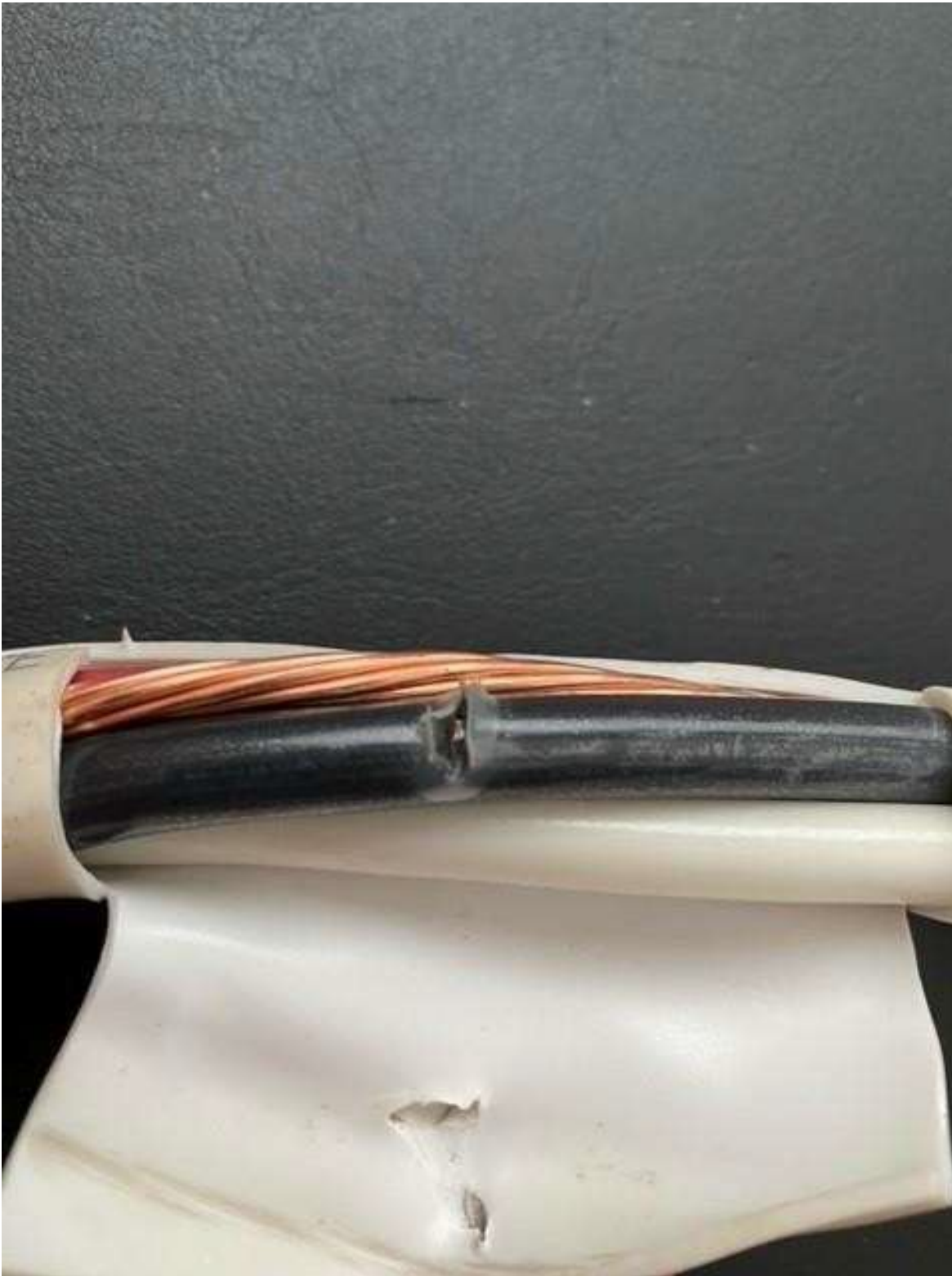
Photo #7 – Damage to conductor insulation of feeder cable.
