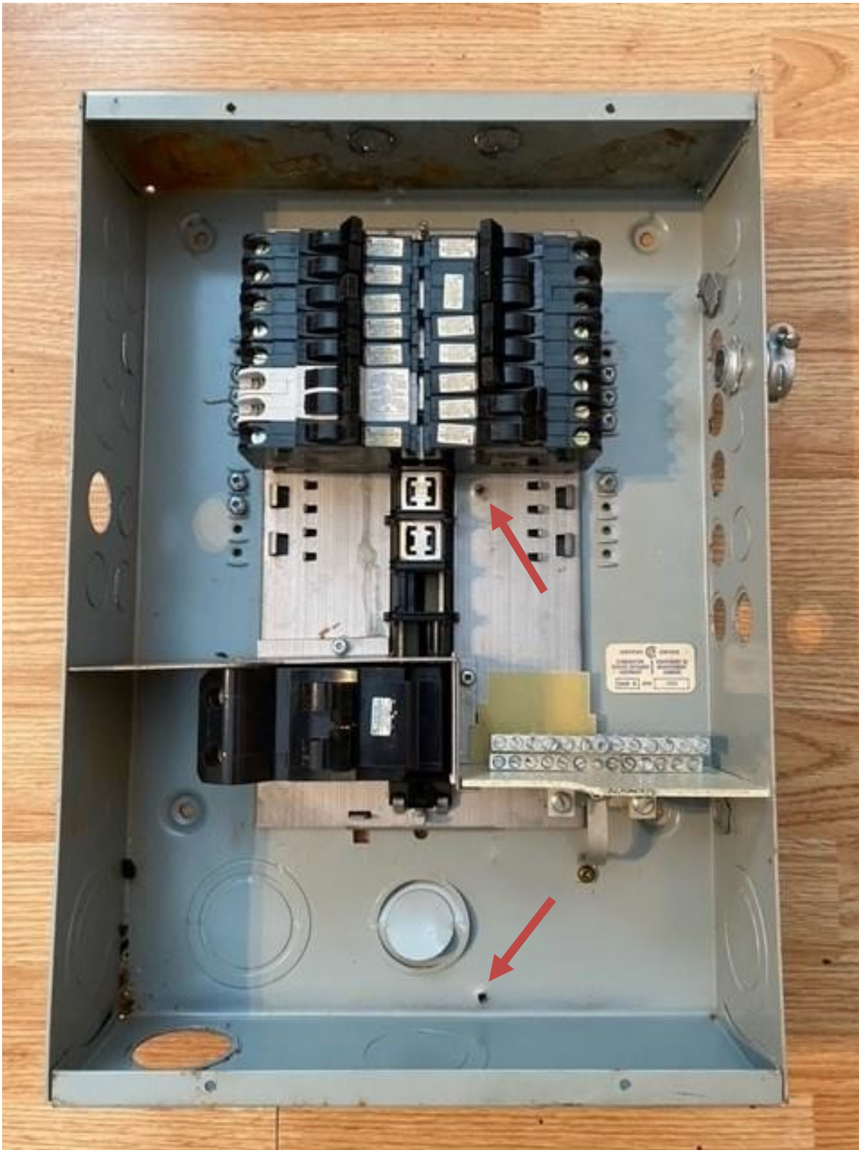
Photo #2 – Interior compartment of main distribution panelboard
