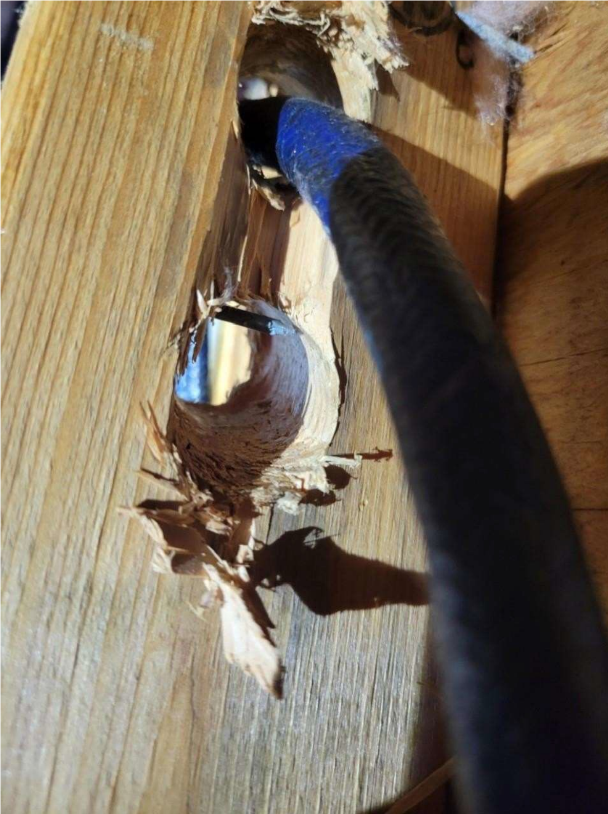
Photo #8 – Hole in 2x4 stud showing the nail that caused the damage to the feeder cable.
