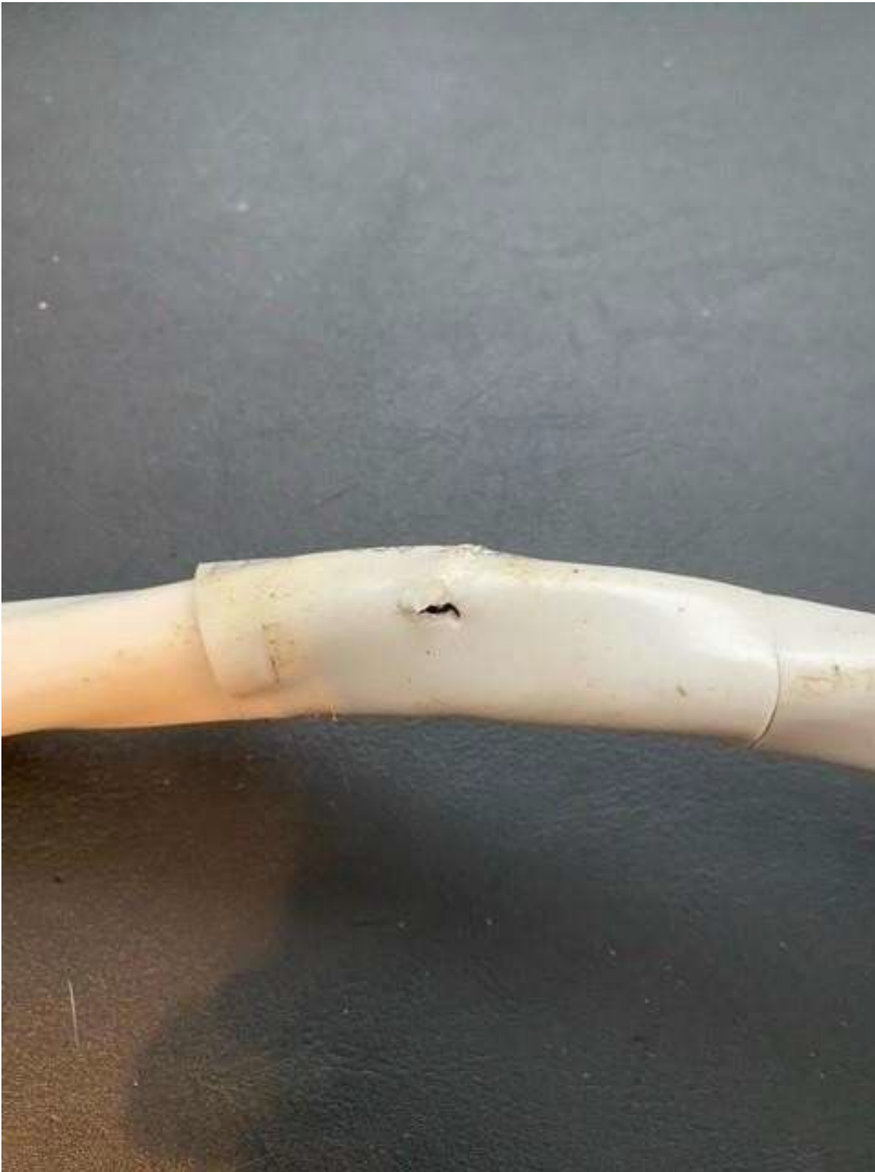
Photo #6 – Damage to outer jacket of feeder cable
