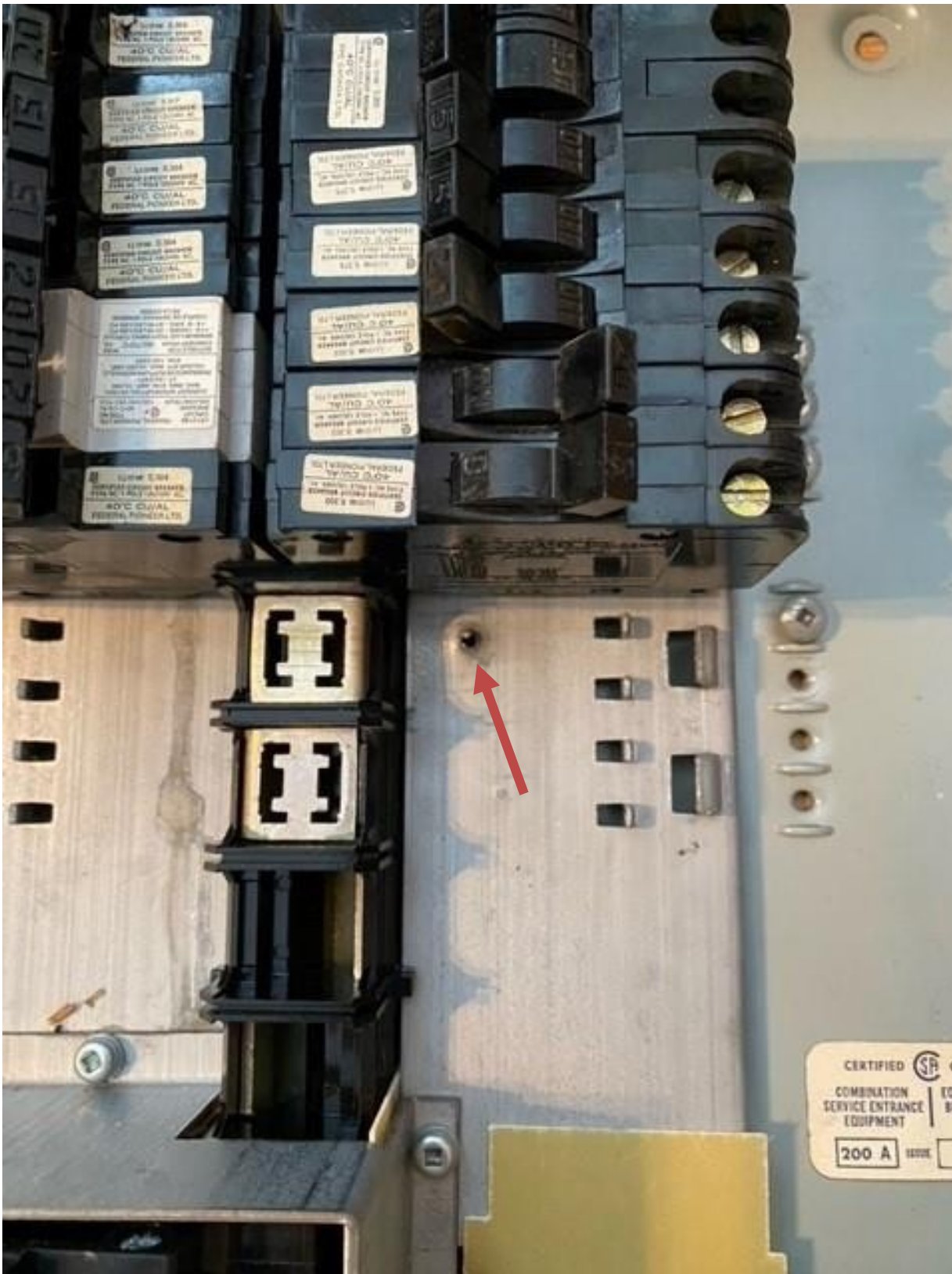
Photo #3 – Close-up of nail hole associated with damaged circuit breaker
