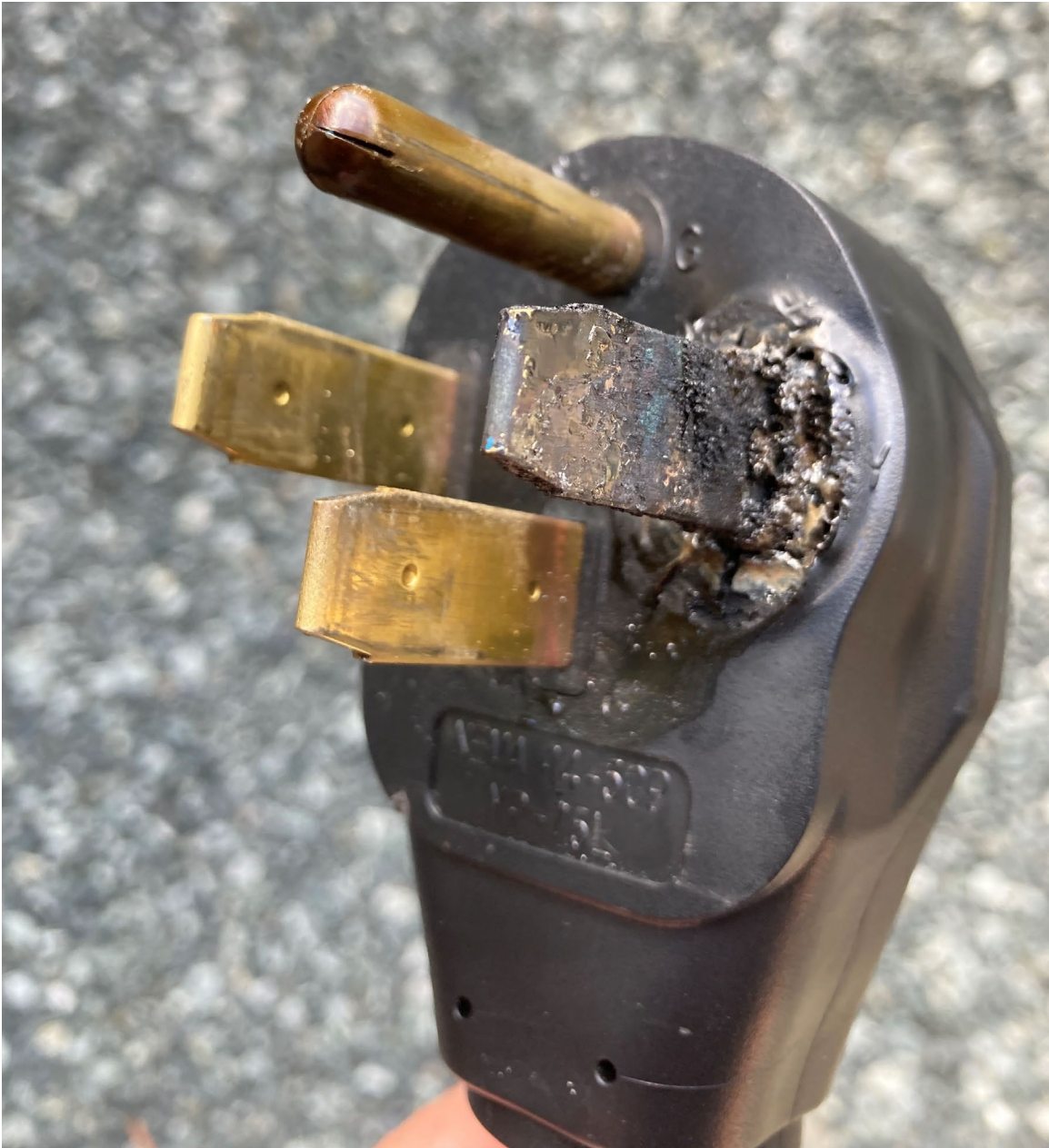
Figure 5 - Damage to plug
