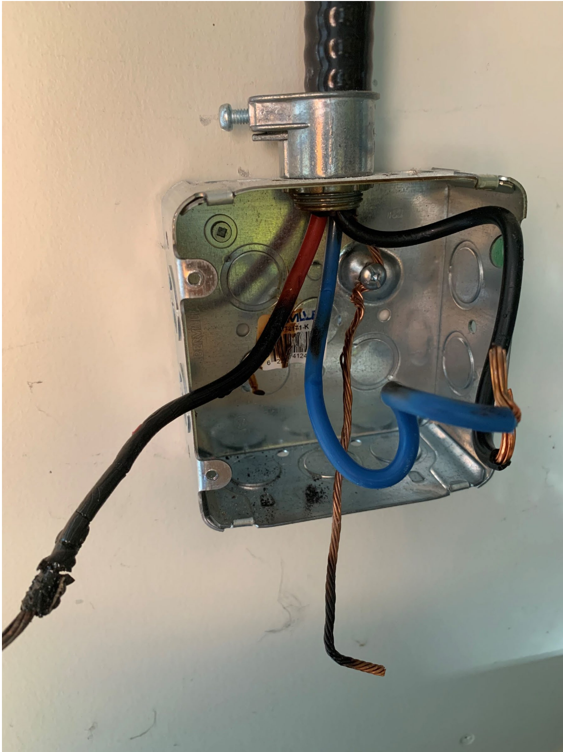
Figure 4 - Damage to conductor in enclosure
