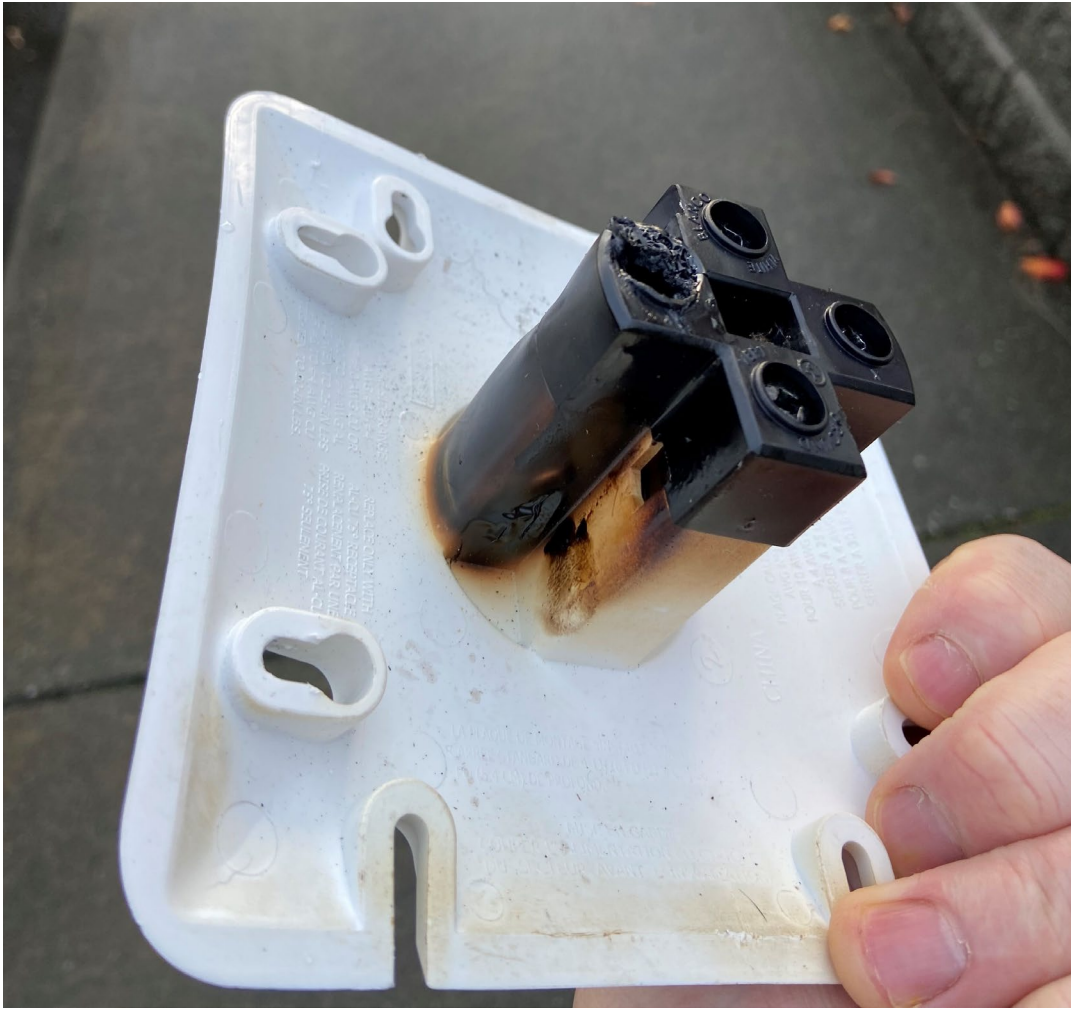
Figure 2 - Rear of receptacle
