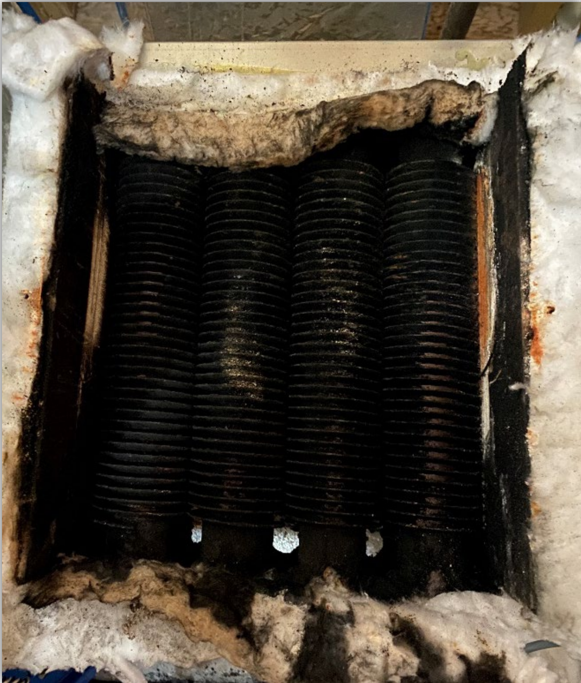
Image 1 - Soot blocking heat exchanger. The fins are covered in soot. This photo was taken after the unit failed. A gas fitter tried to clean after the fact as well.
