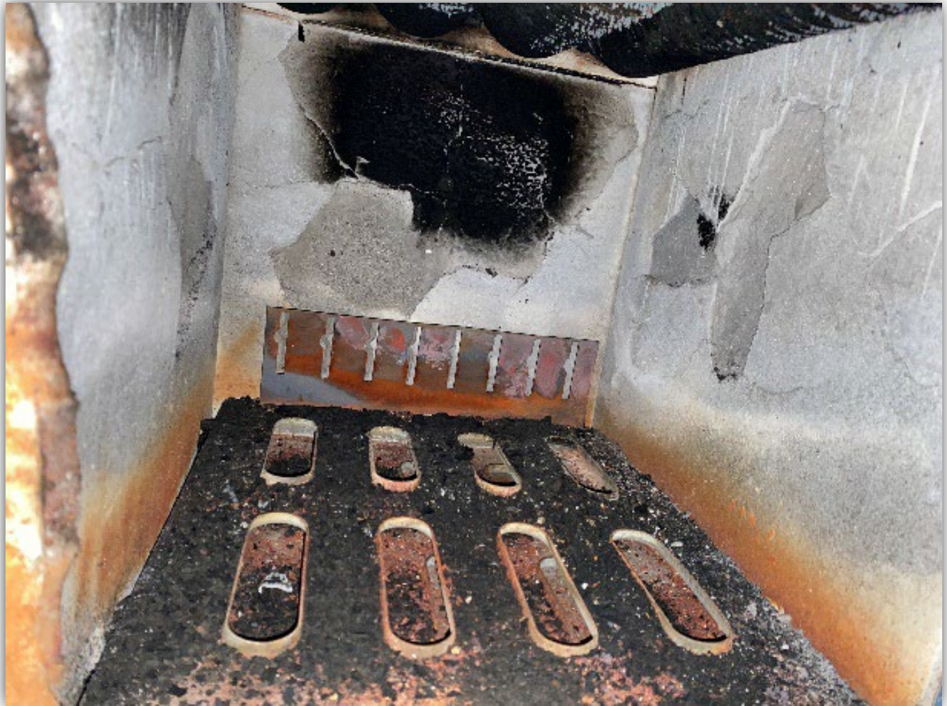
Image 2 - Burner compartment. The atmospheric burners were in this space. The soot at the rear of the burner compartment and cracking of refractory likely caused by flame impingement.
