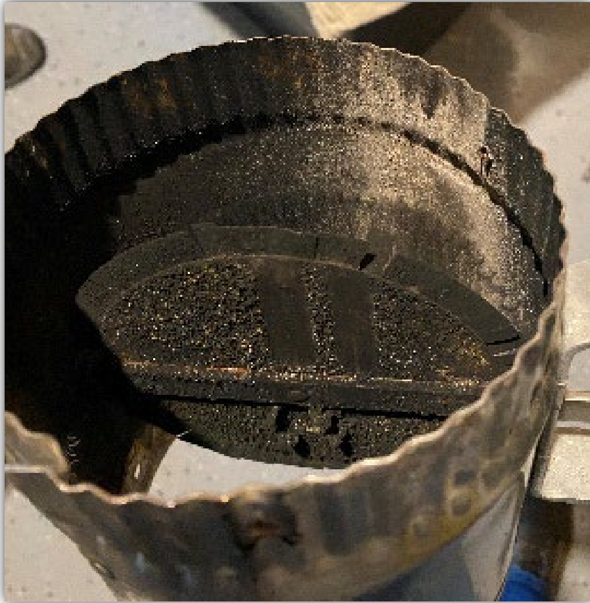
Image 4 - Soot inside flue. Soot is located through the flue to termination, this proves there was incomplete combustion during usage.
