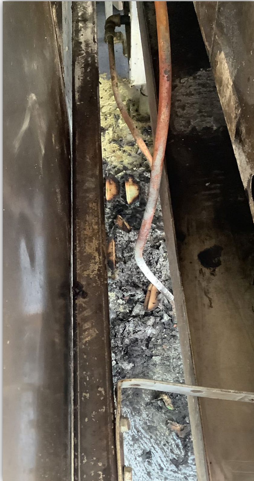
Image 5 – Fire damage behind gas appliances.
