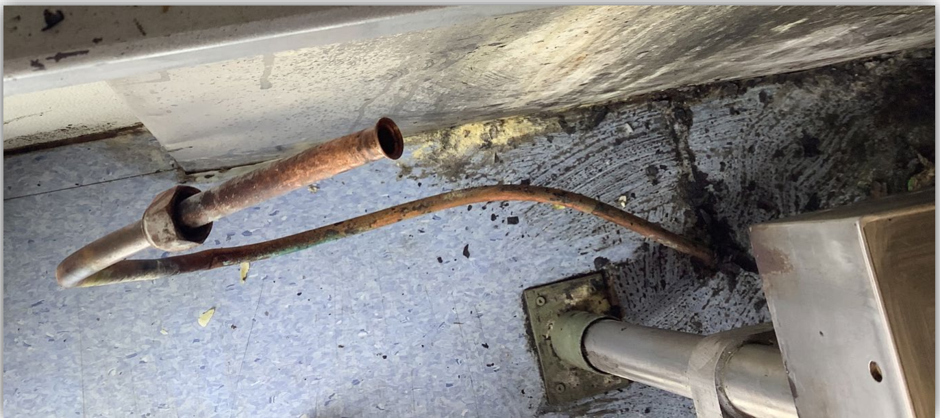
Image 4 – Uncapped gas line previously connected to the char-broiler.
