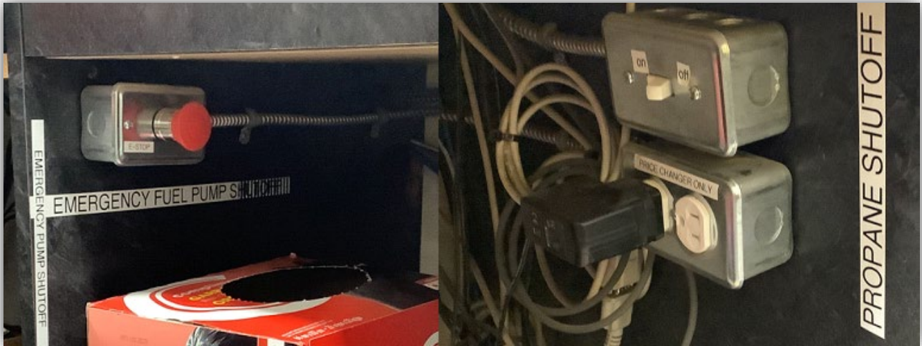
Image 2 – Emergency Fuel Pump Shutoff button was not shut off (Left) and the Propane Shutoff switch that was shut off when the propane leak occurred (Right).
