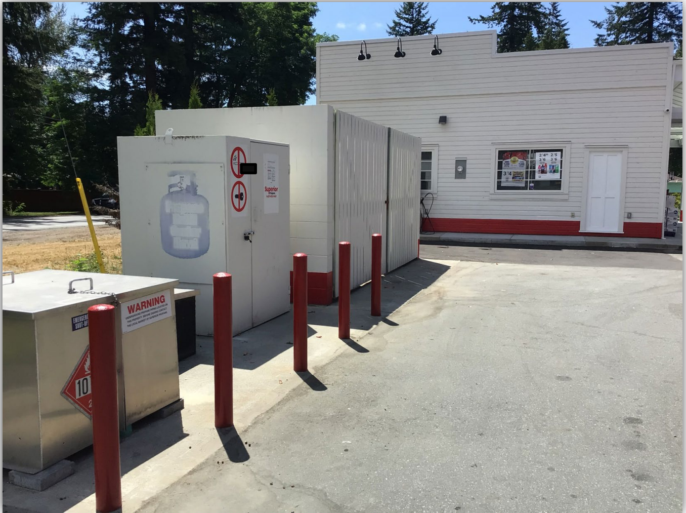
Image 1 – Propane cylinder fill cabinet (White) at fueling station.
