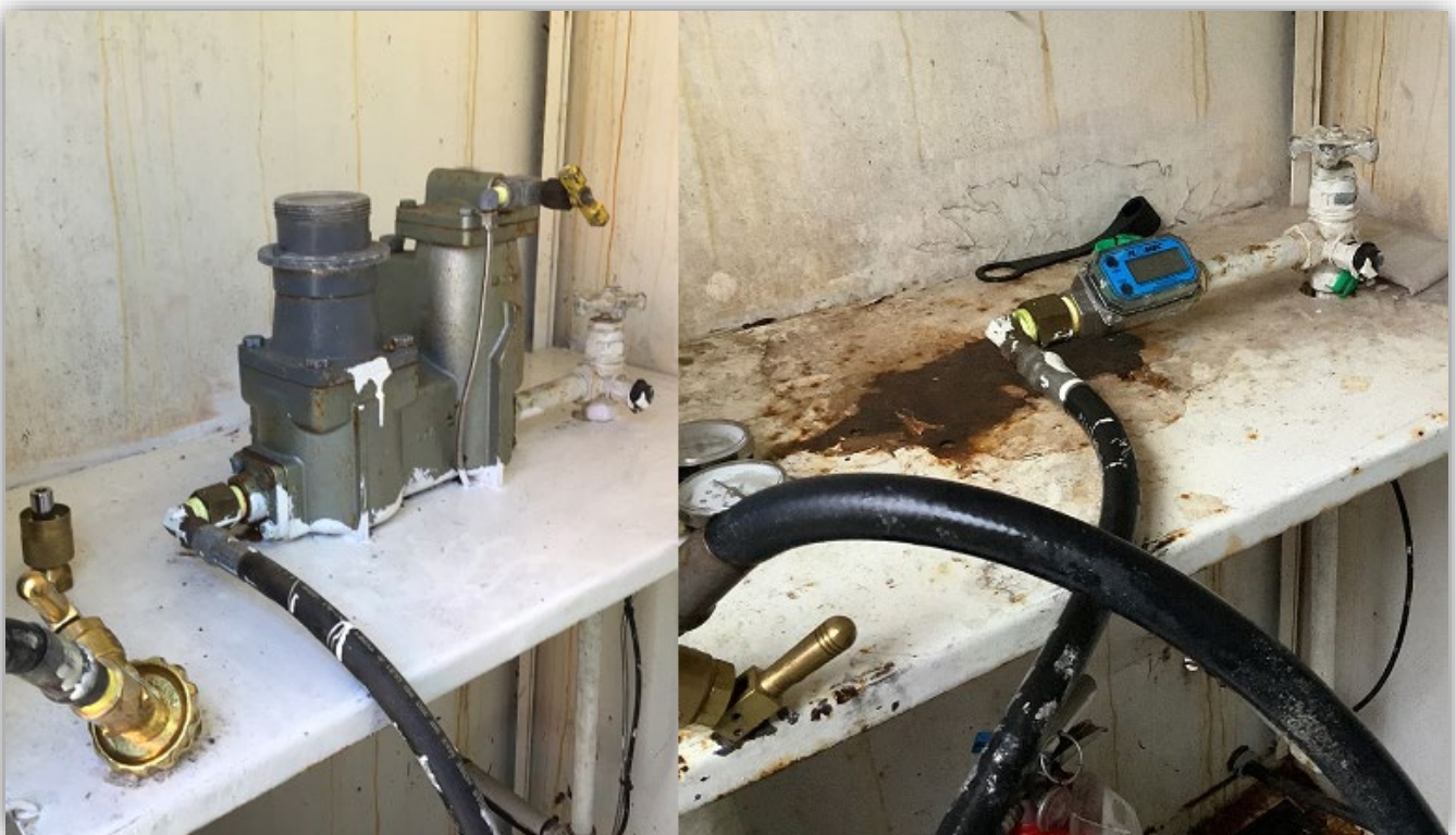
Image 3 – The previously installed mechanical propane cylinder fill meter (Left) and the replacement digital flow through meter (Right).
