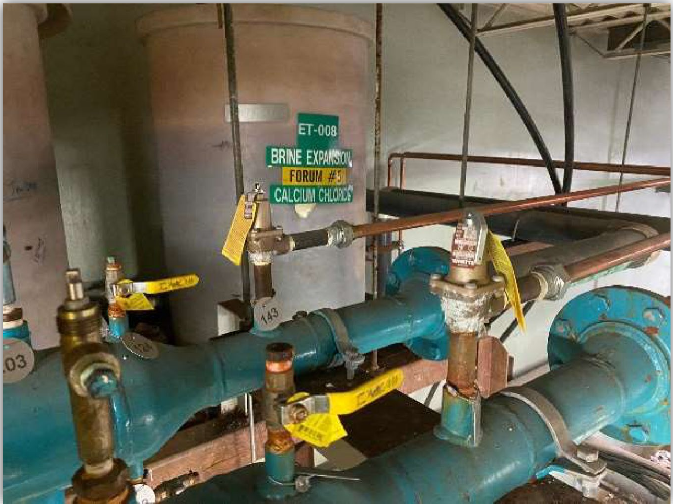
Image 1 - Failed heat exchanger Isolated and awaiting replacement.
