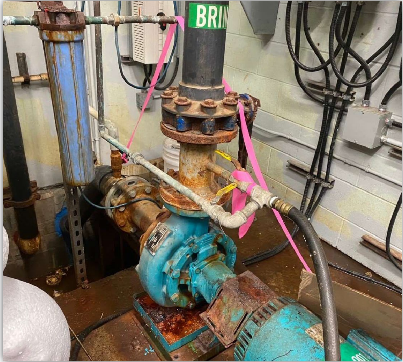
Image 3 - Isolated and locked out brine circulating pump.
