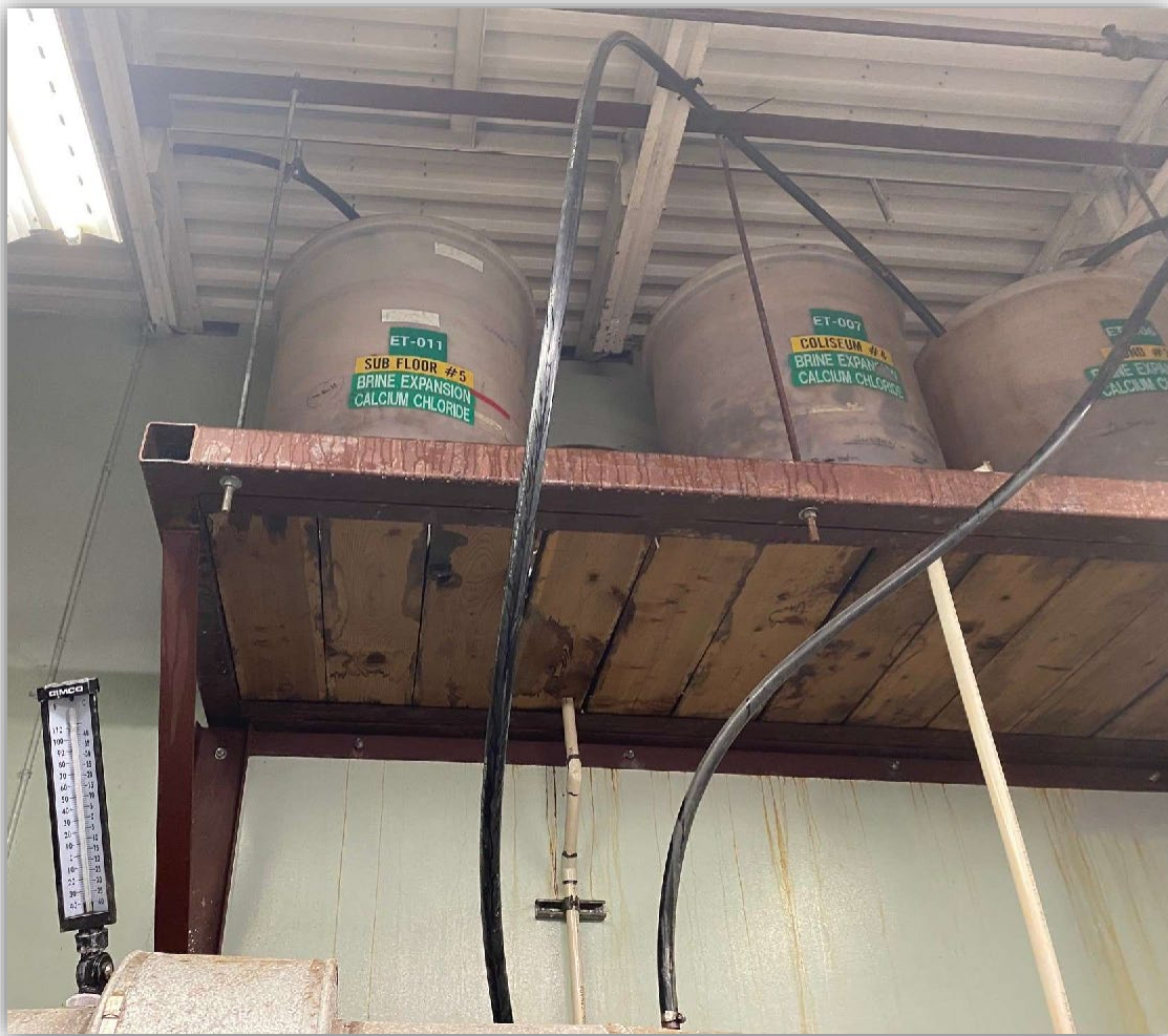
Image 2 - Open expansion tank for the brine where ammonia gas escaped into the mechanical room and liquid brine spilt down below to an open sump.
