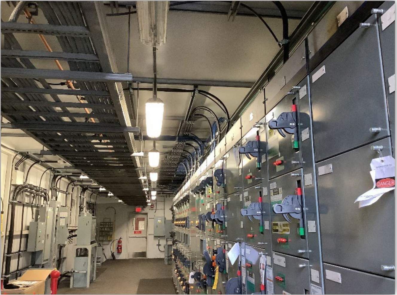
Photo 1 – MCC in the electrical room.
