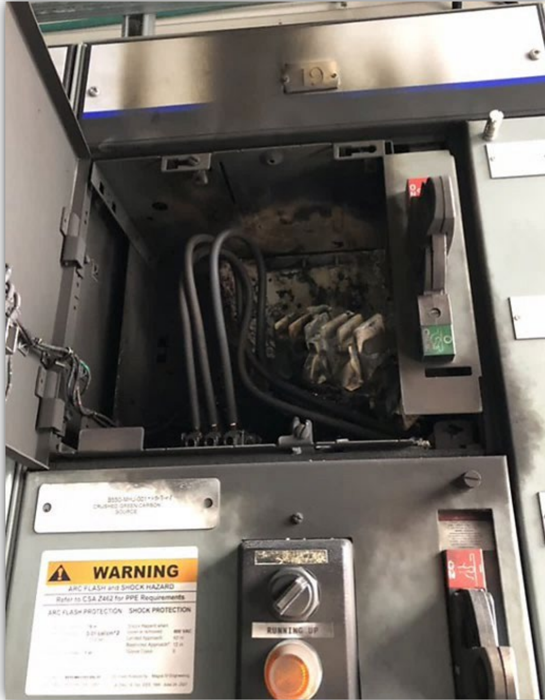
Photo 2 – MCC bucket with burn damage.
