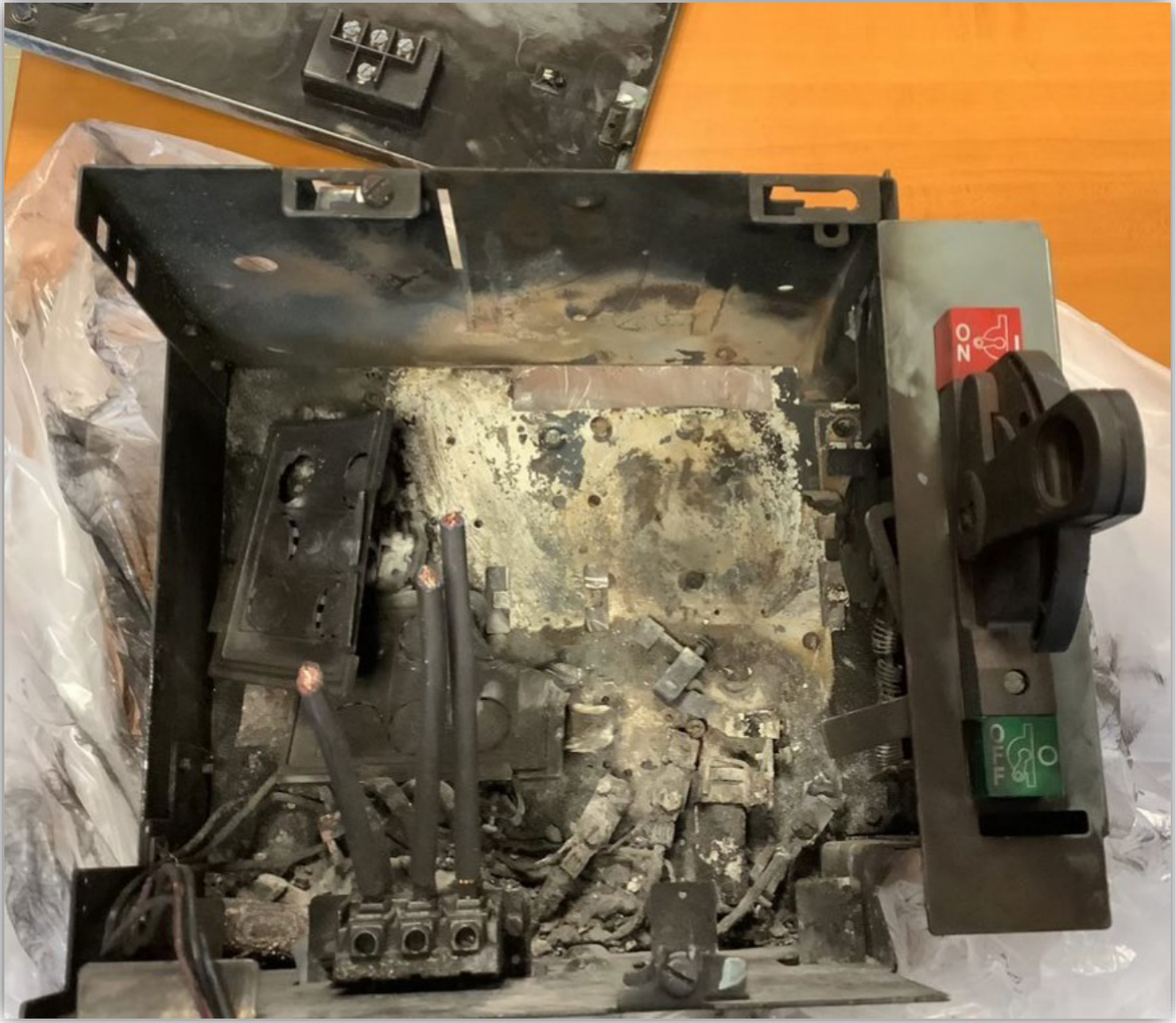
Photo 4 - Damaged MCC bucket removed from unit.
