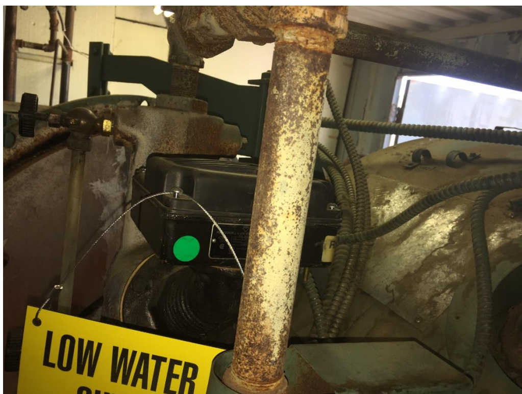
Low water cut off device
