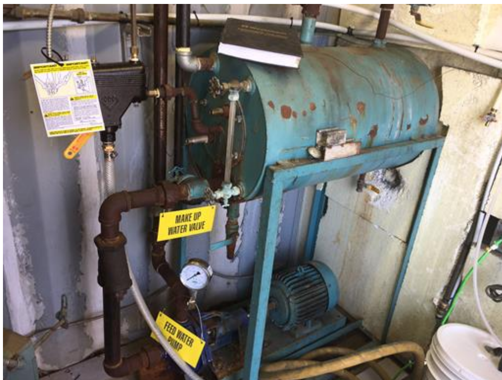
Boiler feed-water tank and pump
