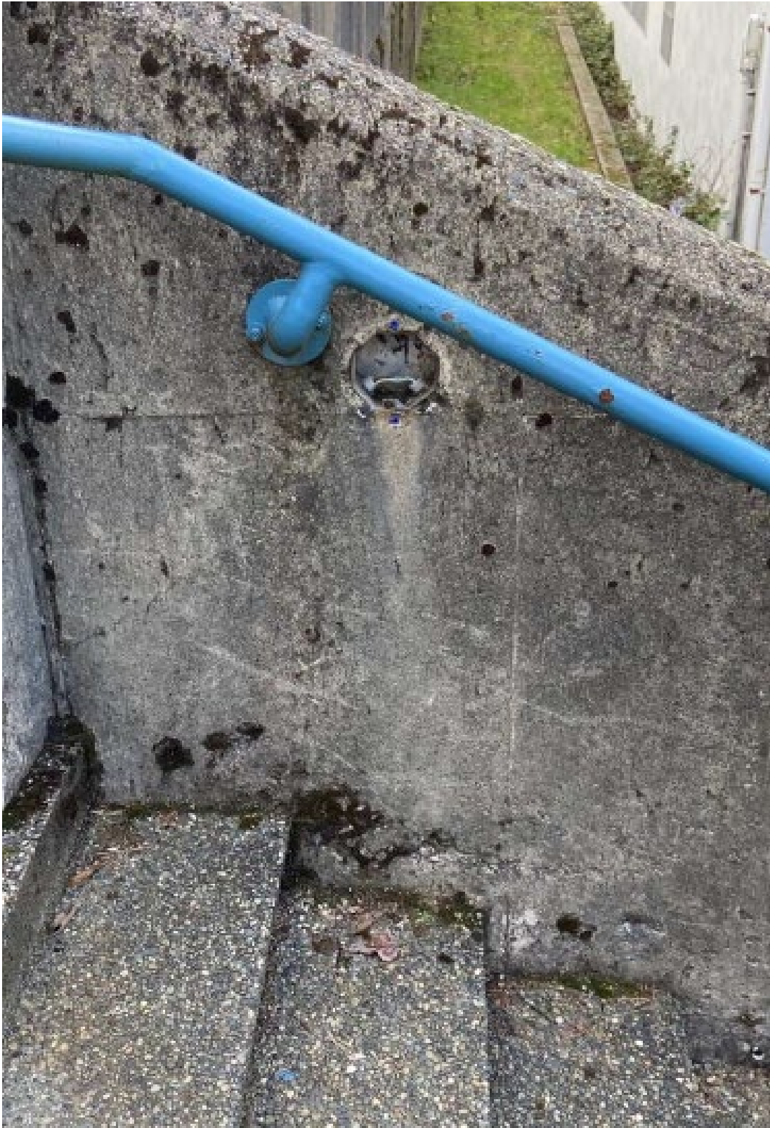
Image 4 - Stairs and junction box.
