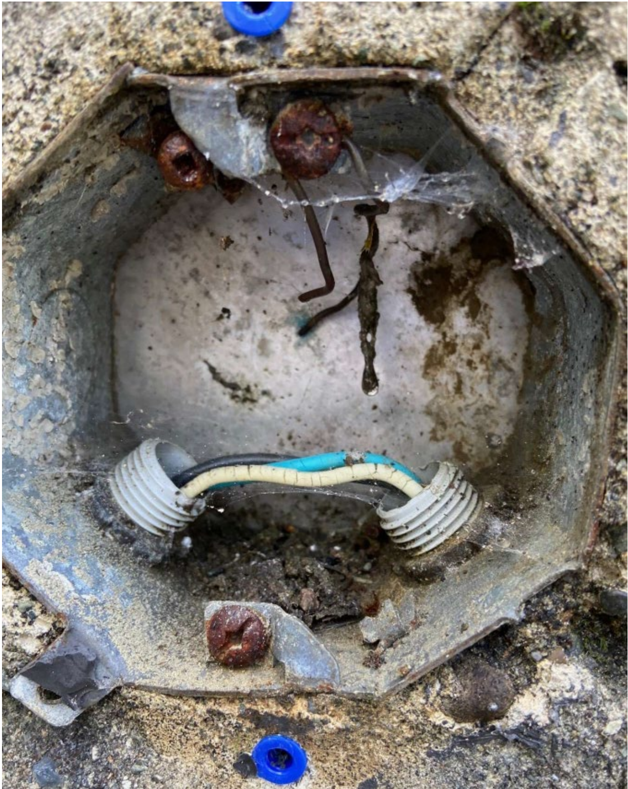
Image 2 - Deteriorated insulation on circuit conductors.
