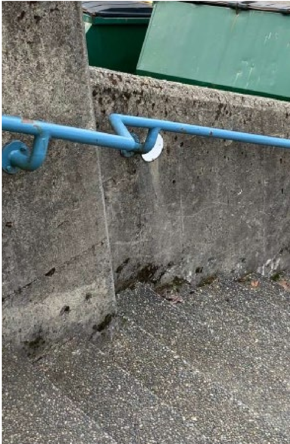
Image 3 - Junction box location on stairs.
