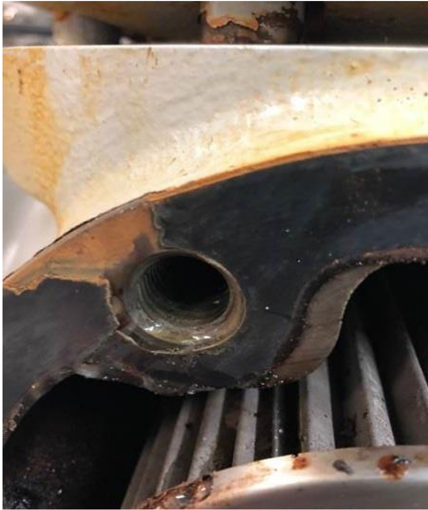
Photo 4: Photo provided by Refrigeration Contractor and used with permission. Not failure on bottom left side of gasket below bolt hole. Also rust on suction valve body where gasket was missing above the bolt hole.
