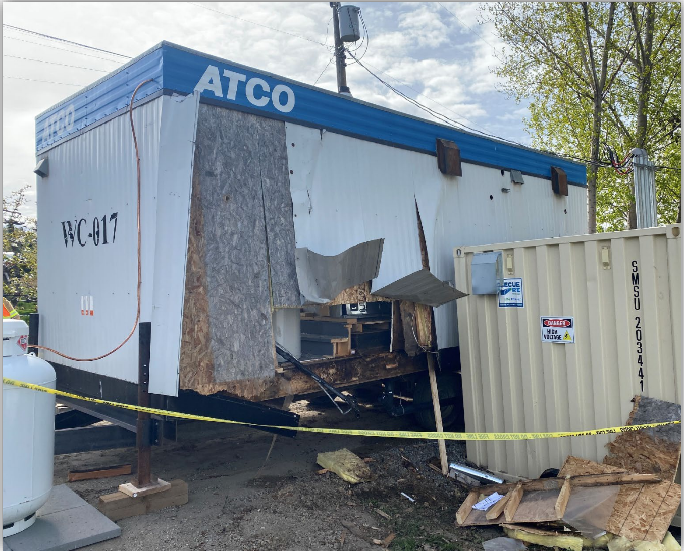
Image 2 – Rear of trailer showing damage from explosion and fire department overhaul.
