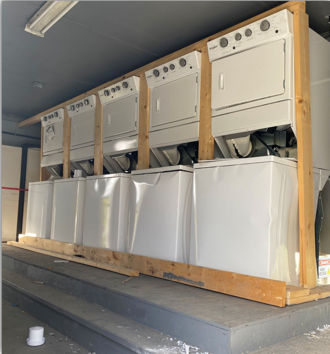
Image 3 – Five Stacker washer and gas dryers installed in trailer.
