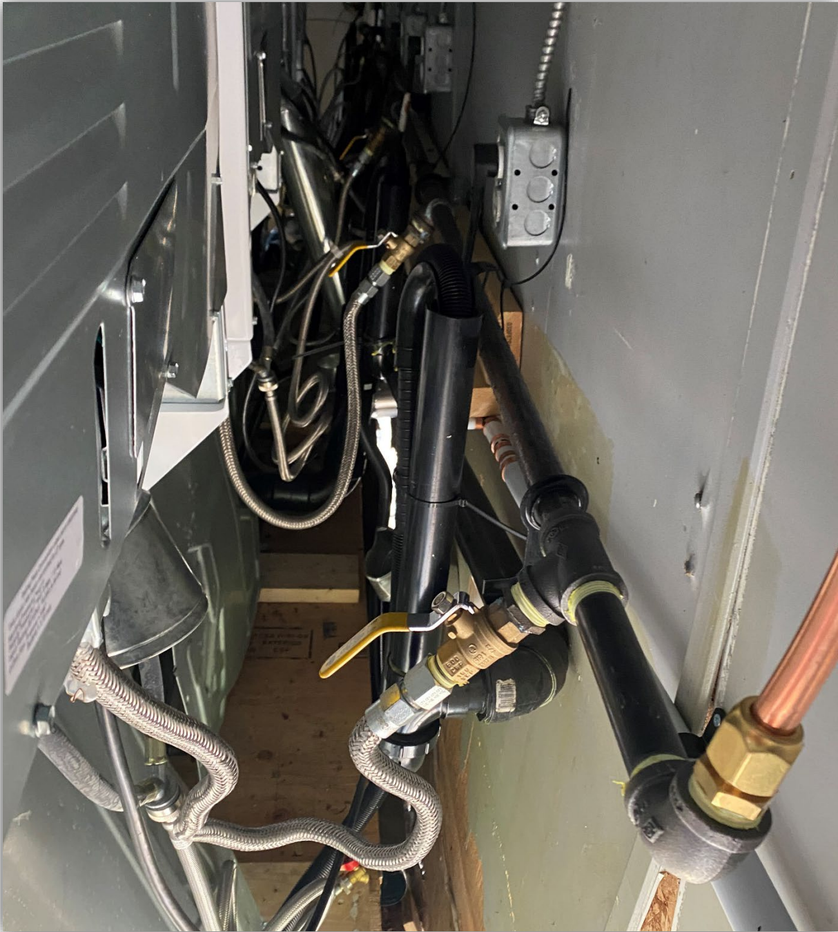
Image 4 – Rear of appliances showing factory appliance connectors, pre-existing gas manifold and shut off valves, and new copper gas tubing and brass fitting.
