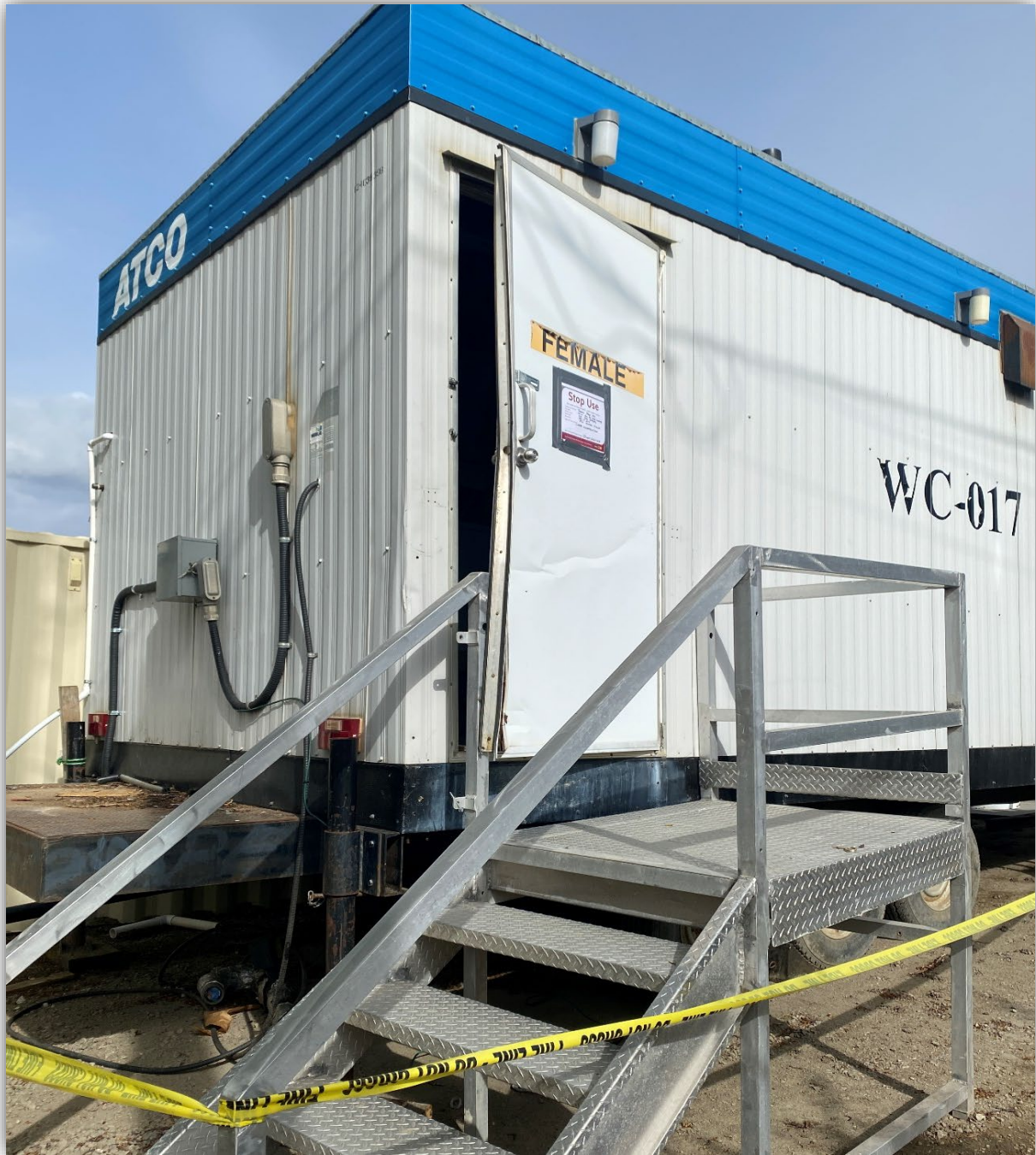
Image 1 – Laundry trailer showing door damaged from explosion.
