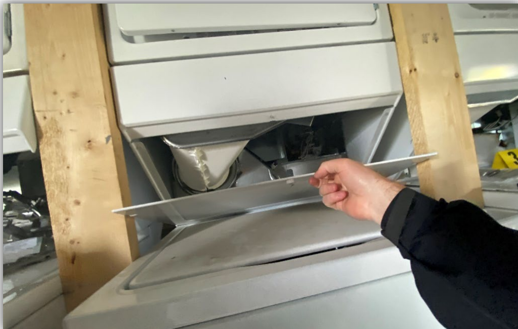
Image 7 – Inspection panel for access to dryer gas valve.
