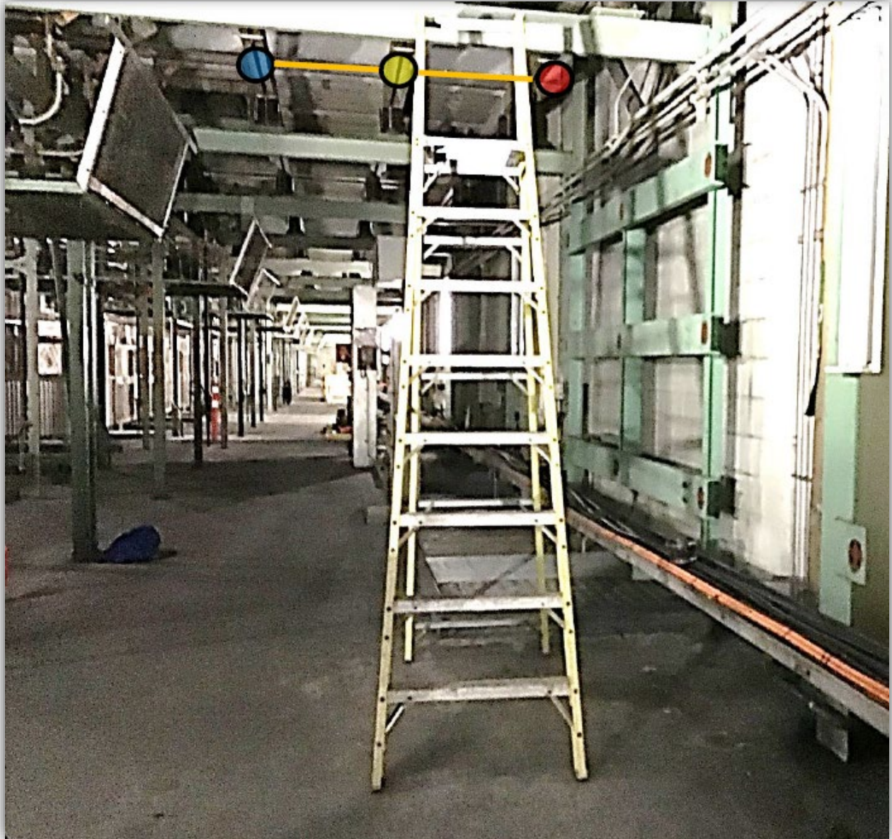
Photo 5 - General area of incident showing three phase high voltage bus bars (3 phase - 13,200/7620-volt) Phase colours shown for reference only.
