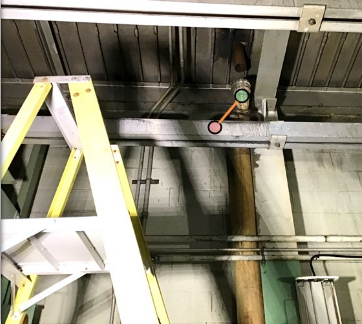
Photo 2 – High voltage bus bar, drainpipe, and ladder. The 7,620-volt shock occurred between one bus bar (RED) and the grounded metal drainpipe (GREEN).
