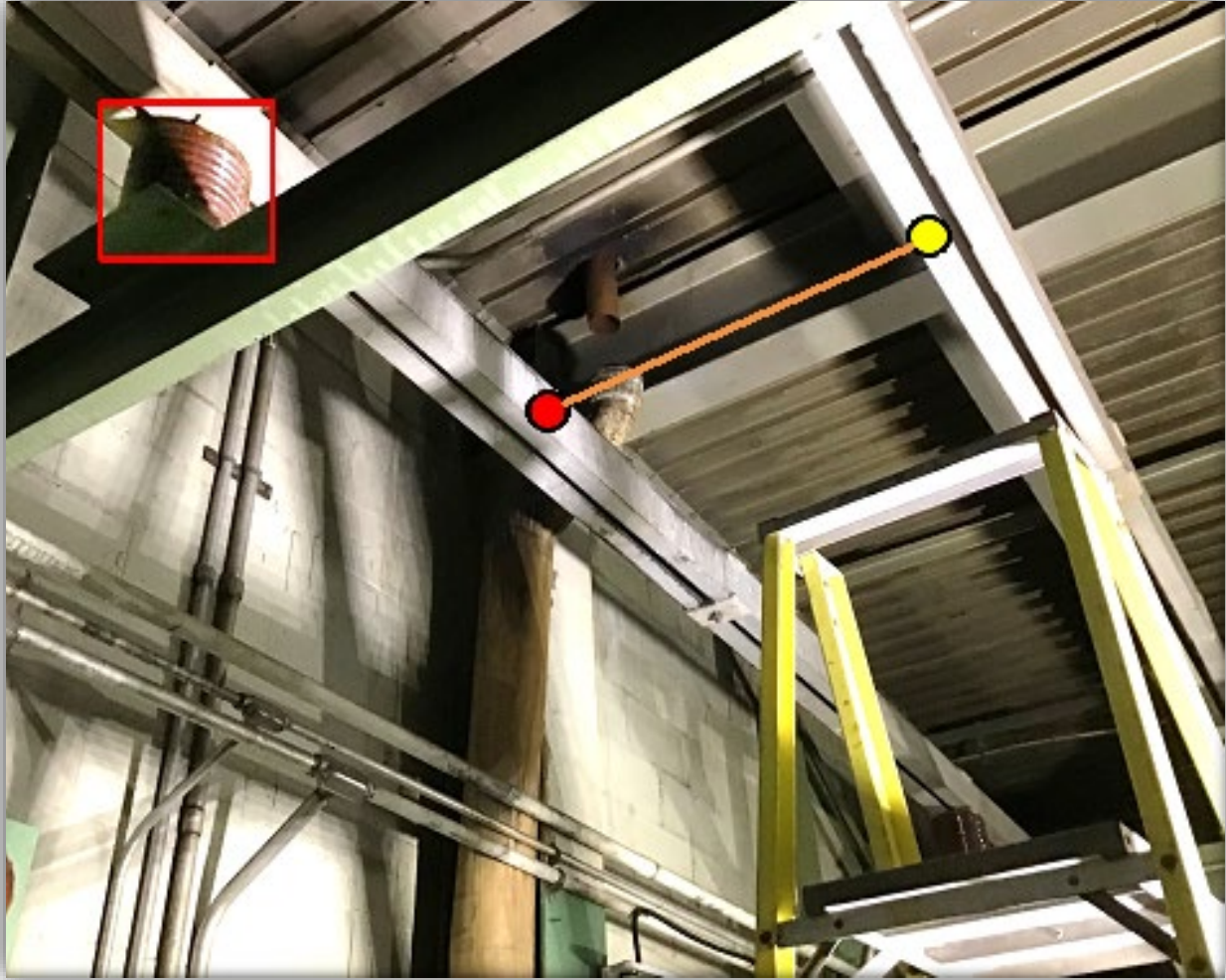
Photo 4 – (RED & YELLOW DOTS) High voltage bus bars and work area. There was 13,200-volts line to line voltage present. (RED BOX) Insulator.
