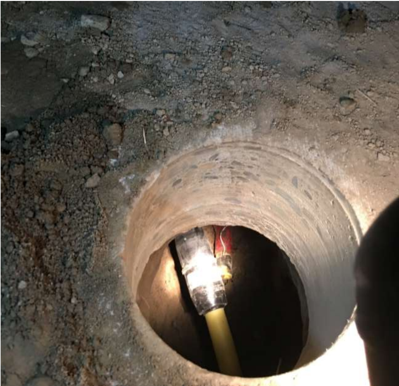
Capped gas line (Picture submitted by notifier)
