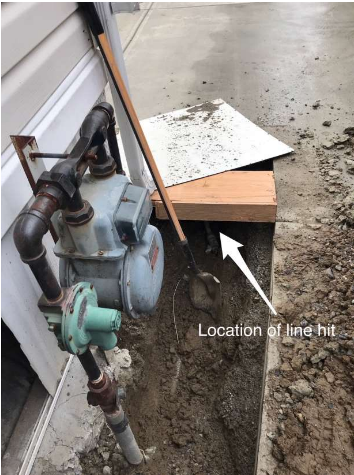
Propane gas meter and location of line hit.
