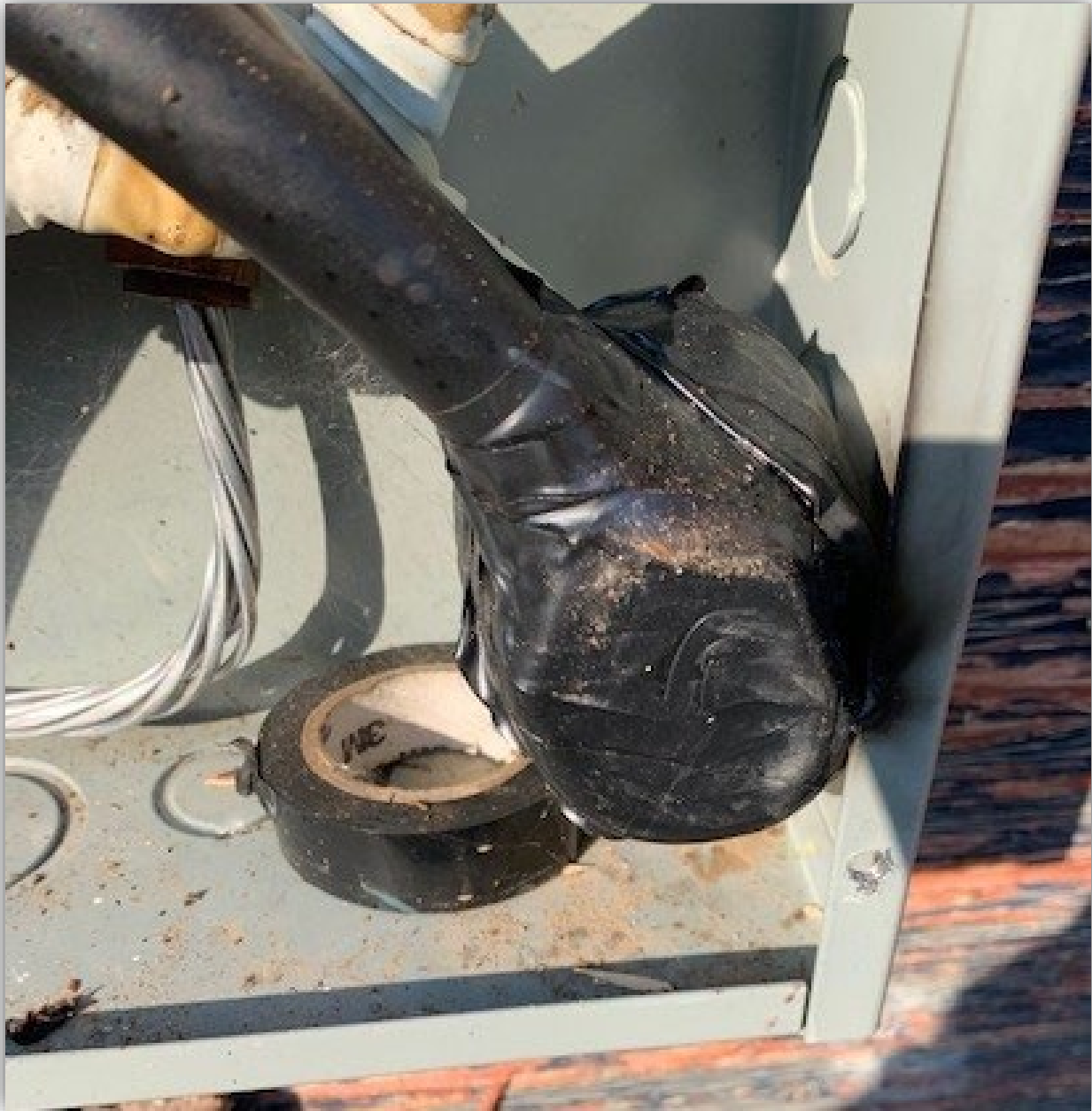
Image 2 - Split-bolt contact with equipment enclosure.
