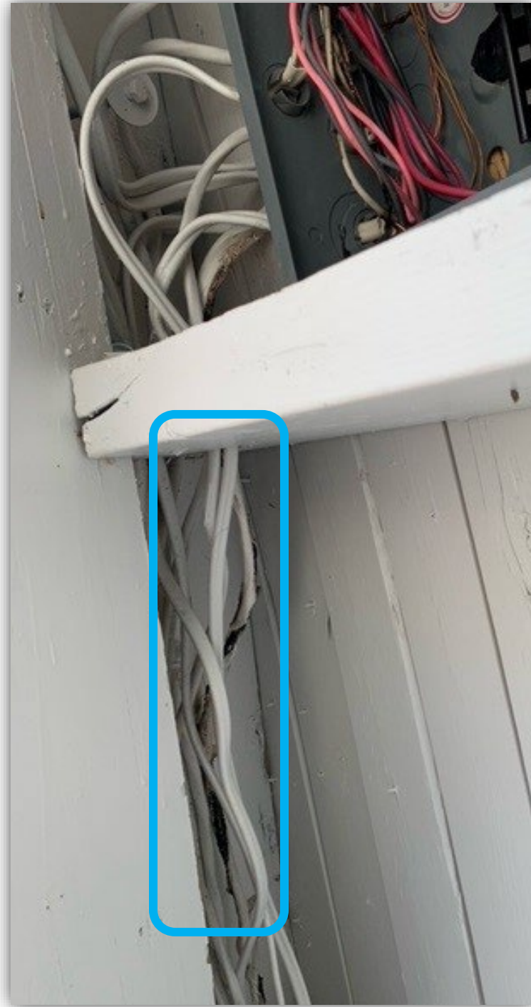
Image 5 – Overtemperature: Cable sheath discoloration resulting from excessive current imposed on neutral and bonding conductors.
