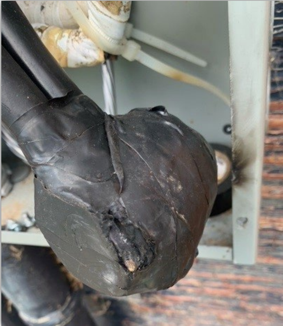
Image 1 – Deteriorated split-bolt insulation.
