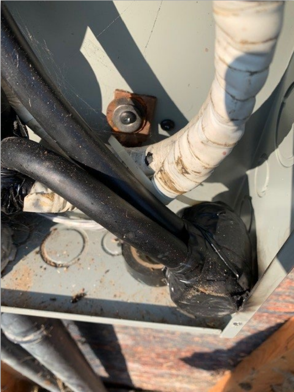
Image 3 - Unapproved equipment, unsafe wiring method, high impedance bonding termination.
