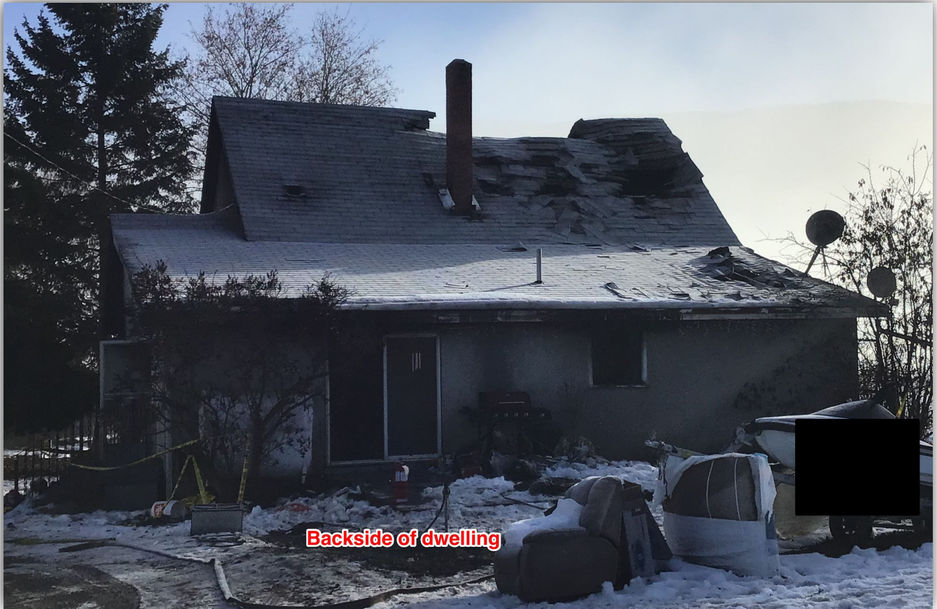
Photo 2 - Backside of dwelling from Northwest side, roof burnt through near South end upper floor.
