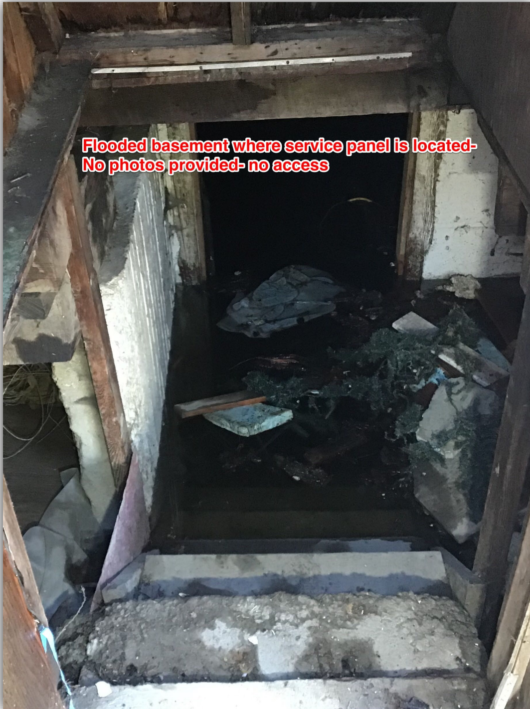
Photo 3 - Basement where service panel was located - no access or photos to review, access is from exterior only. Entry from exterior was flooded, with no further information available.
