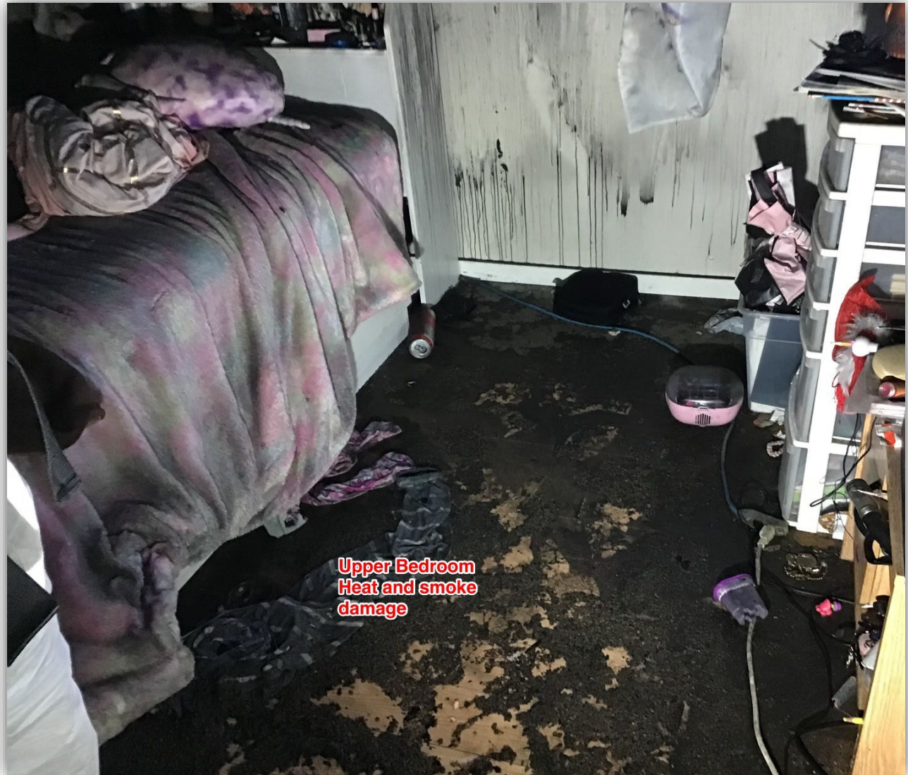
Photo 9 - Upper bedroom floor; North bedroom, with heat and smoke damage.
