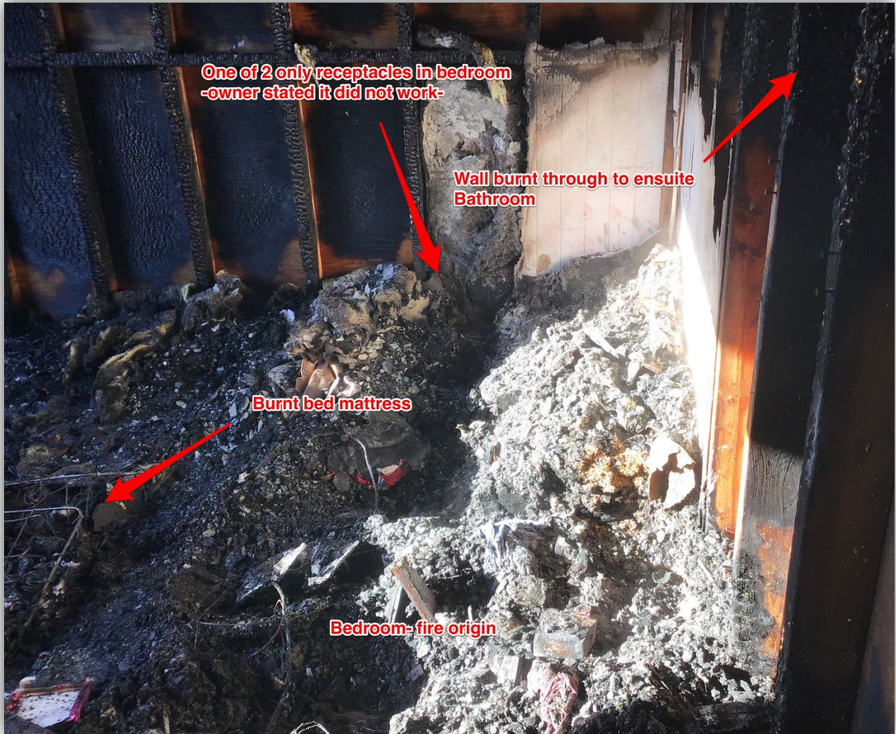
Photo 6 – Origin of fire: Bedroom. Lower area studs with surface charring and the upper section of studs provide deep charring from fire within room. One receptacle (1 of 2 only in room) near back wall was noted as not operational prior to fire. The TV, gaming console and space heater were buried in the debris.
