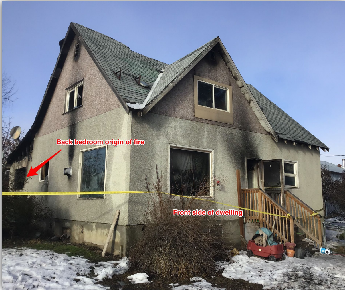
Photo 1 - Front side of dwelling from Southeast direction showing smoke only damage at front with windows intact.
