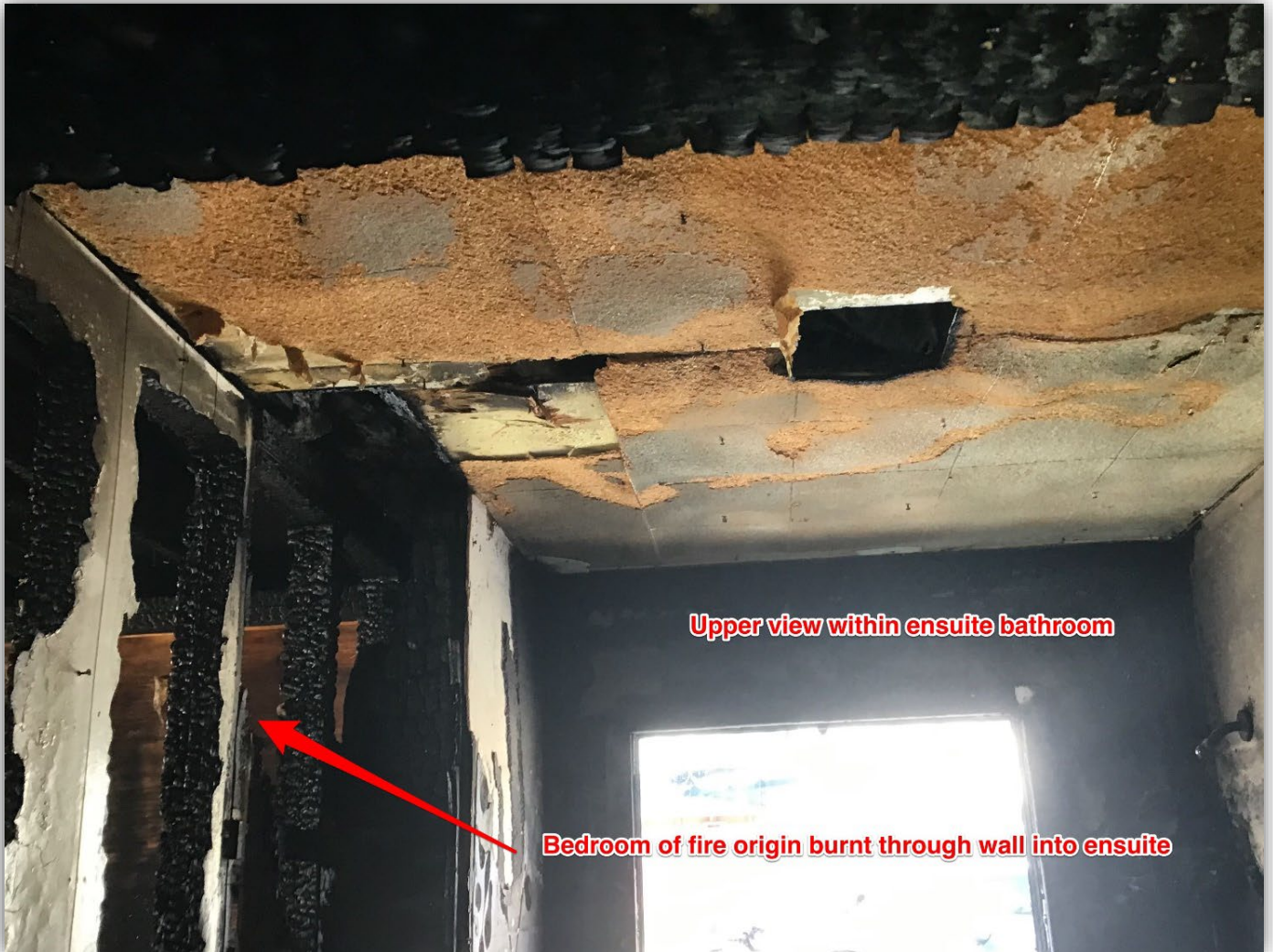
Photo 5 - Upper area within bathroom with heat/smoke damage as well as wall burnt through from bedroom area on left. The bedroom was fully involved during fire.
