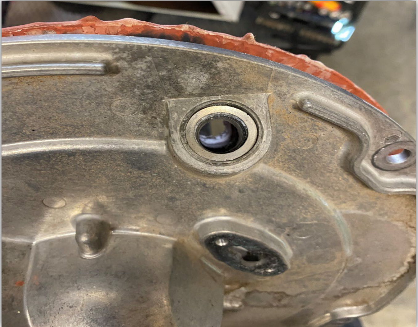
Image 3 - Broken sight glass located in the lid of the heat exchanger and damaged lid.
