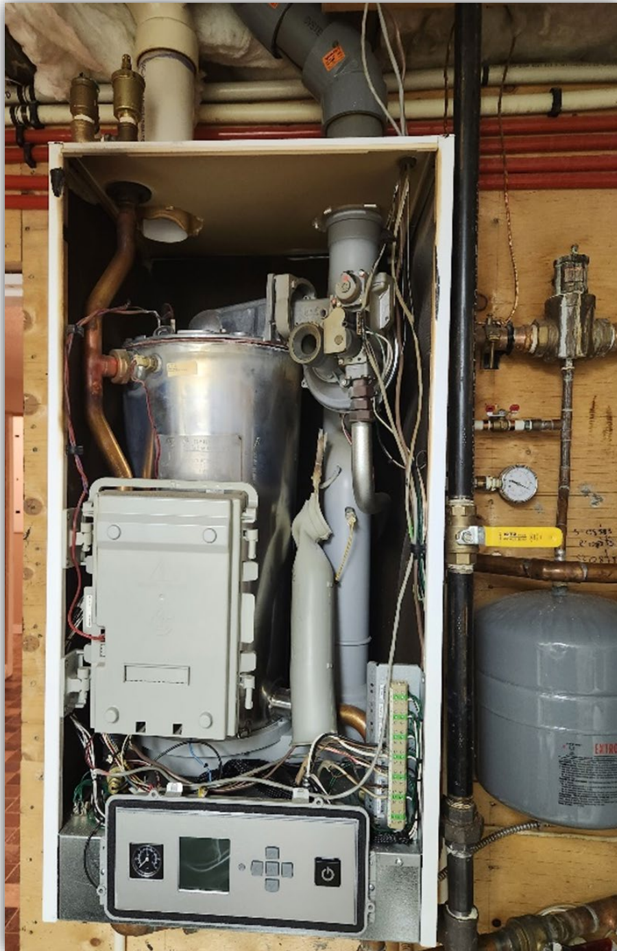
Image 1 – Boiler with the front cover removed.
