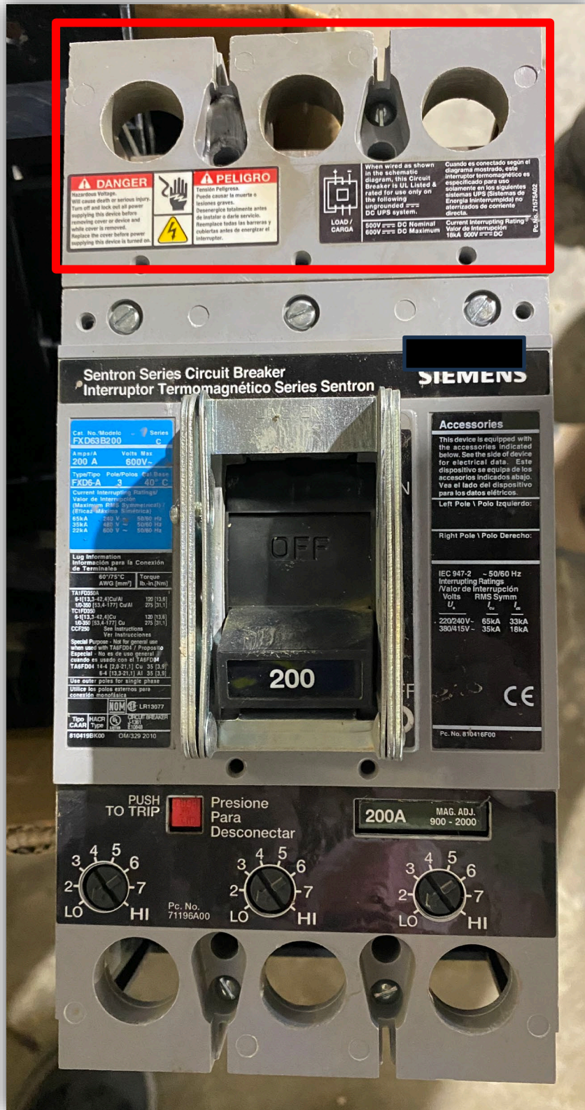
Image 5 - Main breaker that was previously installed in the electrical panel where the fault occurred. A light brown colour can be seen in this area where the fault occurred.
