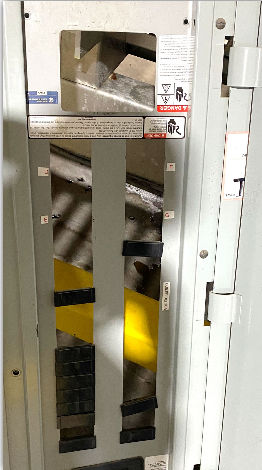
Image 3 - Cover of electrical panel showing signs of charring on panel at location of the fault.
