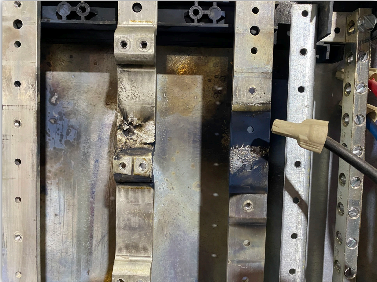
Image 2 - Bus bars of electrical panel showing charring and melting of electrical bus.
