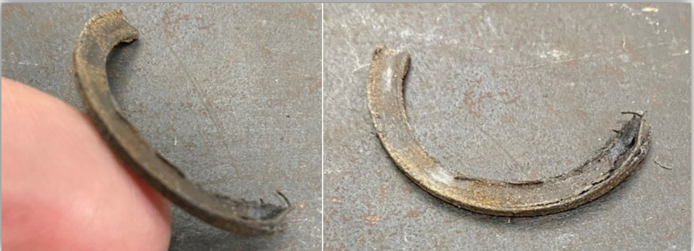
Photo 7 - Two pieces of the damaged flange gasket from the location of the leak.
