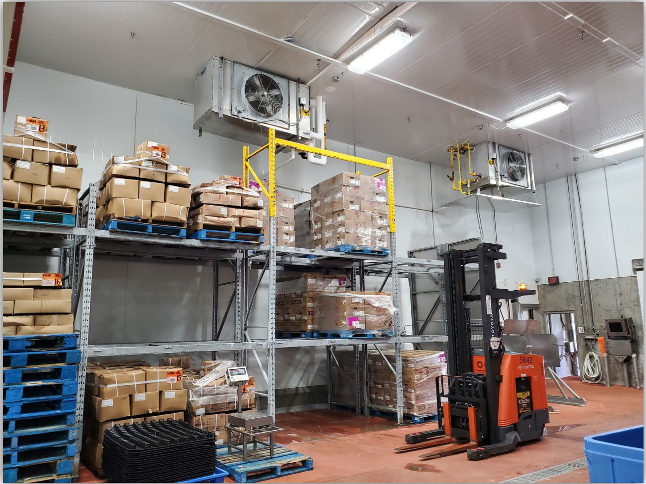
Photo 2 – Refrigerated food receiving area with racks of stacked food pallets, refrigeration condensers, and forklift.
