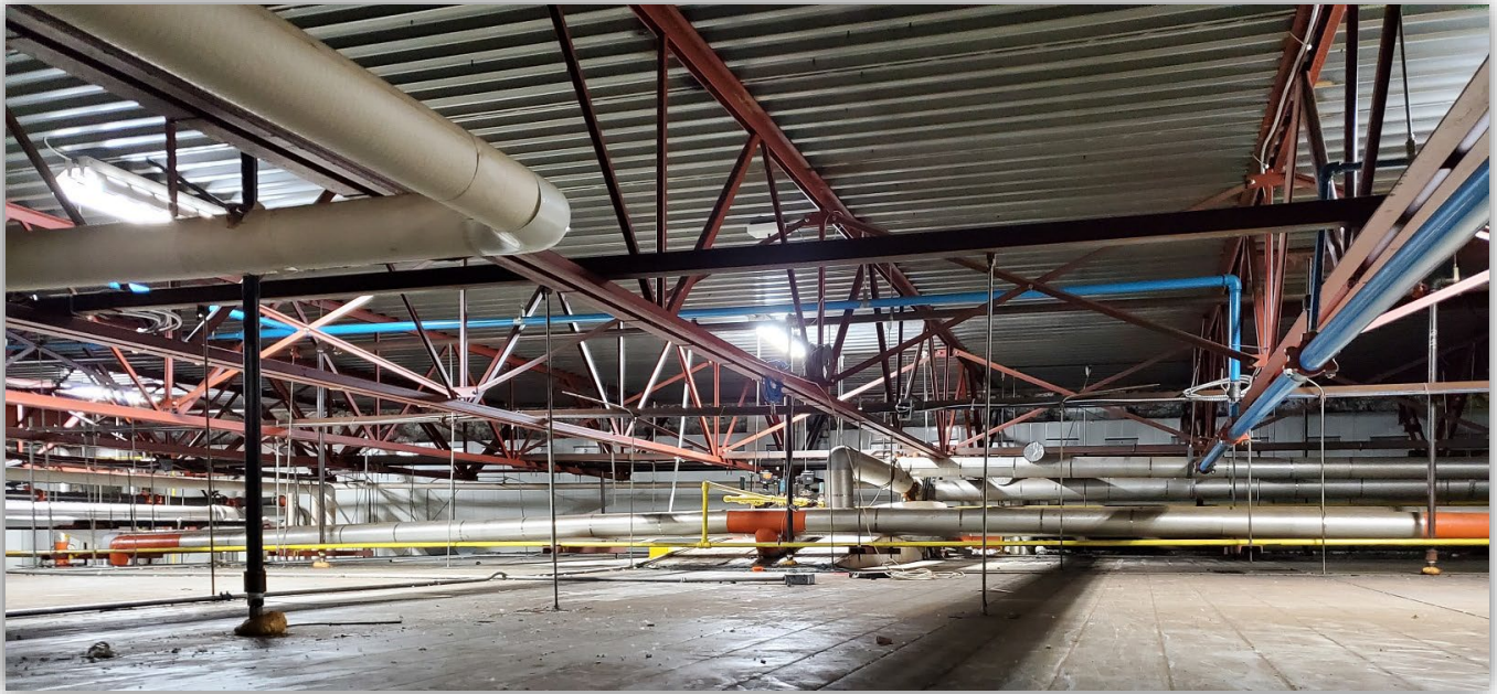
Photo 4 – Mezzanine area above refrigerated food receiving area showing refrigeration piping suspended above insulated panels.
