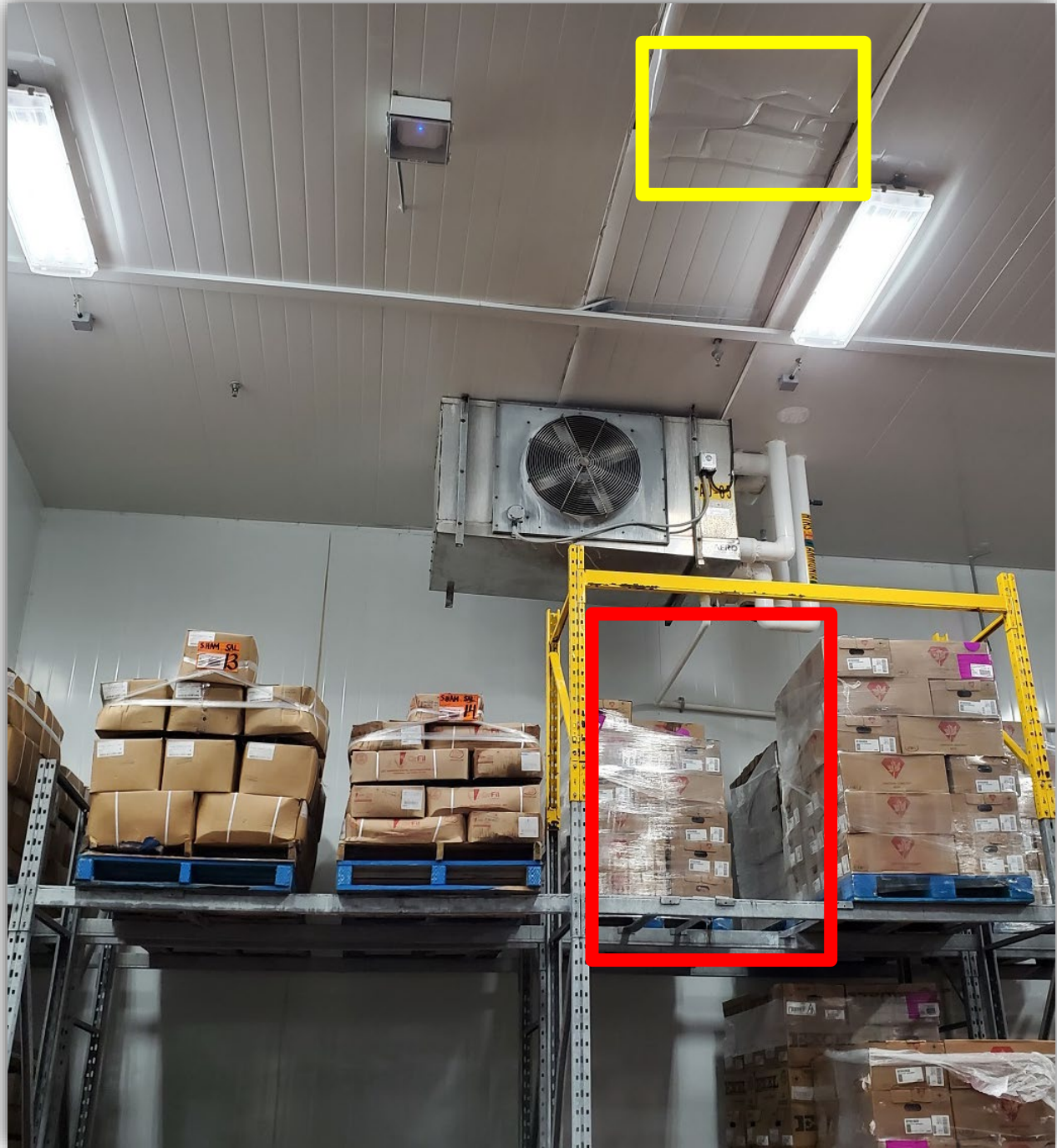
Photo 3 – [RED] Area food pallet was moved from. [YELLOW] Area forklift contacted ceiling.
