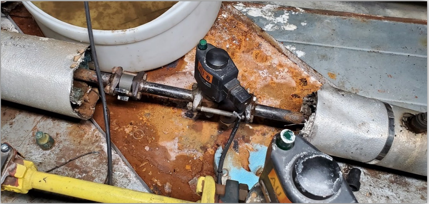
Photo 6 – Closeup of ammonia lines at the location on the leak. Ammonia line with two-bolt flanged connections with sealing gaskets.
