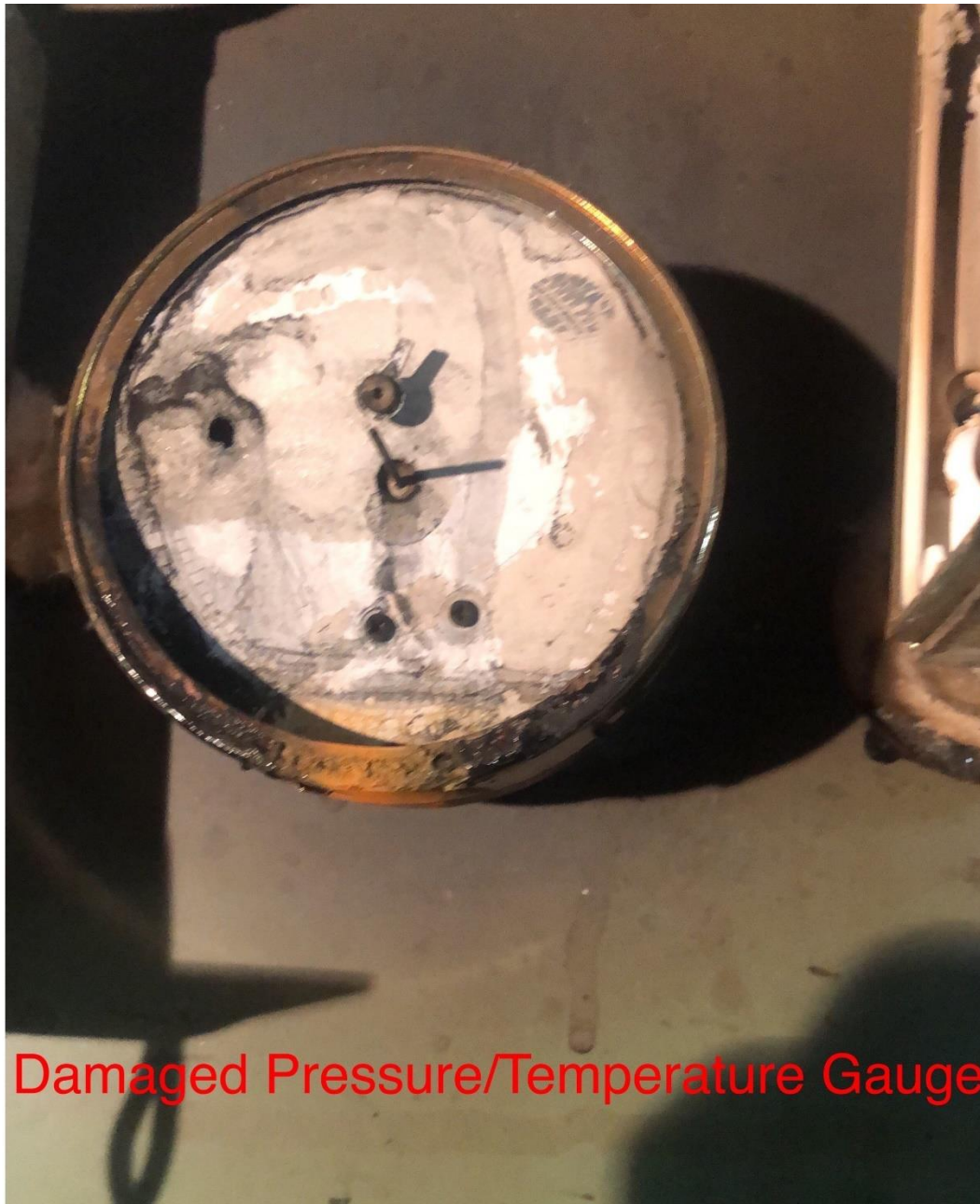
Image 4: Damaged Pressure Gauge
