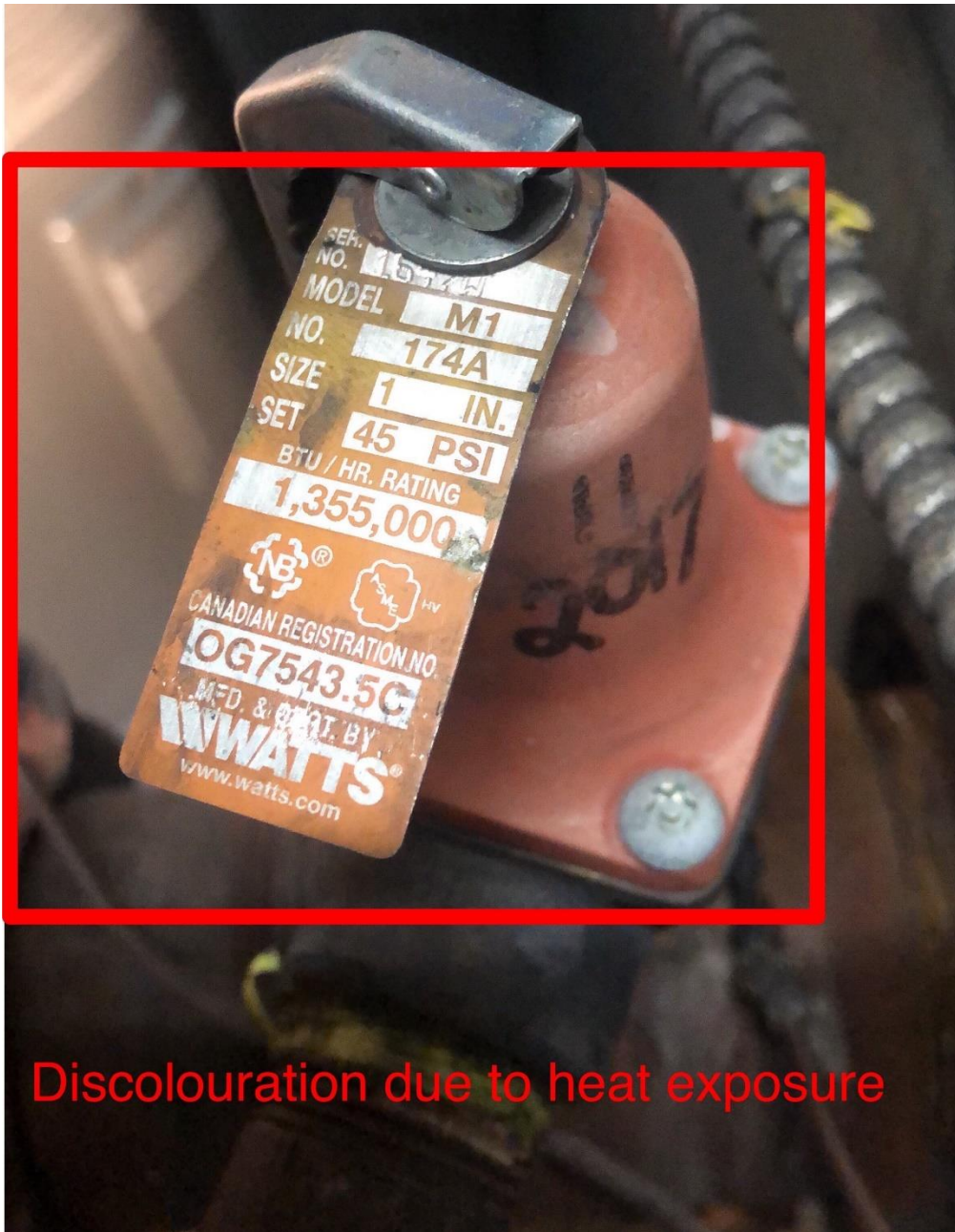
Image 6: Damaged Safety Relief Valve
