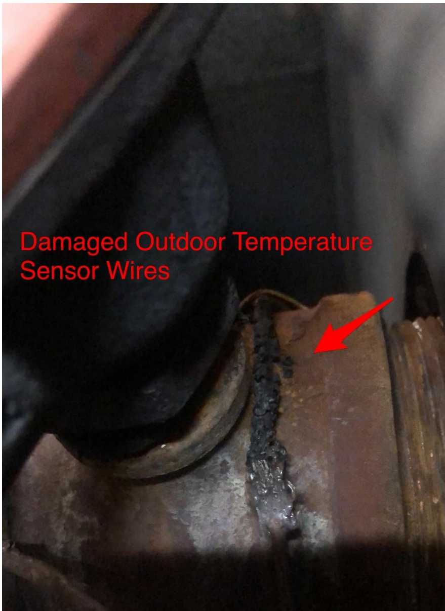
Image 7: Damaged Outdoor Temperature Wires at base of Safety Relief Valve
