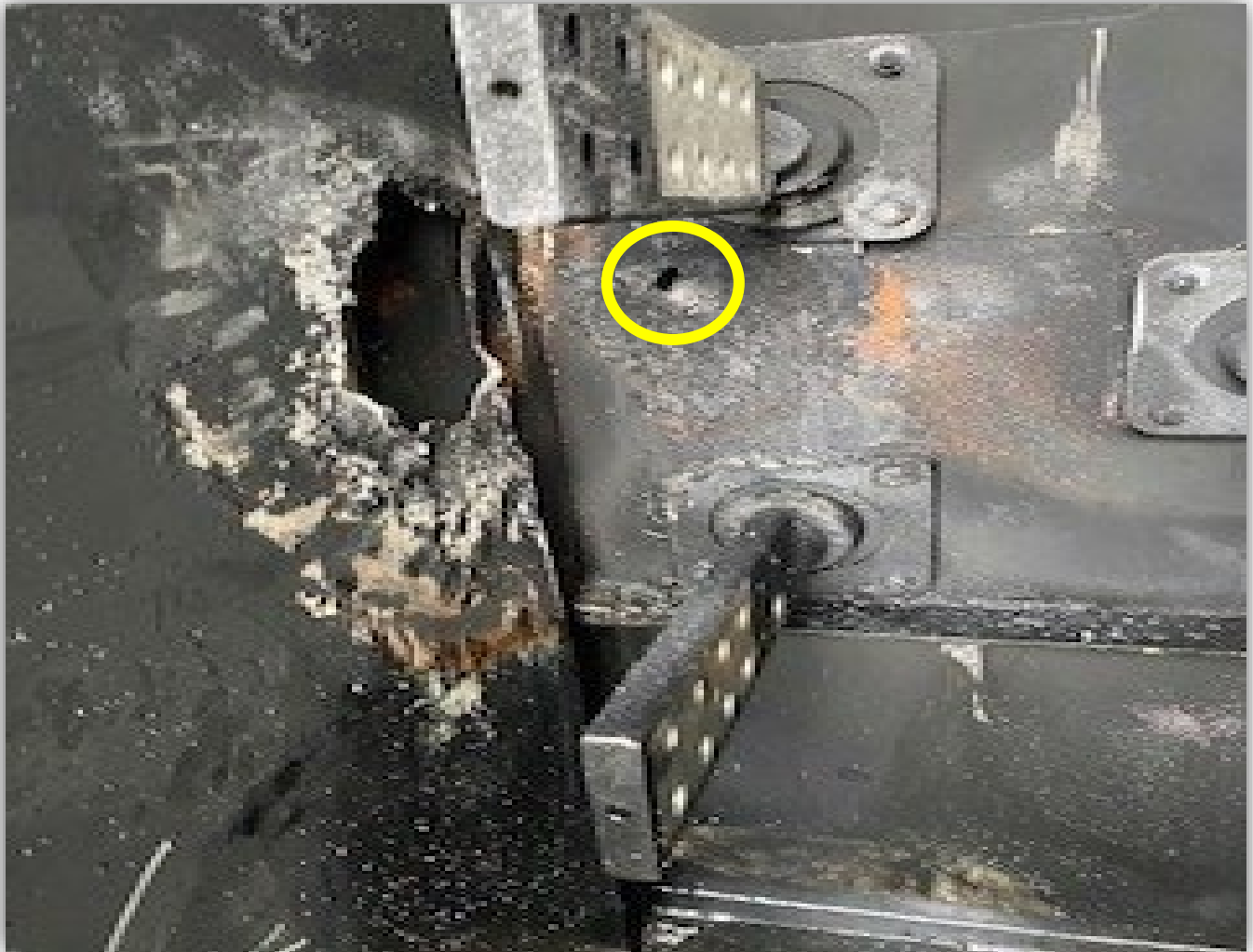
Image 4 - Possible initial fault location just past the “A” phase terminal block insulator and directly below where the bottom left bolt would have been if it had not melted off.
