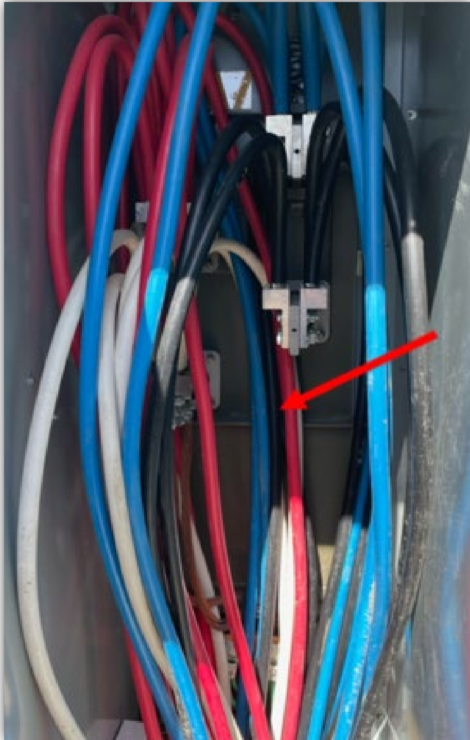
Image 2 - The route taken to install the two red phase conductors that were in close proximity to where the fault occurred (Provided by FSR).
