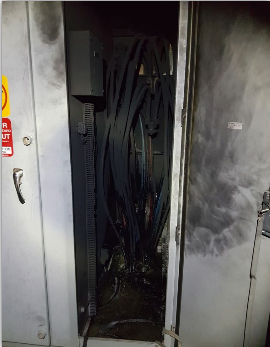
Image 5 - Secondary compartment at time of incident. Shows soot and damage from outside looking into transformers.
