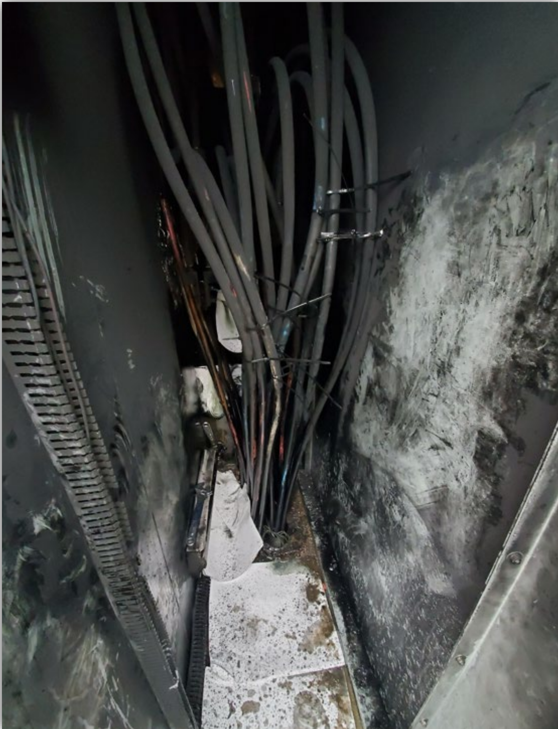
Image 6 – Interior of secondary compartment at time of incident.
