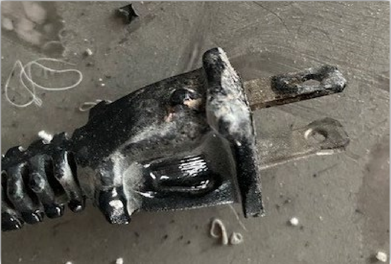
Image 3 - Portable heater plug-end showing charring on the line voltage prong, as well as localized melting of the plastic receptacle body around that prong.
