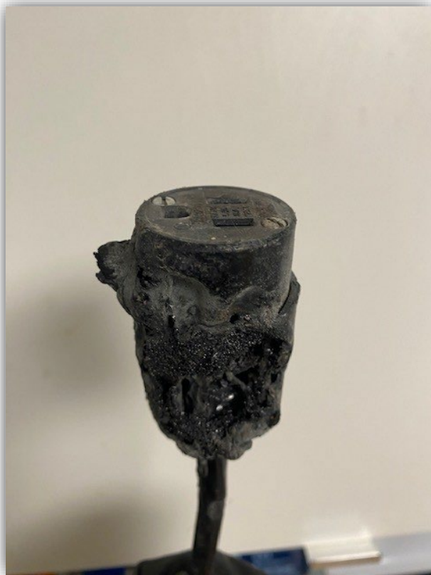
Image 6 - Melting around line voltage terminal.
