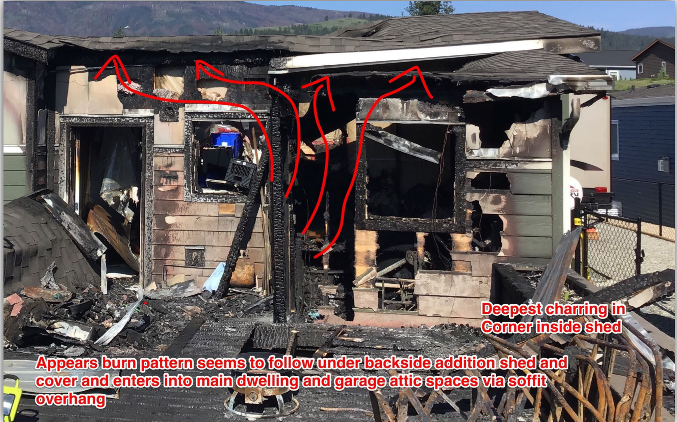
Image 4 - Lines provide proposed fire travel from shed location and access into garage and dwelling attic through soffit area.
