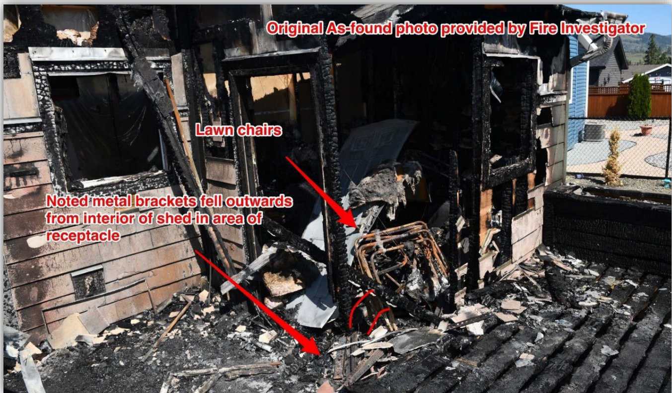
Image 1 - Original as-found on site prior to sifting through and removing electrical evidence on Monday May 15 (Image provided by Fire Investigator).
