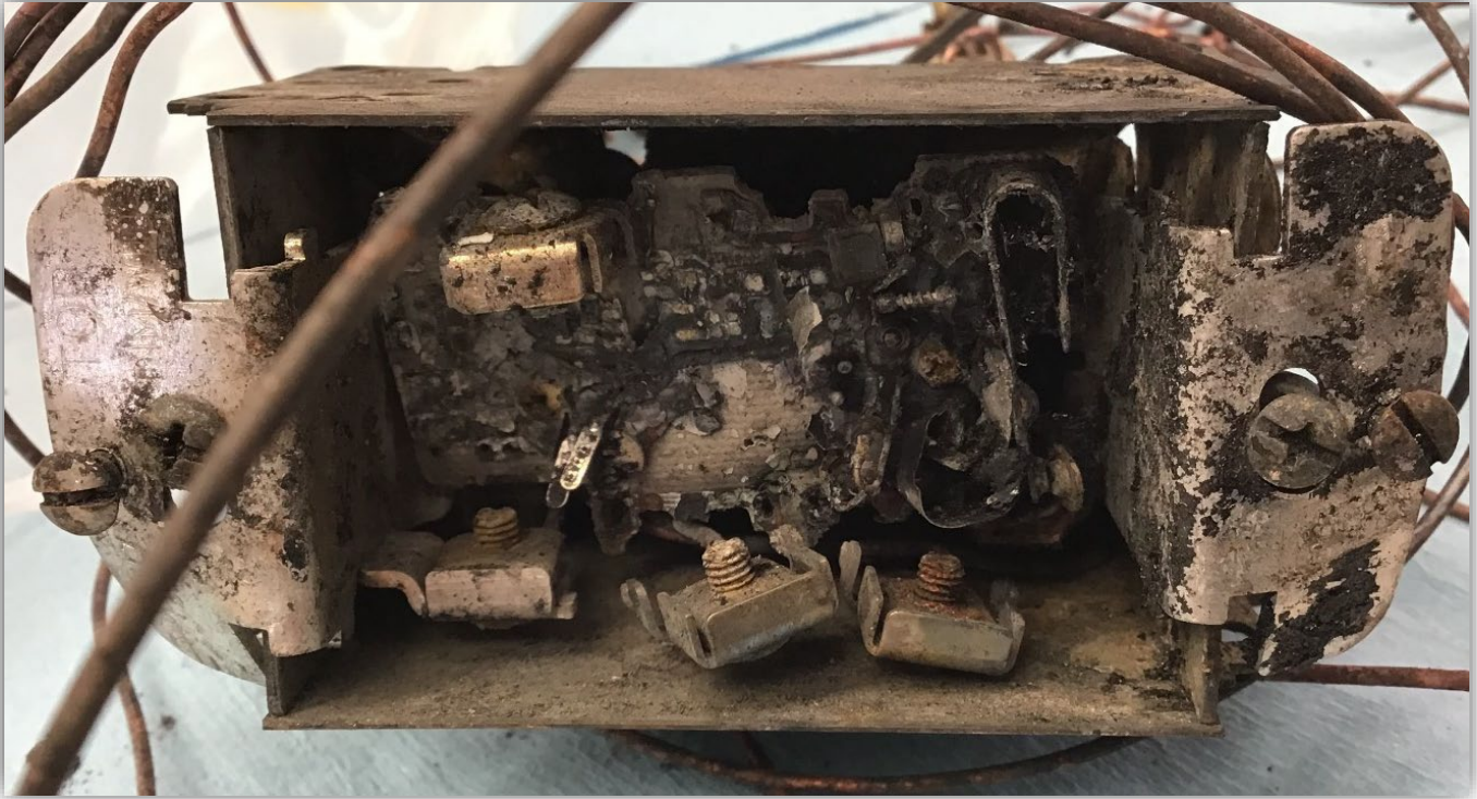
Image 11 - Damaged Dimmer switch- for reference only. Aluminum mounting bracket in one piece with no melting noted from extensive heat.
