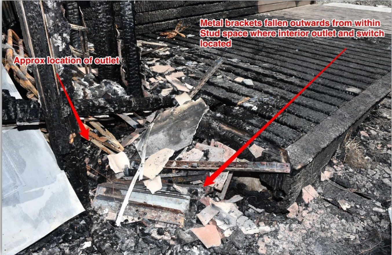
Image 2 – Site prior to Fire Investigator site review on Monday May 15 ( Image provided by Fire Investigator ).
