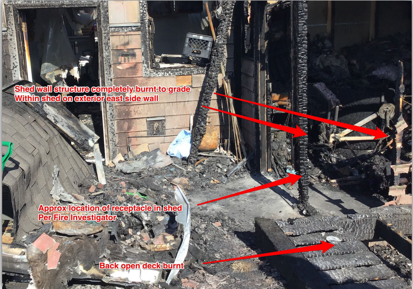
Image 5 - Back entry area: covered back open area roof laying on ground to left with shed location to right where most fire damage occurred. Extensive heat noted along upper wall area of garage and major fire damage to shed and wood decking.
