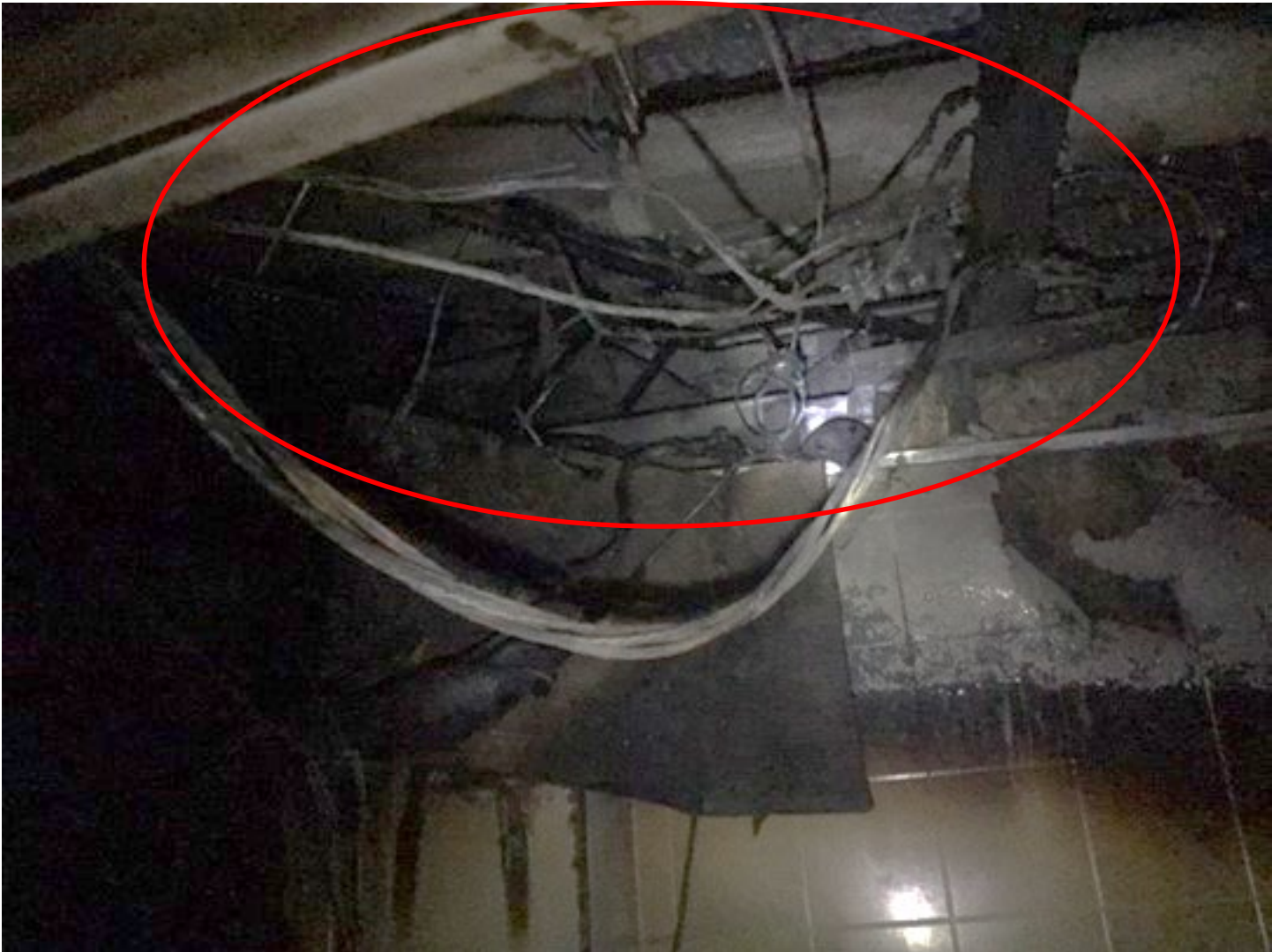
Area and main level floor joists above domestic hot water tank – fire and smoke damage.
