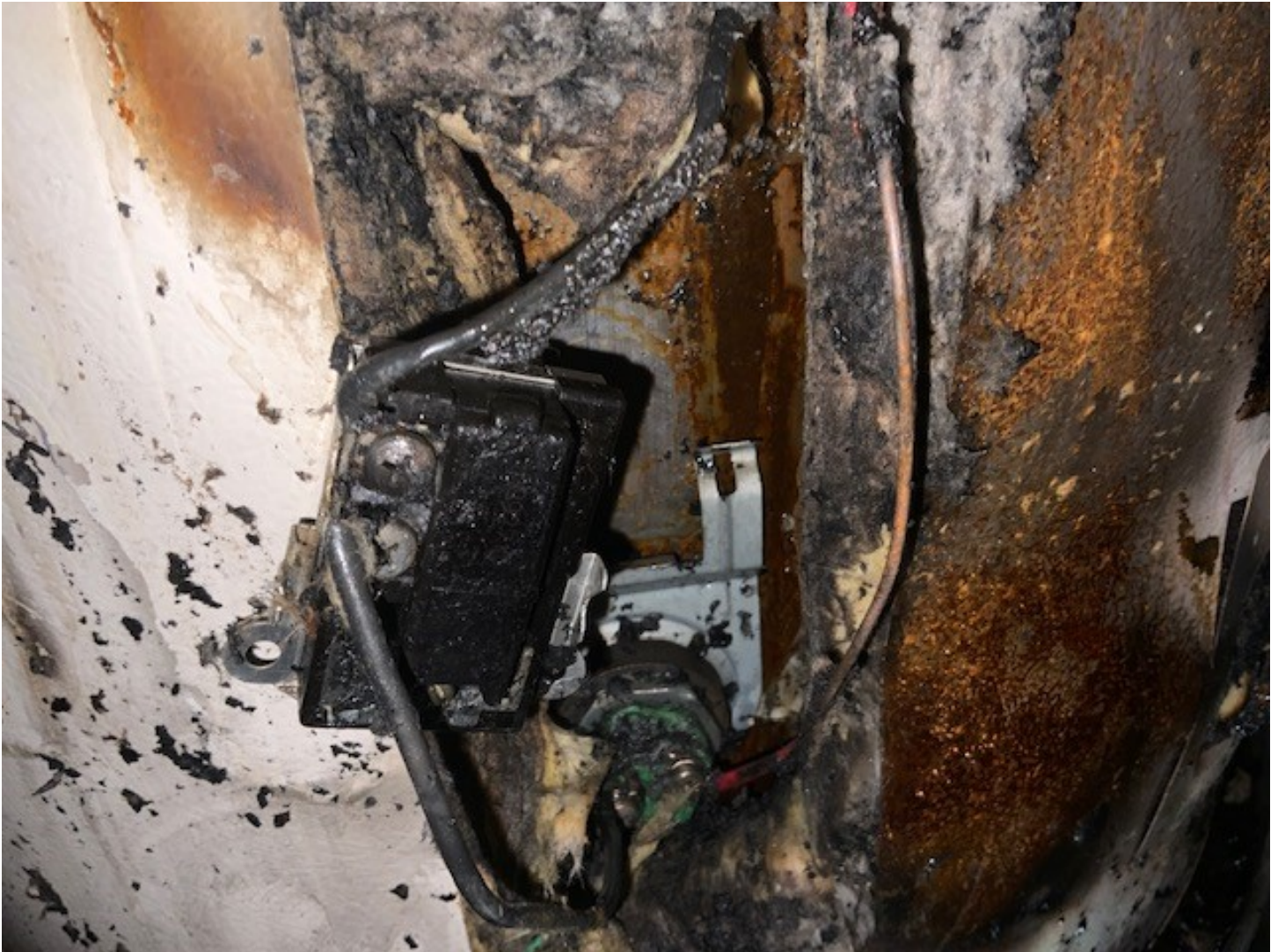
Photograph obtained by Regional Fire/Rescue – upper element and thermostat as found during fire suppression, cover previously removed.
