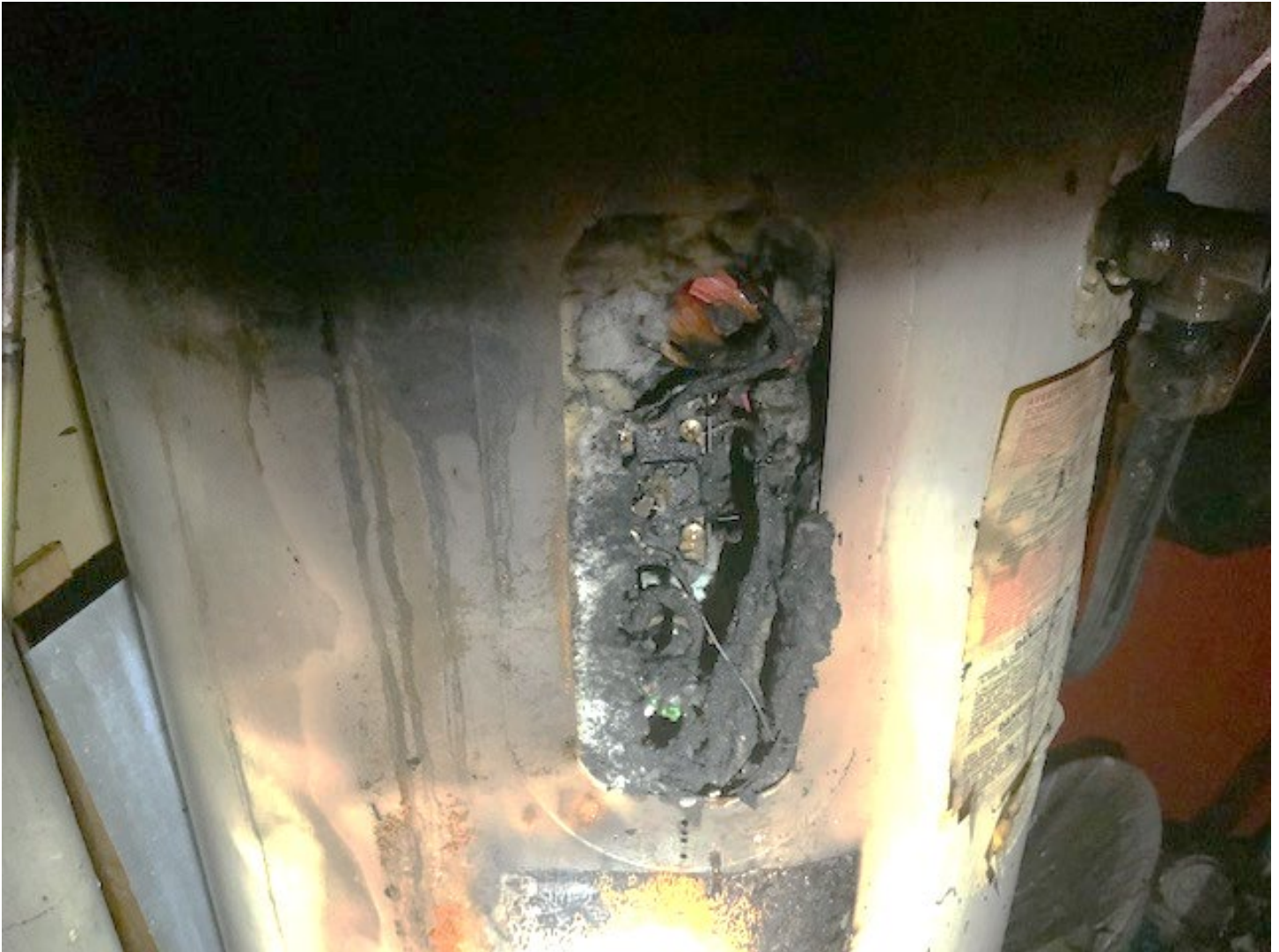
Photograph obtained by Regional Fire/Rescue – upper element and thermostat as found during fire suppression, cover previously removed.
