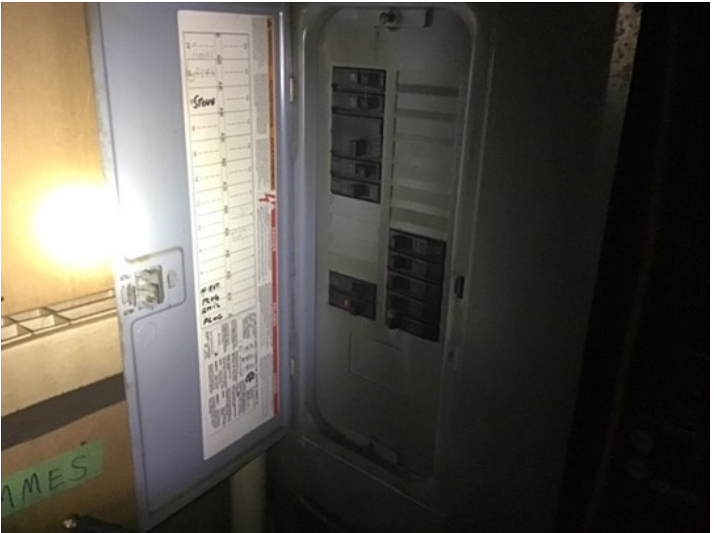
Dwelling subdistribution – 100A 120/240V panel board, located adjacent to domestic hot water tank.
