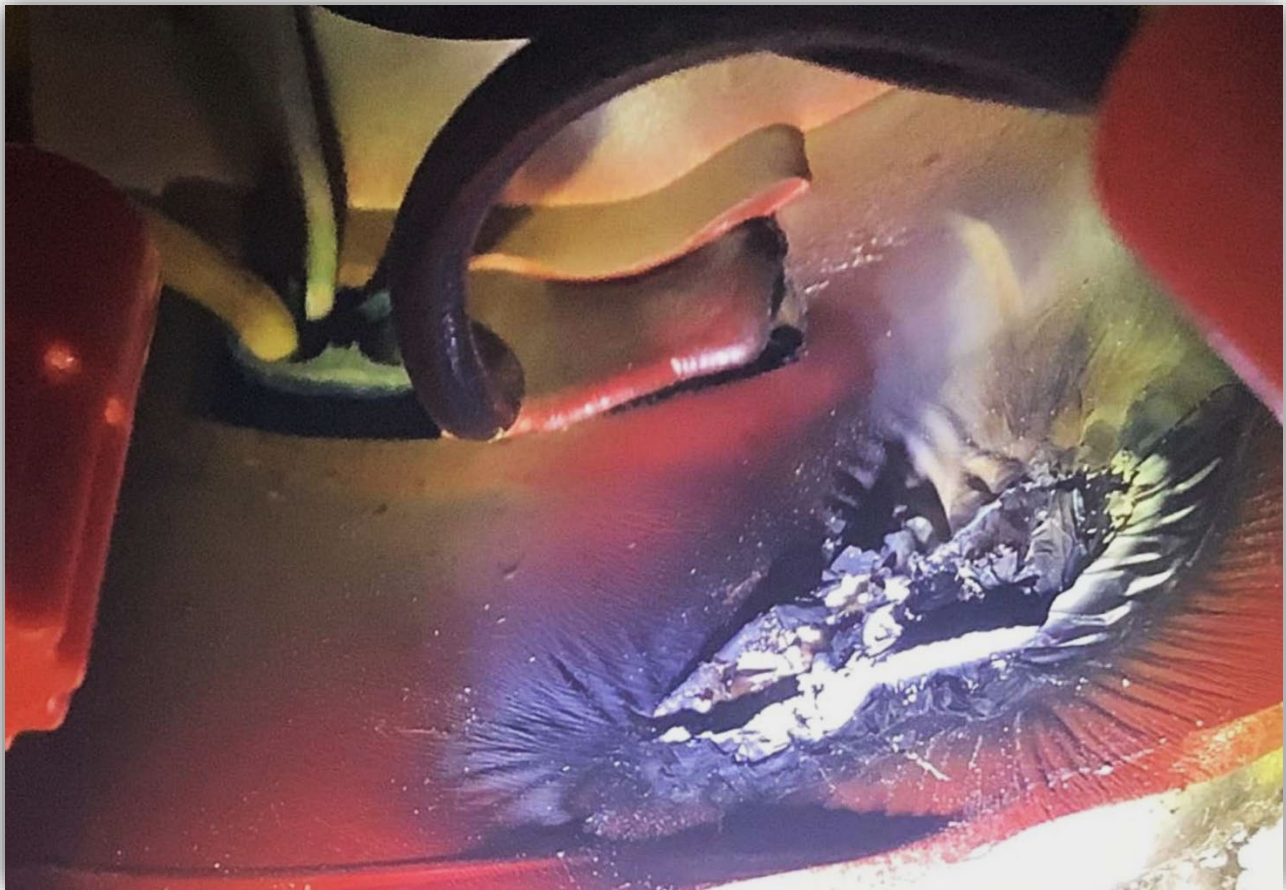
Image 4 - Damage to the smoke alarm outlet box.
