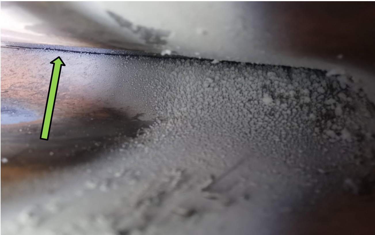
Picture 2 - Looking up into the heat exchanger a crack can be seen.
