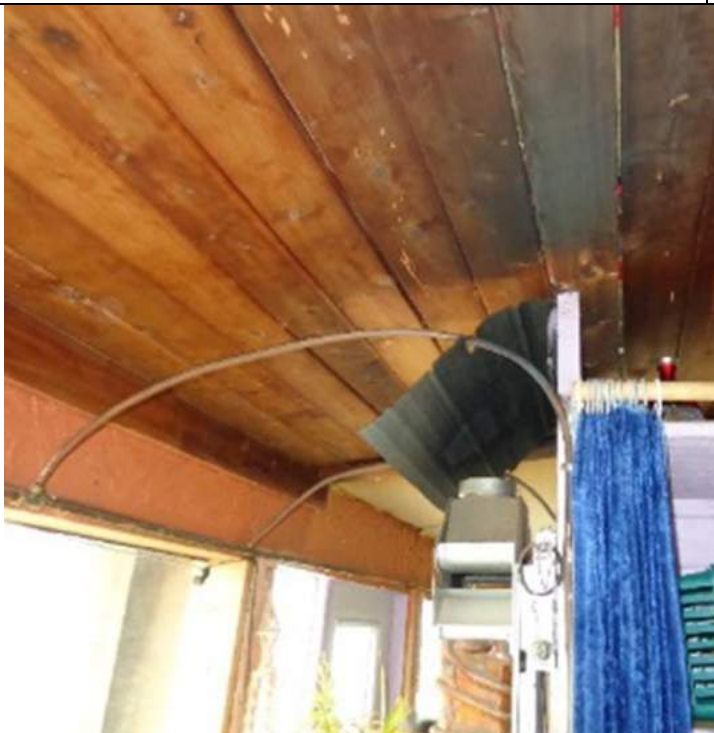
Vent outlet of water heater note soot on ceiling
