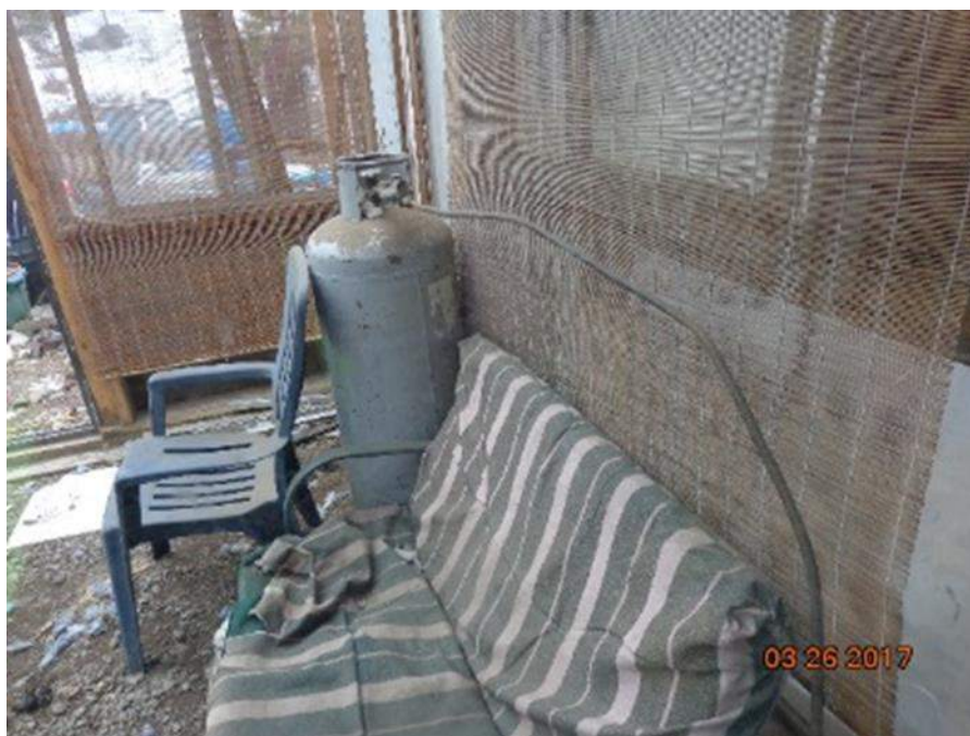
100 pound propane tank attached to water heater
