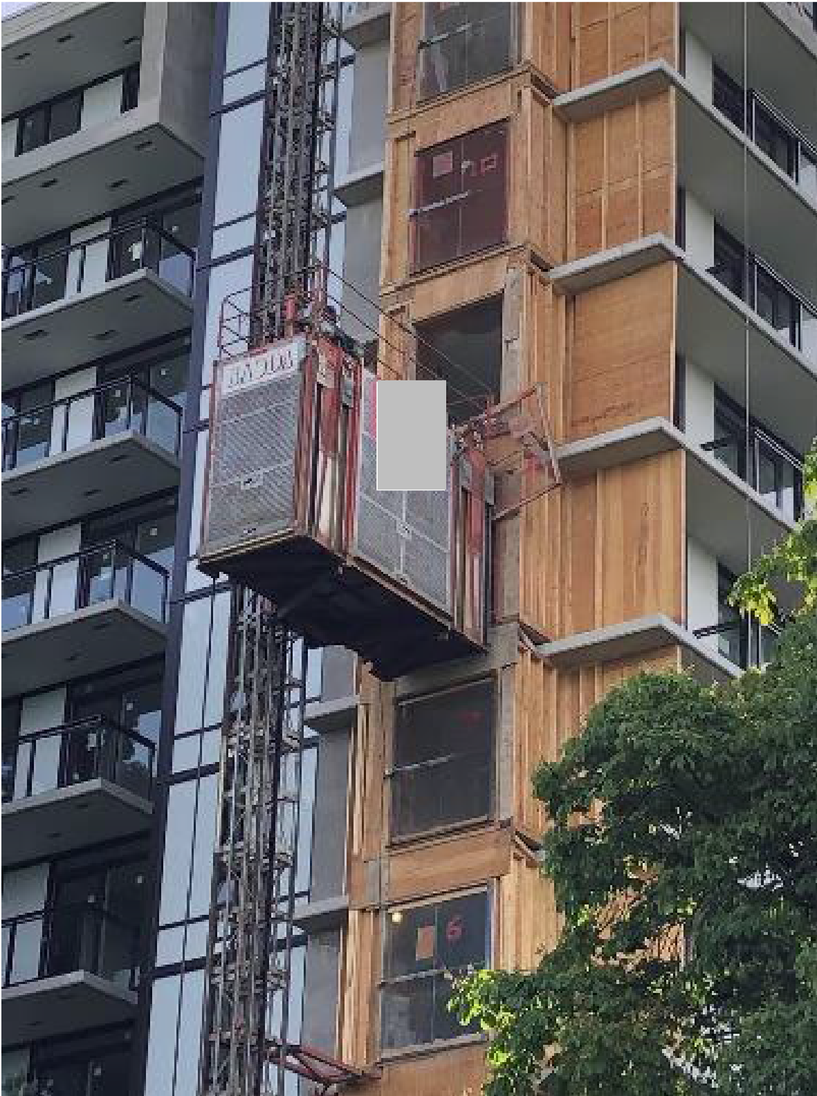
Gate dislodged from hoarding
