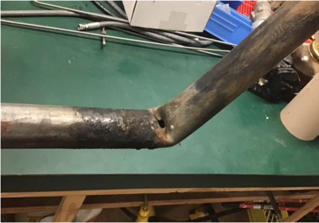
Photo 2: Mast pipe bend area. Hole created by electrical arcing event which would result in molten metal projecting from bend area and igniting adjacent combustible materials.
