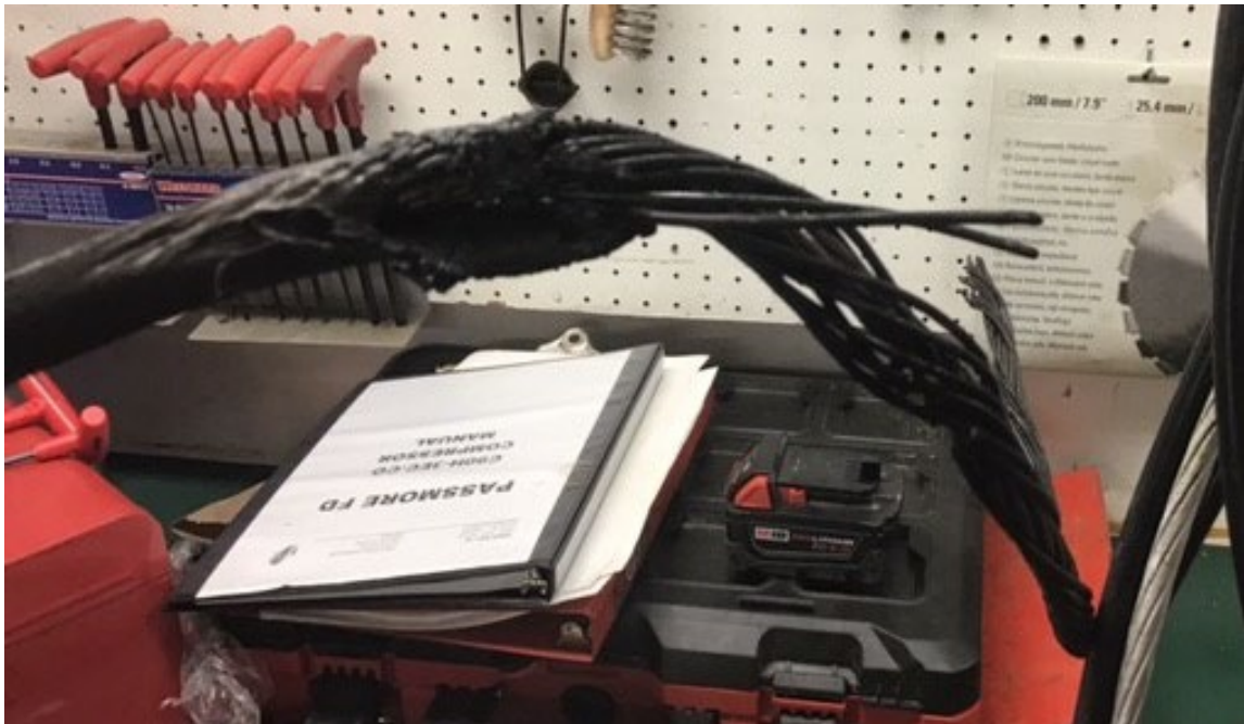
Photo 4: Ungrounded service conductor #2 area of electrical fault when withdrawn from mast pipe
