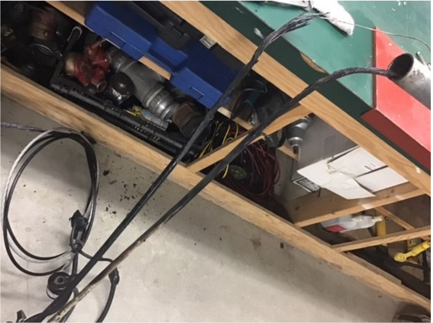
Photo 5: Service conductor withdrawn from mast pipe
