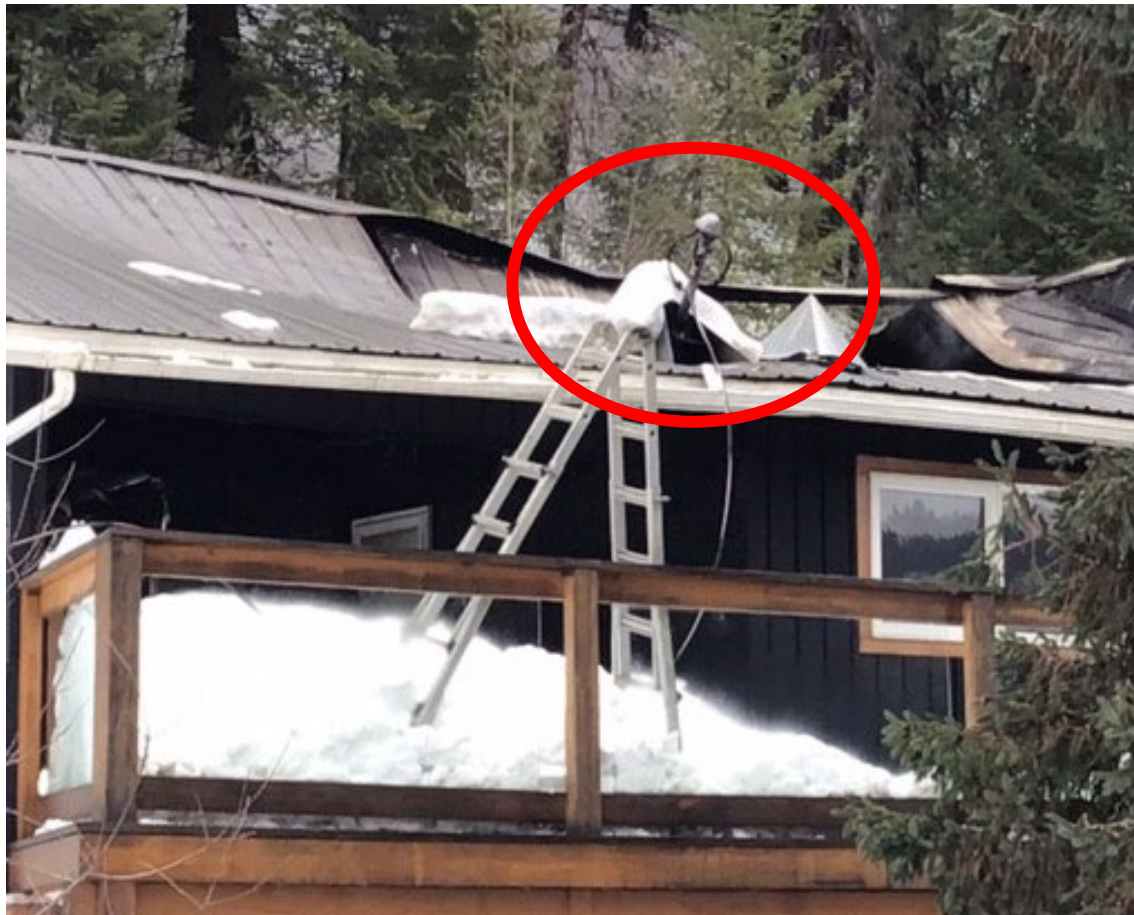
Photo 1: West side of structure revealing roof structure fire damage and bend electrical service mast pipe
