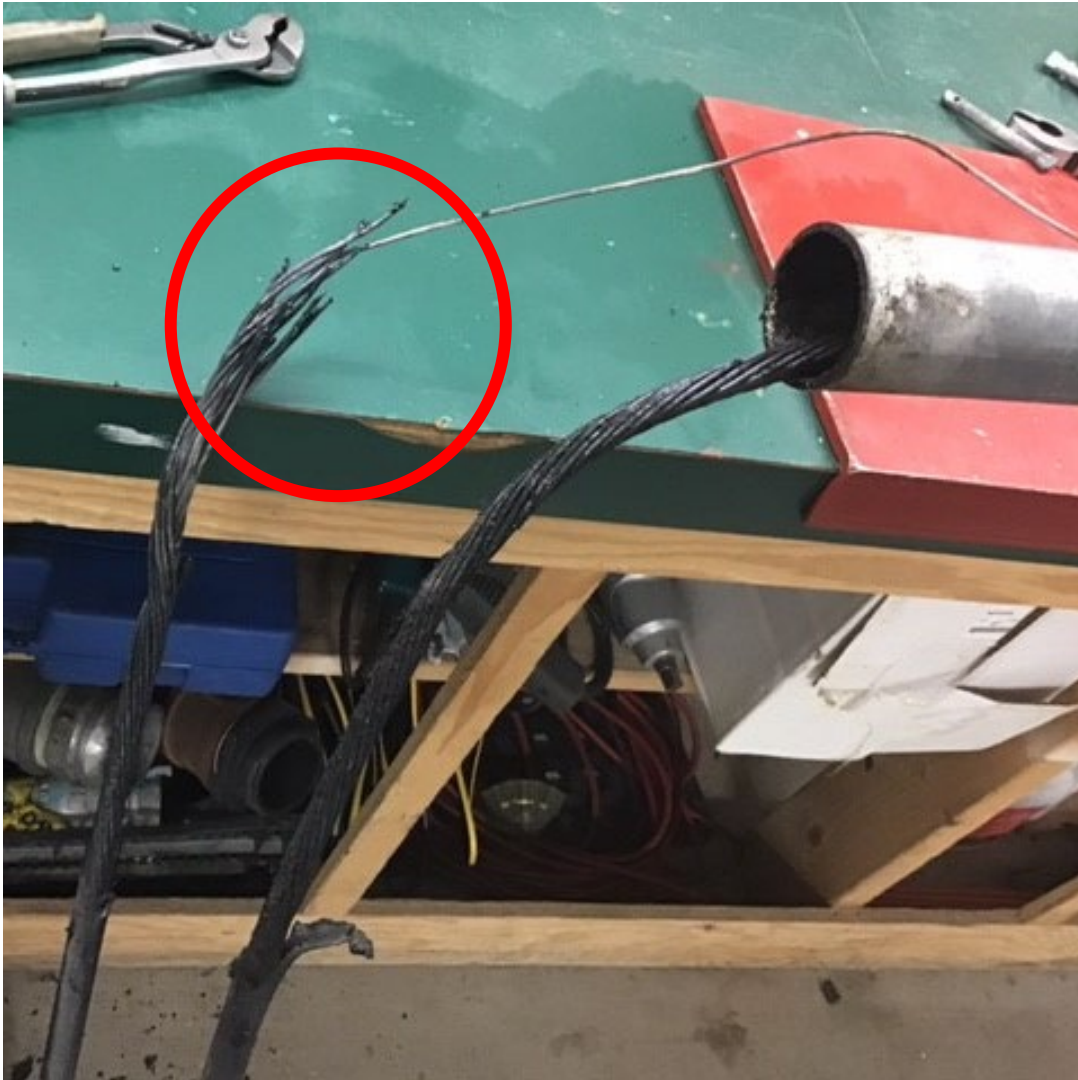
Photo 3: Ungrounded service conductor #1 electrical fault area when withdrawn from mast pipe
