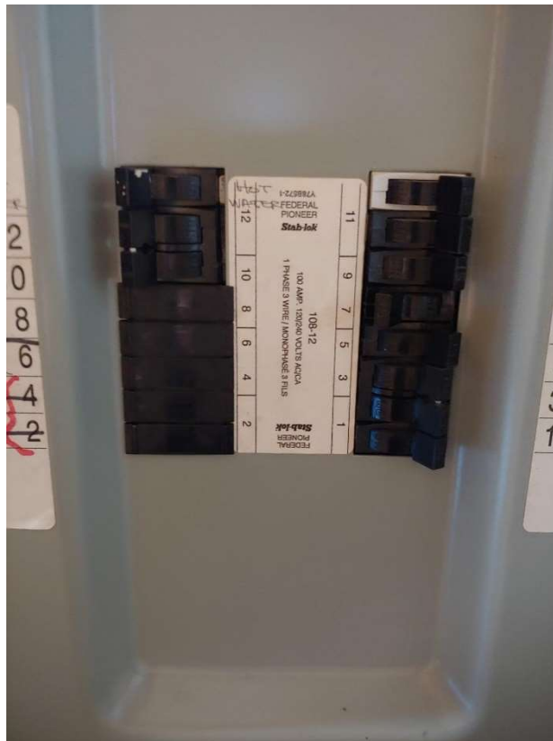
Federal Pioneer Distribution Panel with Breaker in off position.
