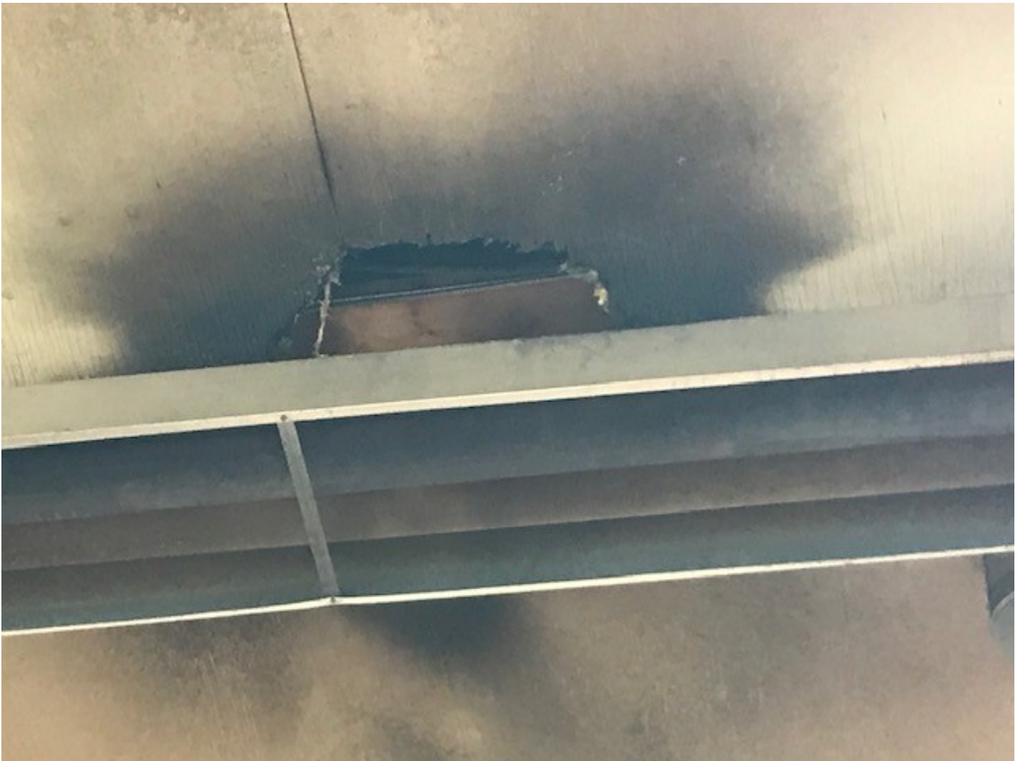
Overview Burnt ceiling
