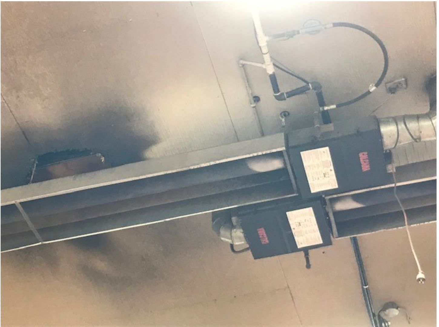
Heater in place, hole burnt through plywood ceiling
