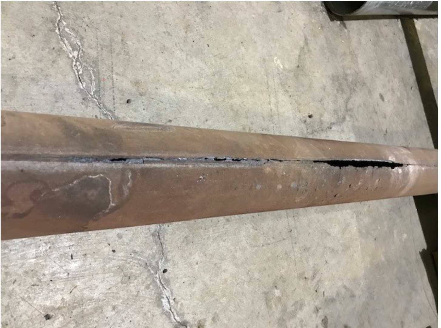
First section of heat tube, close up view
