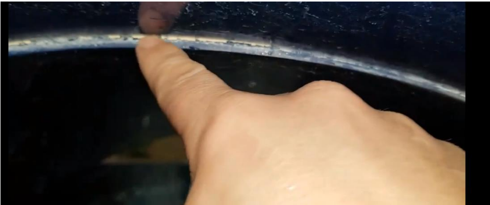
Photo 3: 1/4" protruding edge at flume connection
