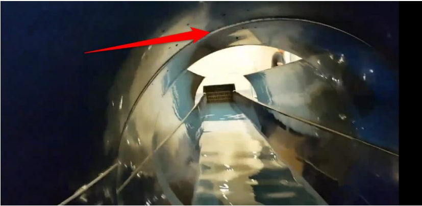
Photo 2: Misaligned flume connection prior to run out lane
