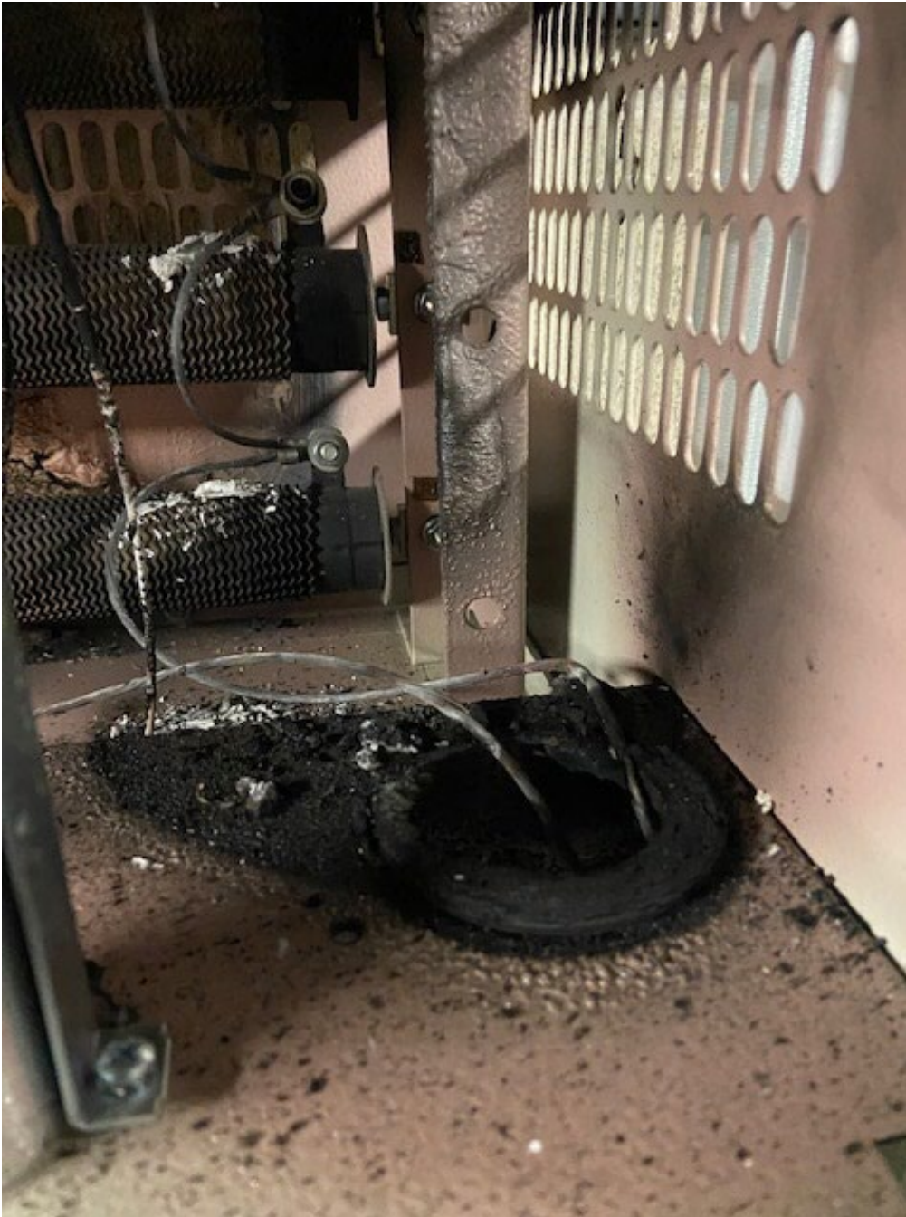
Image 6: Damage caused by heat
