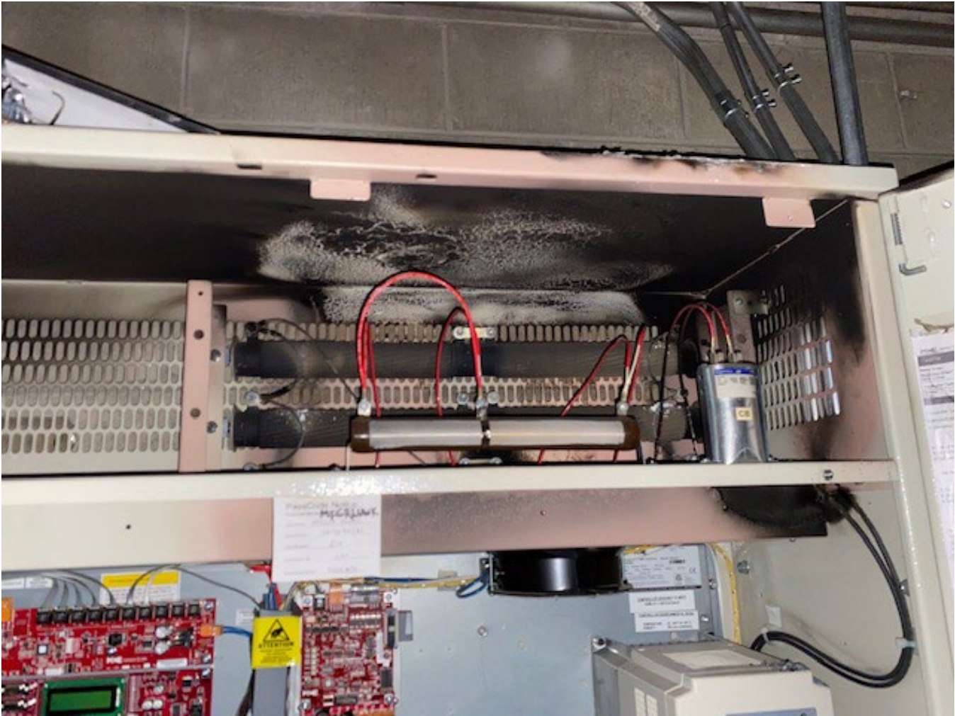
Image 5: Damage caused by heat
