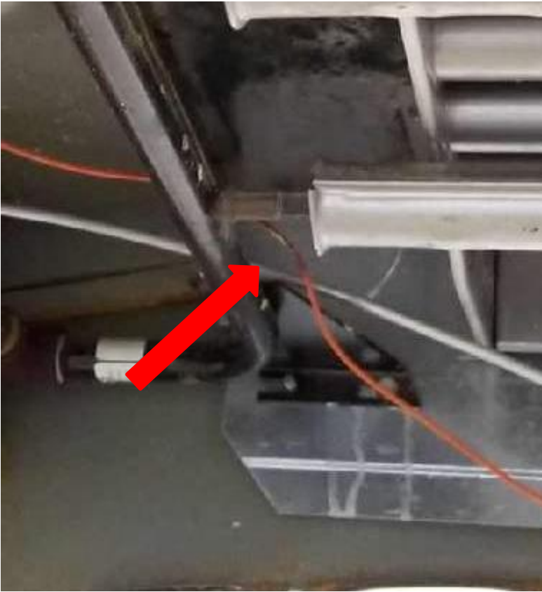
Figure 3. Close-up picture of burnt ignition wire.
