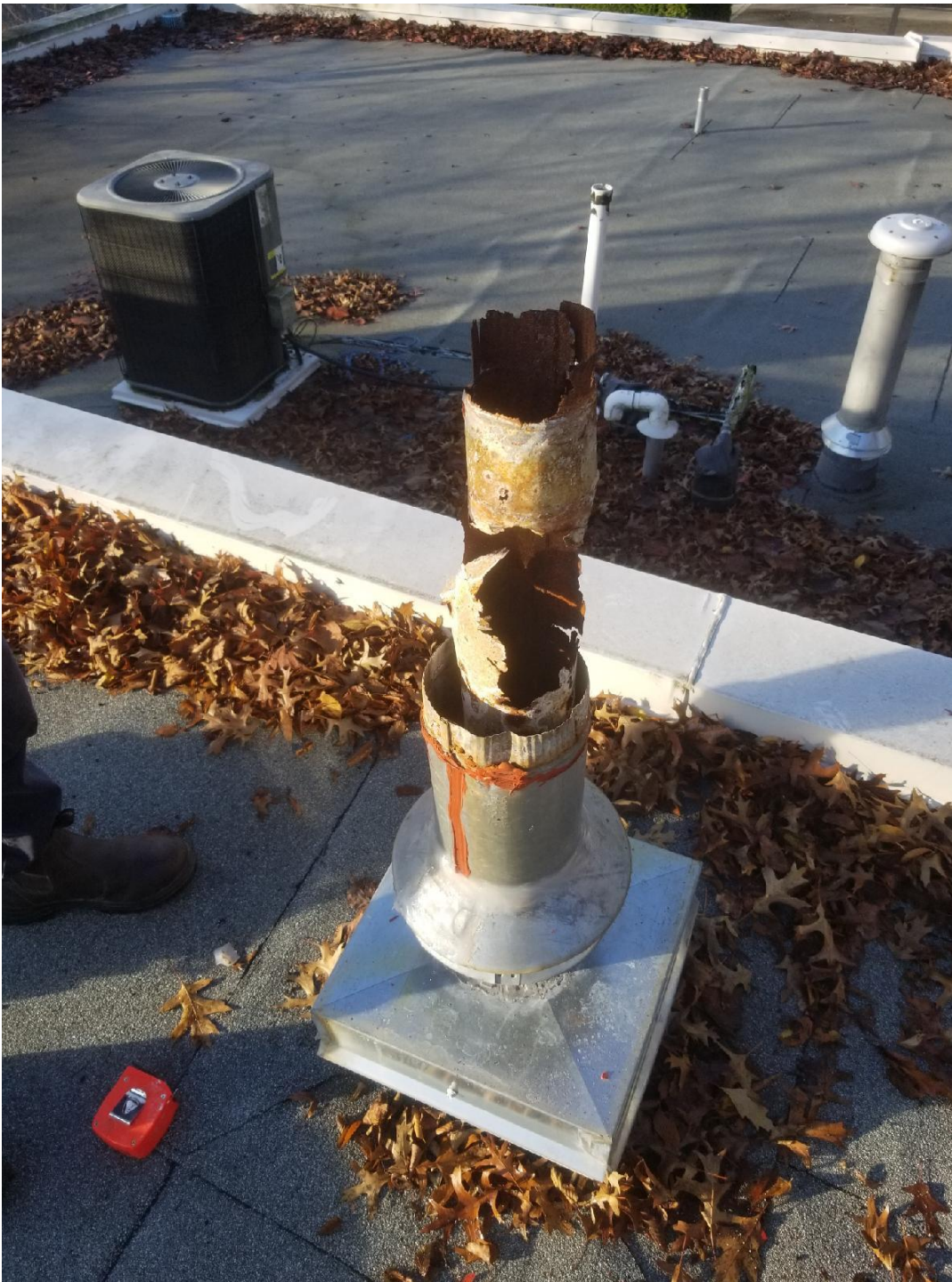
Figure 6. Picture of disassembled concentric termination showing corrosion damage
