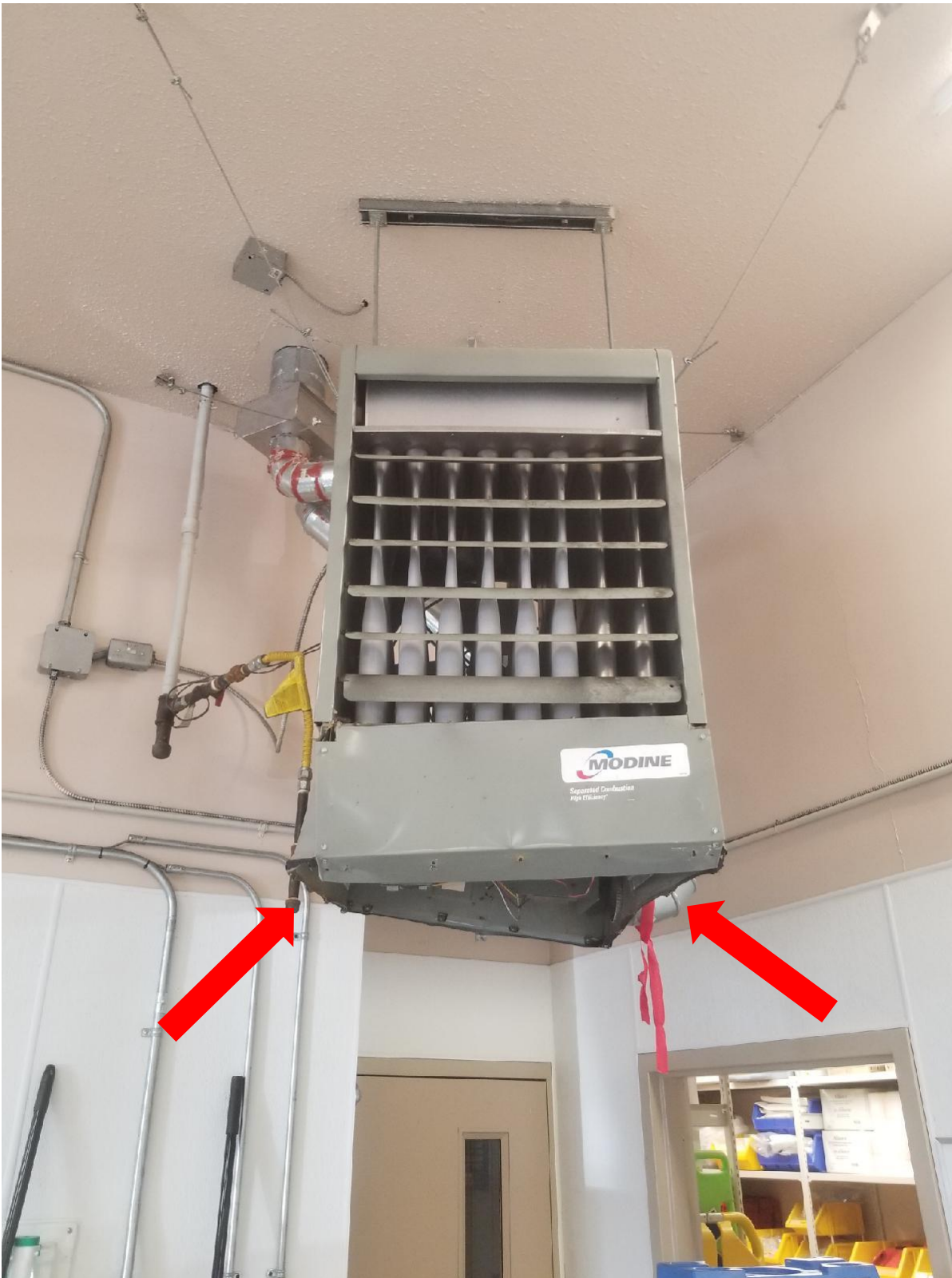
Figure 1. Picture of appliance showing damage
