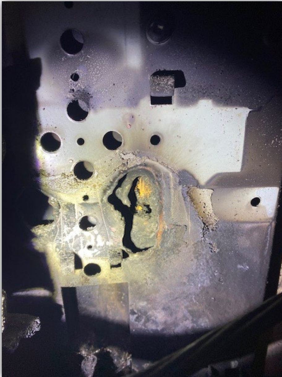
Image 3 - Close up image of electrical main combination panel metal enclosure located directly behind where main circuit breaker and metal bussing mechanically interconnect.
