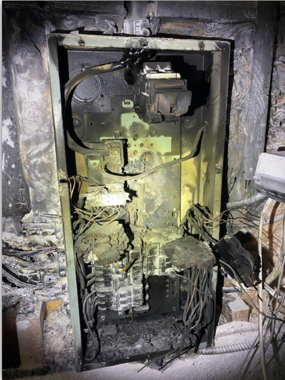
Image 2 - Close up image of Federal Pacific Electric (FPE) main combination panel.
