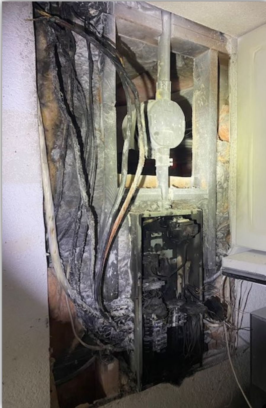
Image 1 – Main electrical panel within dwelling showing damage to panel and connected electrical equipment.
