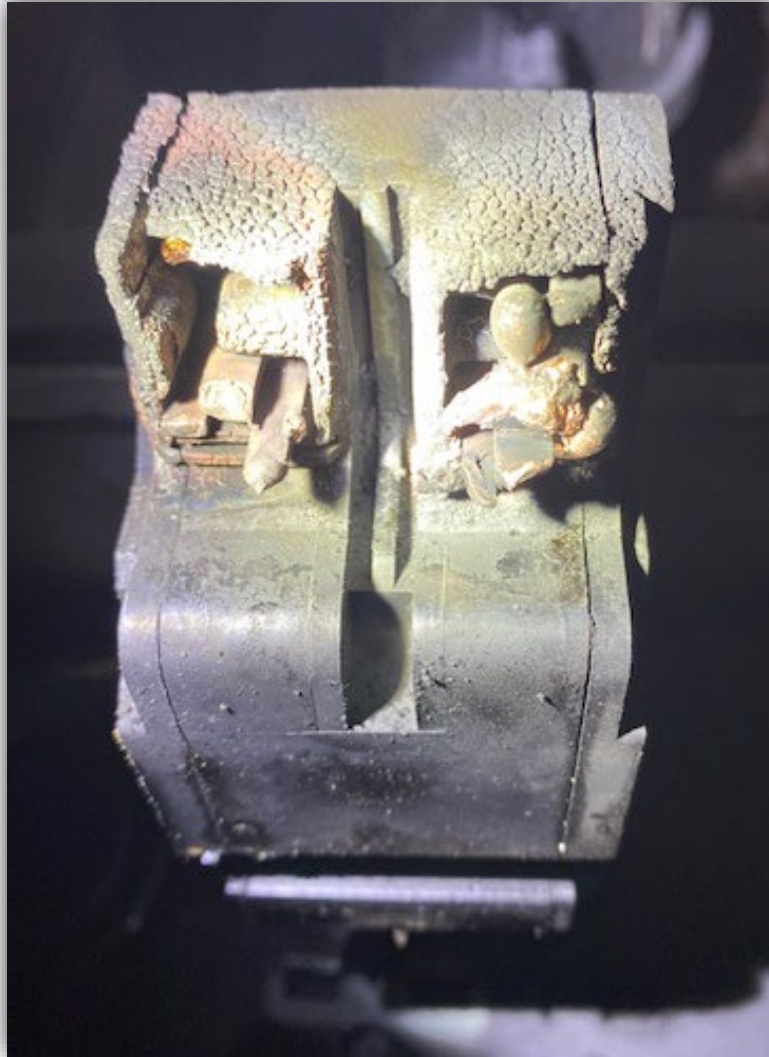
Image 4 - Close up image of load side of main circuit breaker showing tab design of connection and damage to the tabs. Condition of circuit breaker plastic enclosure also shown.
