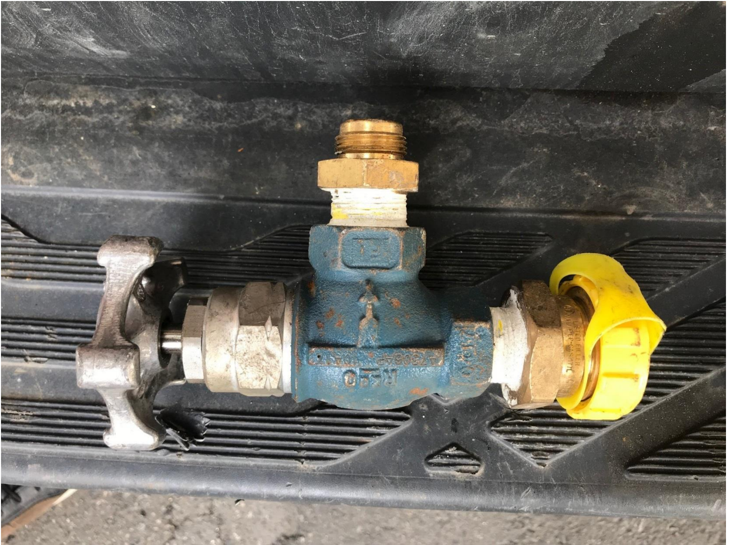
Photo #4: Evacuation valve adaptor and shut off valve. This is the shut off valve and adaptor used to connect to the evacuation valve on the existing tank that needs to have propane liquid removed.
