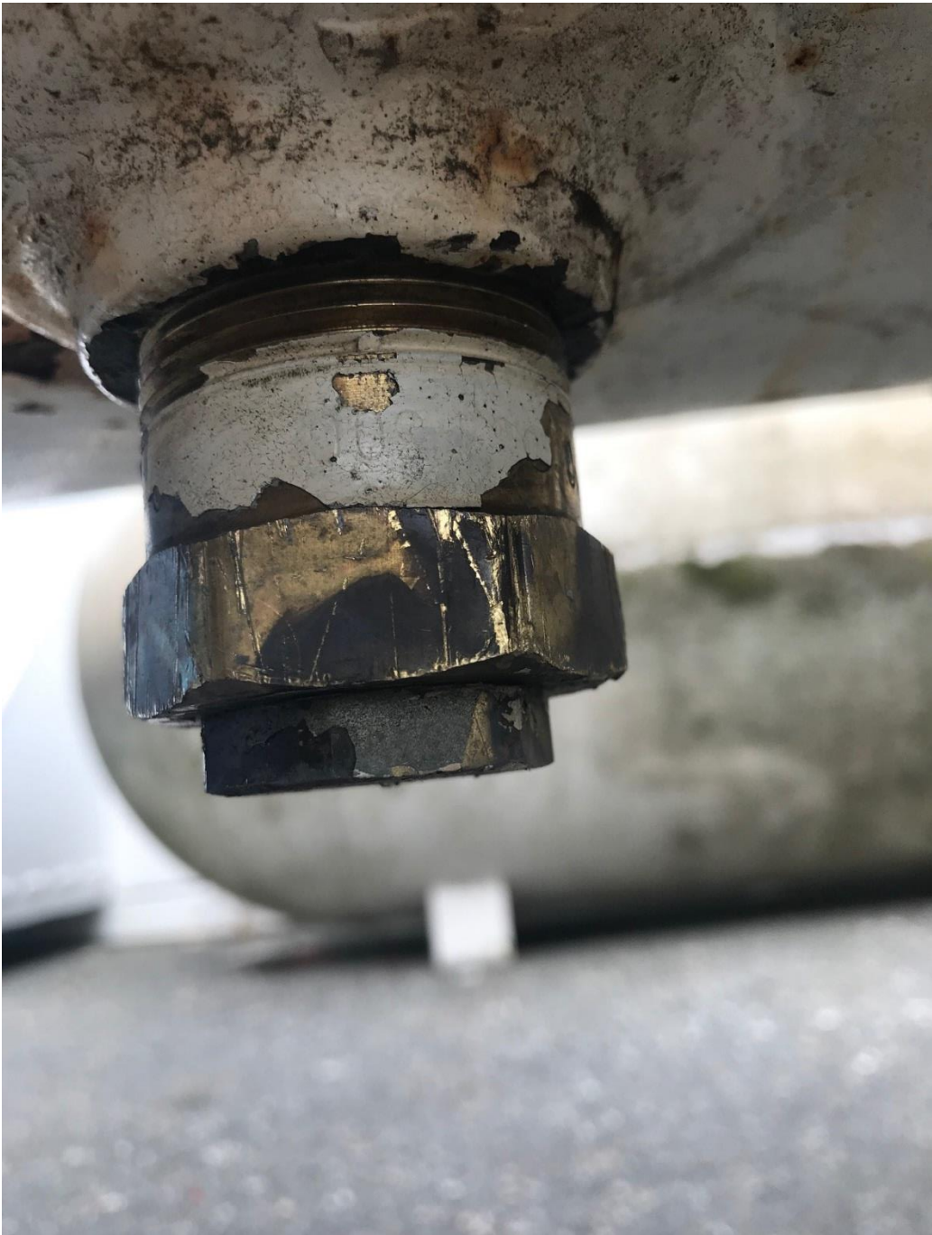
Photo #2: Evacuation valve on old propane tank.
