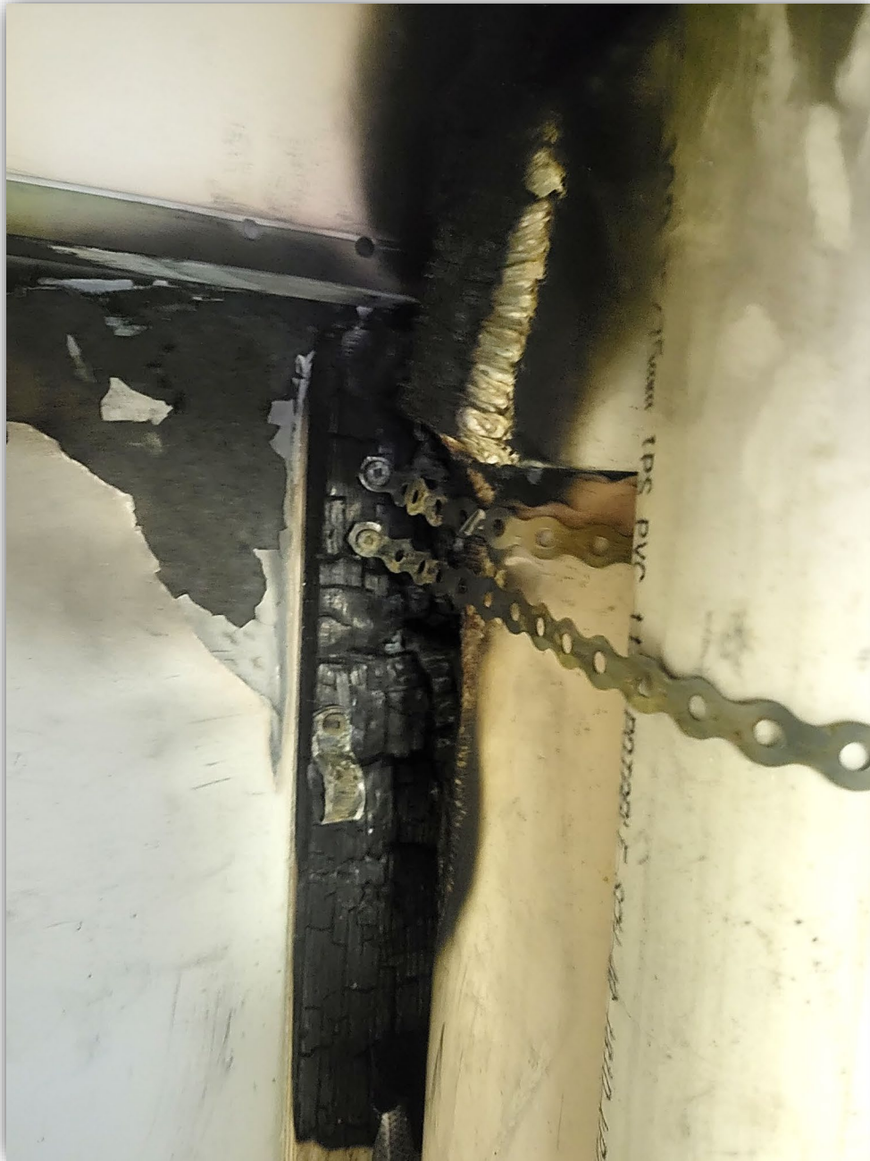
Photo 5 – Venting system fire damage.
