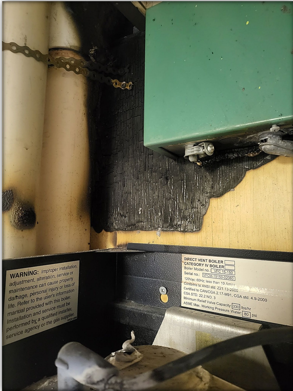
Photo 4 – Boiler nameplate and closeup of fire damage.
