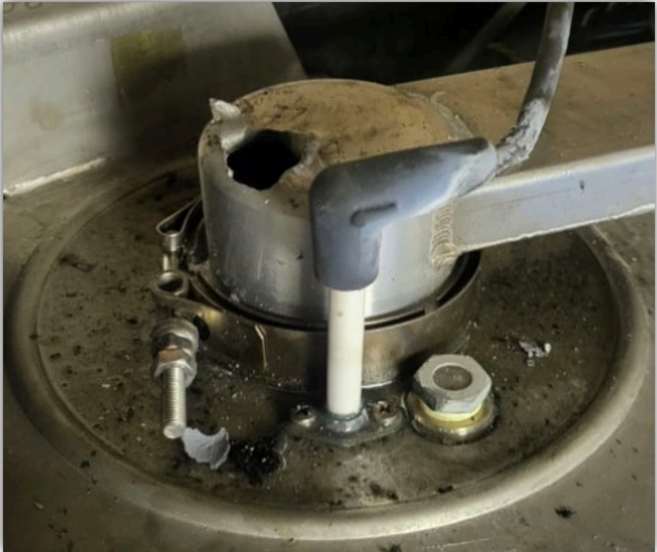
Photo 2 – Fan coupler with hole blown out of the top.
