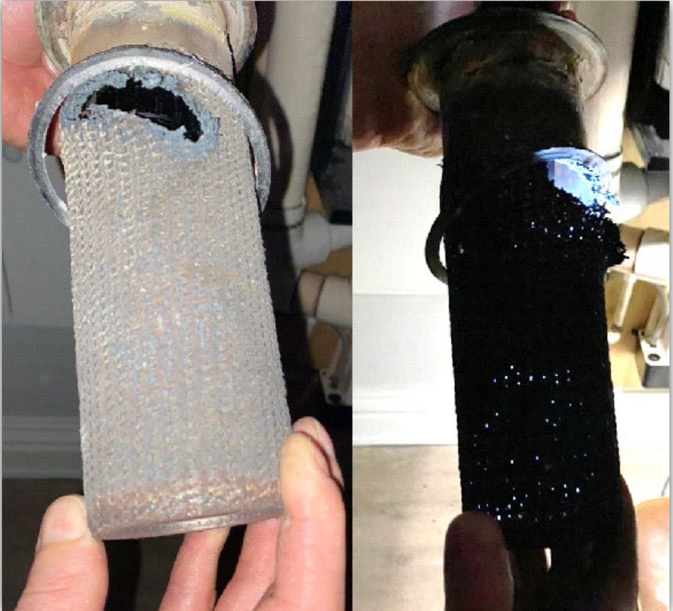
Photo 3a – Boiler burner mesh with hole.
