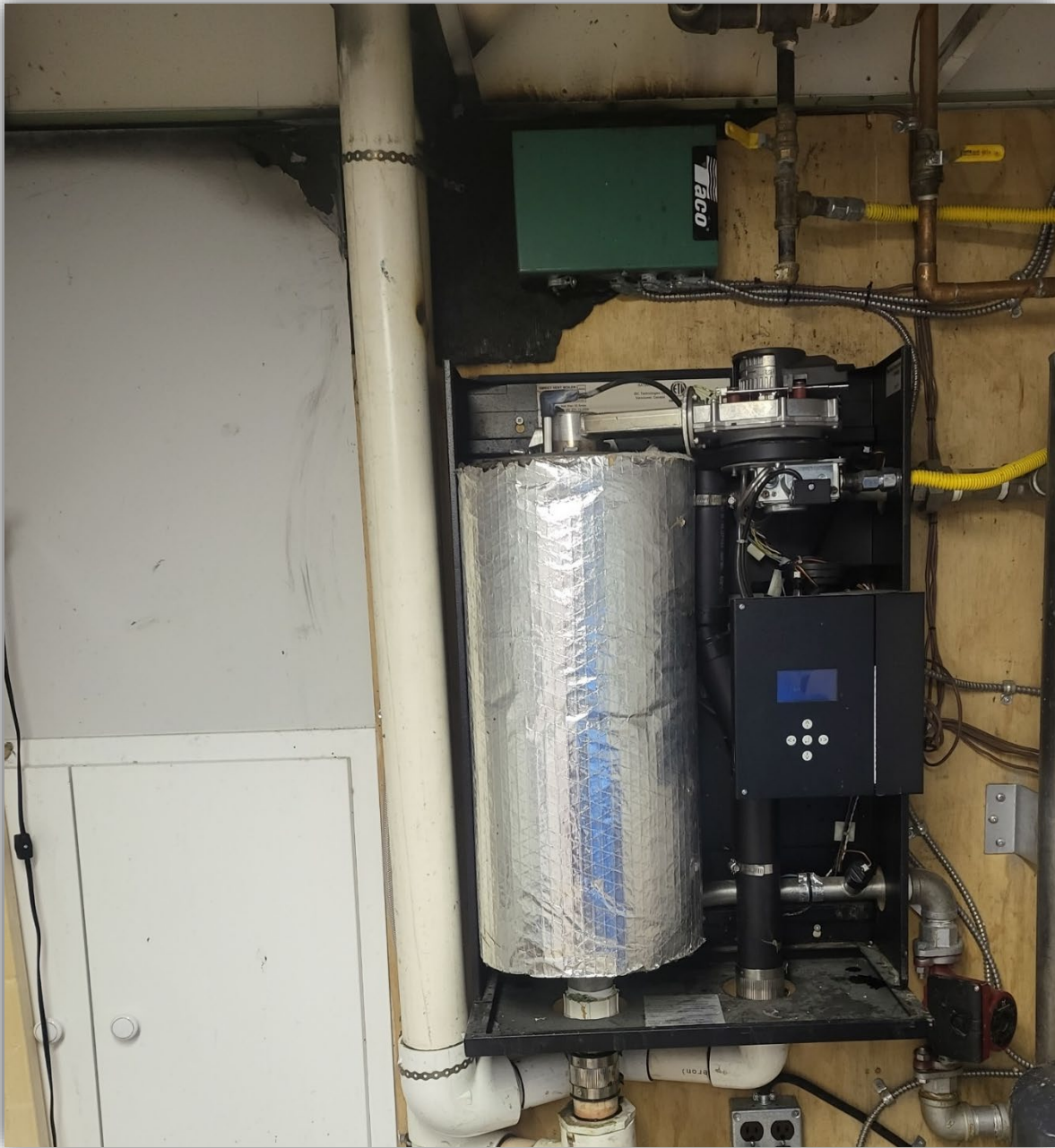
Photo 1 – Boiler with fire damage at top left corner.
