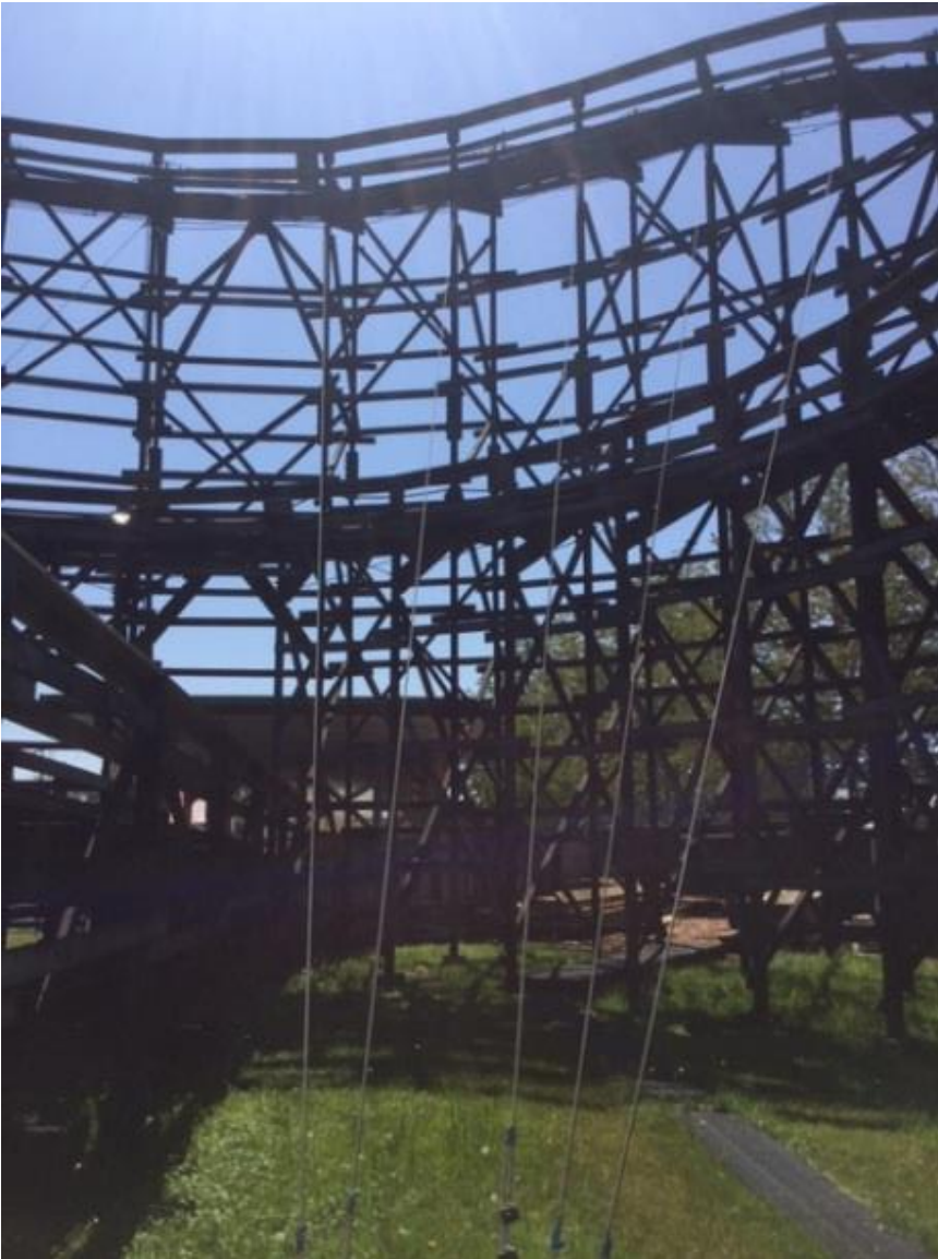
Photo 5: West guy lines connected to southern upper horseshoe.
